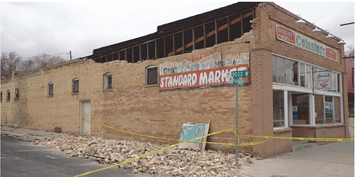
Figure 5-3 Damaged URM building in the 2020 M5.7 Magna Earthquake (from Utah Geological Survey).
