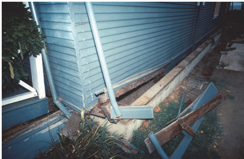
Figure 4-6 House that fell off its foundation in the 1989 Loma Prieta Earthquake.
