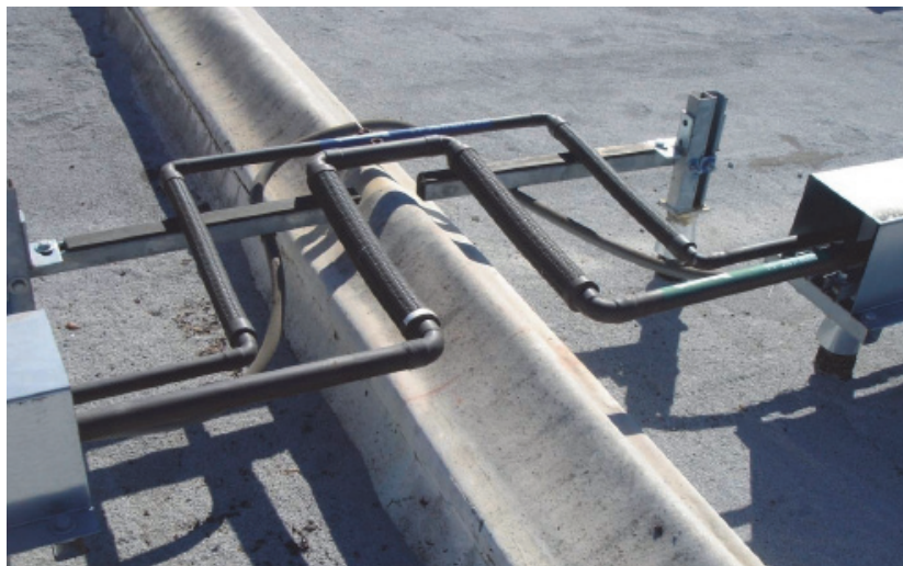
Figure 9-3 Pipe crossing seismic joint between two buildings (from M. Phipps). The loops in the pipe have been designed to provide flexibility to accommodate movement across the joint.
