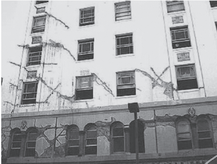
Figure 5-6 Diagonal cracking in a reinforced concrete building damaged by the 1989 Loma Prieta Earthquake (from FEMA P-154).
