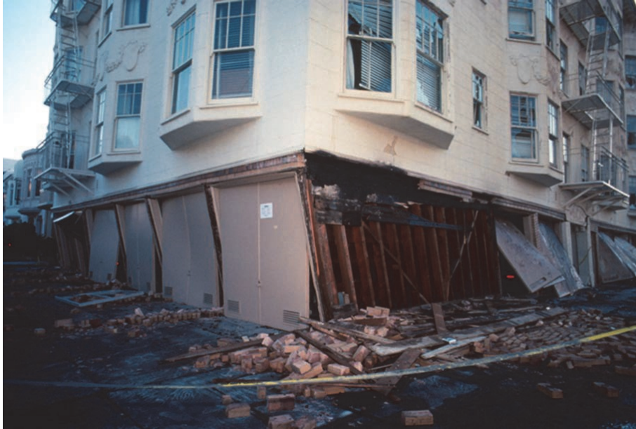
Figure 4-8 First story of an apartment building in San Francisco leaning to the side after the 1989 Loma Prieta Earthquake.
