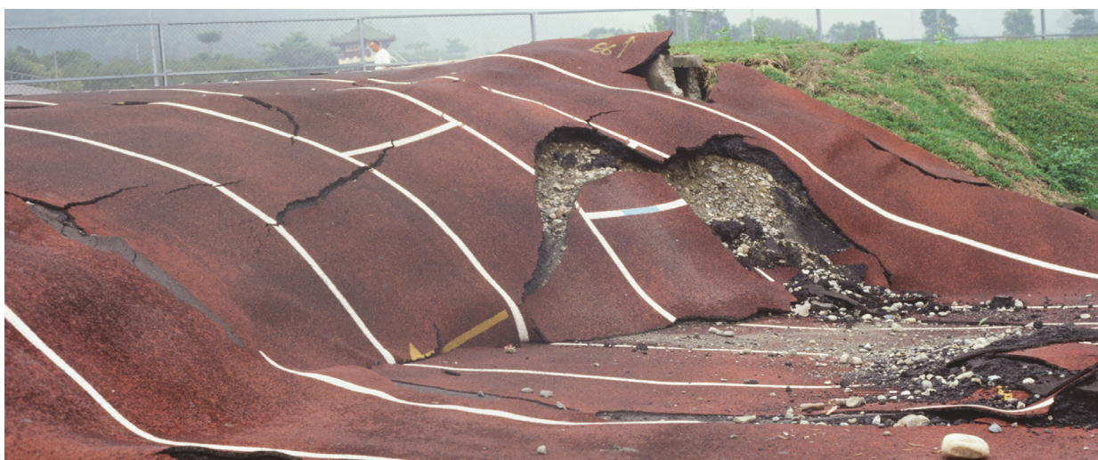
Figure 1-15 Vertical fault offset of a school track from surface fault rupture in the 1999 M7.7 Chi-Chi Earthquake in Taiwan (from B. Yeats).
