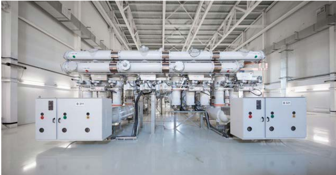
Figure 4.3.11. Indoor gas-insulated switchgears can be used in environments where water can penetrate the control house. (Source: Siemens Energy, 2021)
