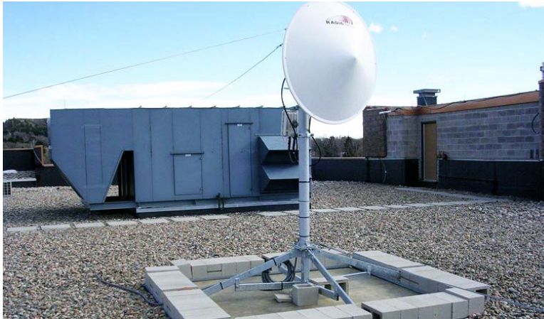
Figure 4.4.2. Rooftop antennas often are mounted using ballast sleds.
