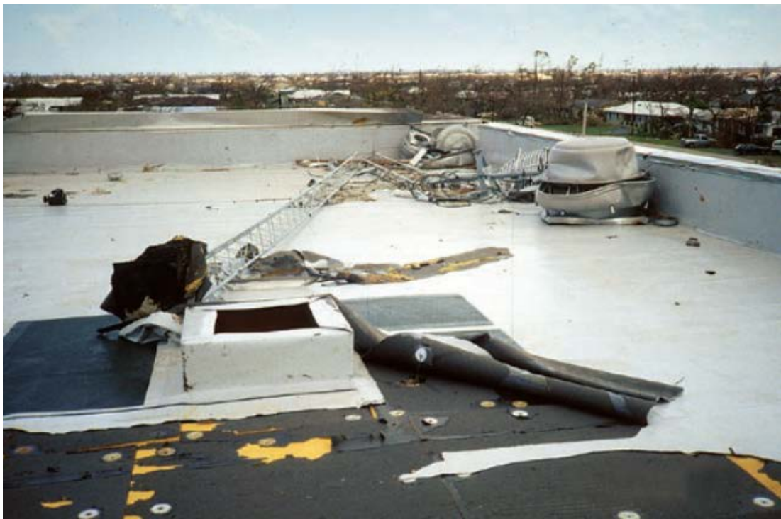
Figure 4.4.1. The collapse of a tower with antennas can damage the roof membrane, causing it to peel.
