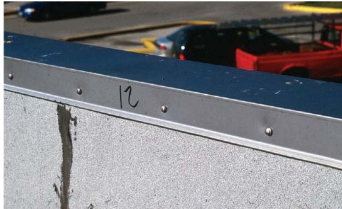
Figure 3.3.2.3. Both vertical faces of coping were attached with exposed fasteners (1/4-inch diameter stainless steel fasteners spaced 12" on center) instead of concealed cleats following Typhoon Paka (1997) in Guam to prevent the flashing from tearing in future storms.
