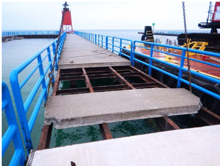
Figure 5.5.3. Improve pier performance during future storms by replacing storm-damaged pre-cast concrete pier deck panels with reinforced cast-in-place concrete (Source: U.S. Army Corps of Engineers, No Date).
