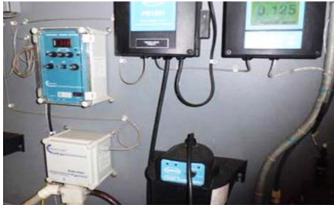
Figure 4.1.6. Elevating instrumentation can protect it from flood damage. (Source: U.S. Environmental Protection Agency [EPA], 2014)
