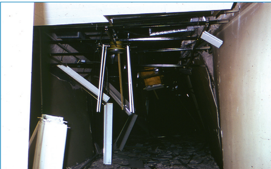
Figure 2-23: A damaged exit corridor—dark and barely passable
