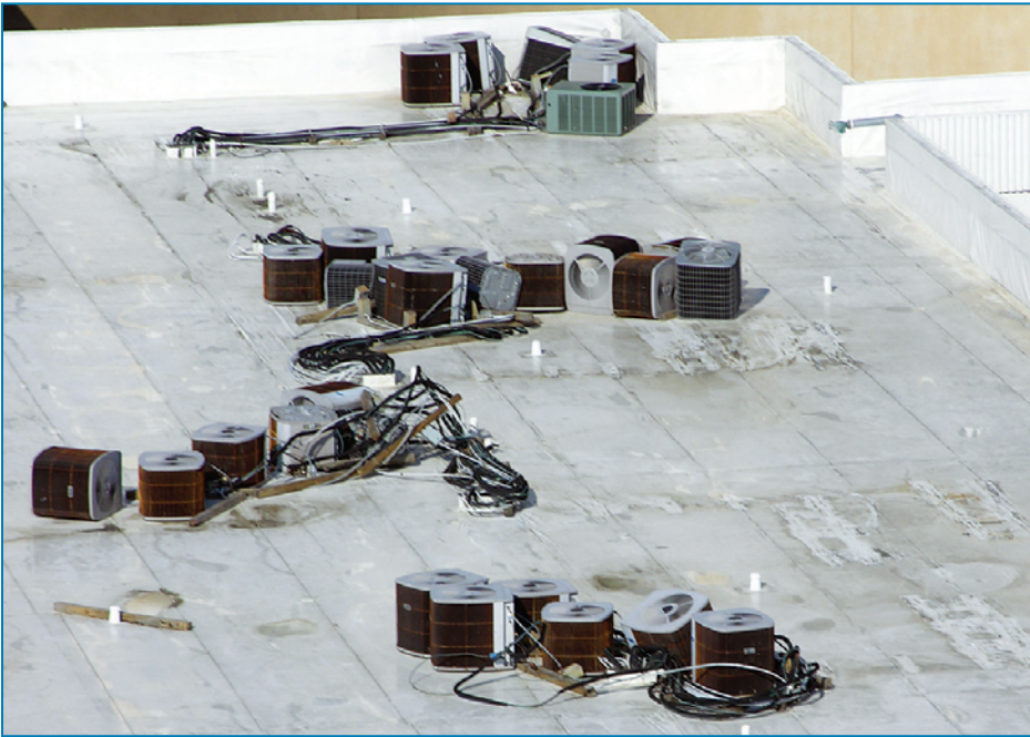
Figure 4-90: Sleeper-mounted condensers displaced by high winds. Hurricane Katrina (Mississippi, 2005)
