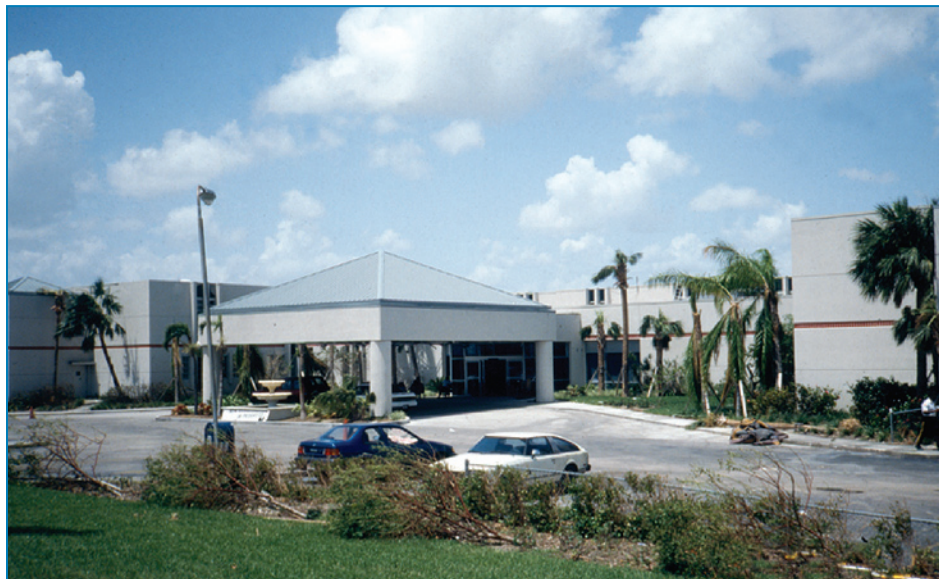
Figure 4-1: Deering Hospital was evacuated after Hurricane Andrew due to water infiltration caused by roof covering, window, and door damage.
