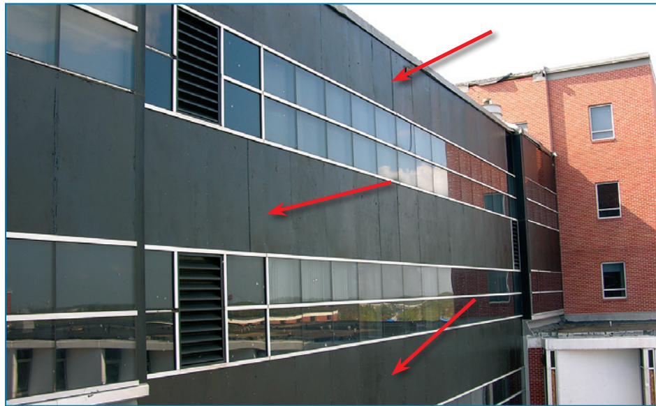
Figure 4-46: Plywood panels (black continuous bands) installed after the glass spandrel panels were broken by roof aggregate. 9 Hurricane Katrina (Mississippi, 2005)
