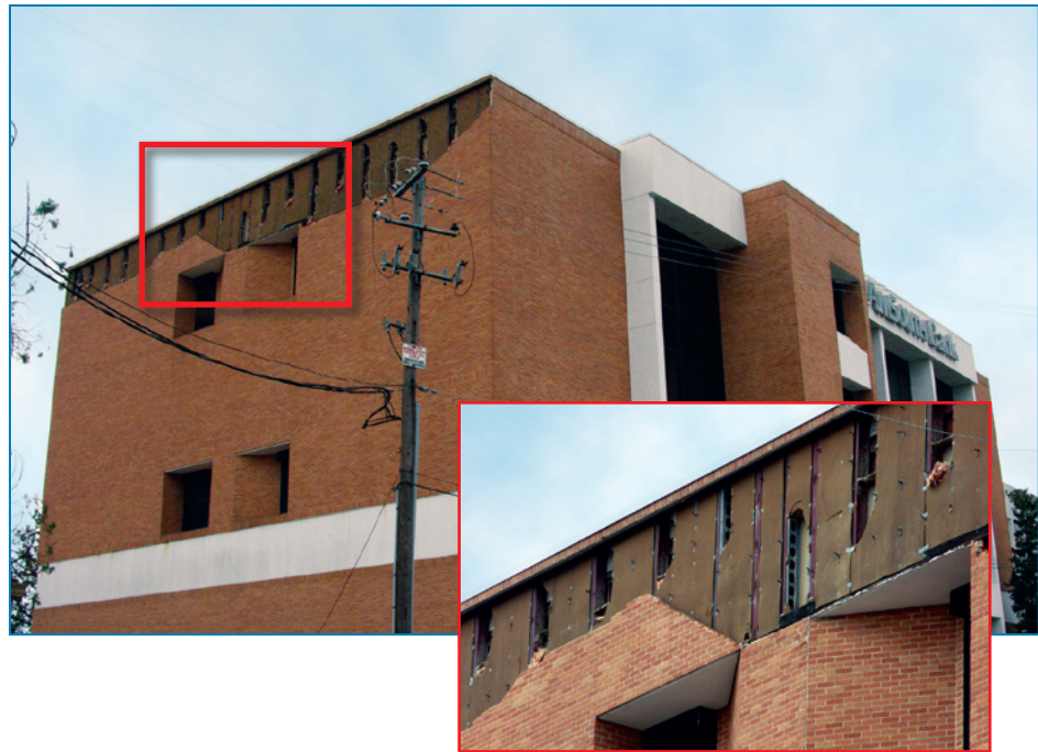
Figure 4-52: The brick veneer failure on this building was attributed to tie corrosion. Hurricane Ivan (Florida, 2004)
