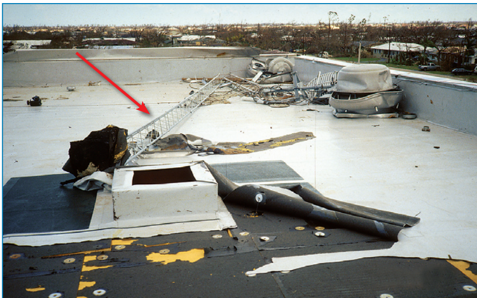
Figure 4-95: The collapse of the antenna tower caused progressive peeling of the roof membrane. Also note that the exhaust fan blew off the curb, but the high parapet kept it from blowing off the roof. Hurricane Andrew (Florida, 1992)
