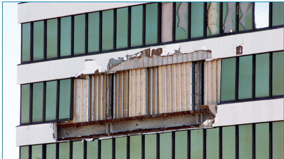
Figure 4-17: Broken windows in the MOB. Wood studs and gypsum board had been temporarily installed after the hurricane to prevent patients from inadvertently falling out of the MOB.
