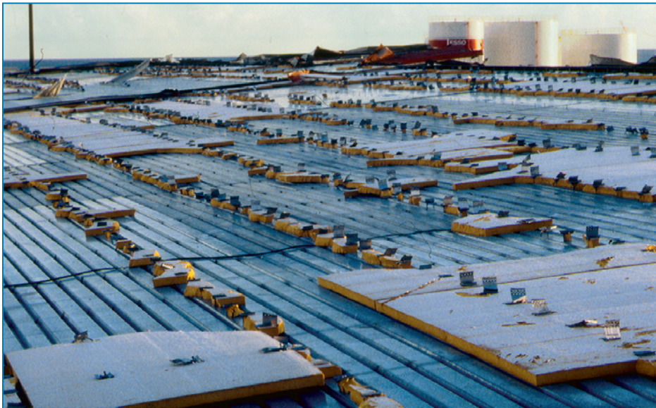
Figure 4-73: Significant interior water damage and facility interruption occurred after the standing seam roof blew off. Hurricane Marilyn (U.S. Virgin Islands, 1995)
