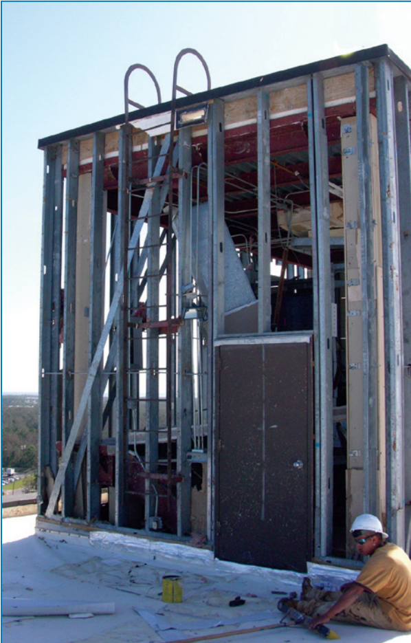
Figure 4-22: The only remaining portion of the exterior wall surrounding the elevator penthouse on the MOB was the steel studs.
