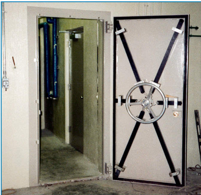
Figure 3-36: Permanent watertight doors designed for deep water
