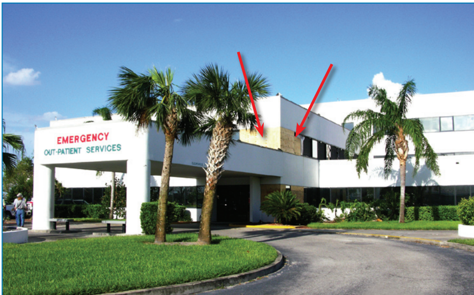
Figure 4-80: The second floor beyond the canopy houses the ICU. Several windows along the two ICU walls that are visible were broken.
