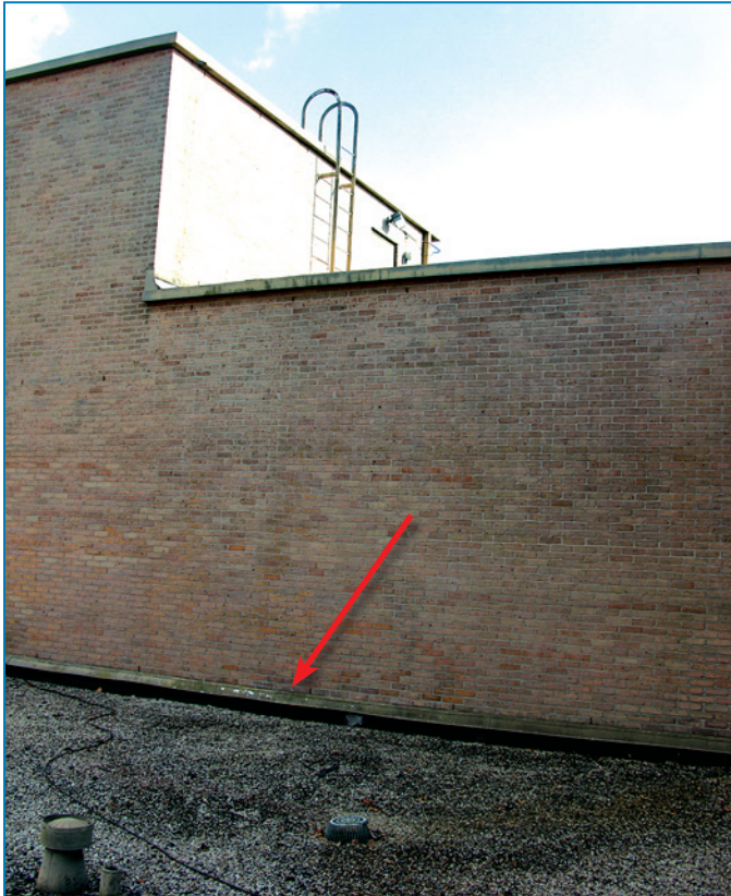
Figure 4-58: Water leaked inside along the base of the brick veneer walls (red arrow). Hurricane Katrina (Louisiana, 2005)
