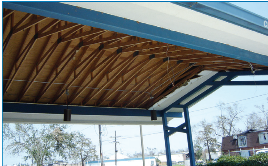
Figure 4-50: Hospital canopy damage. Hurricane Katrina (Louisiana, 2005)
