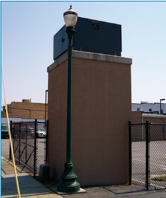
Figure 3-48: Elevated utility box
