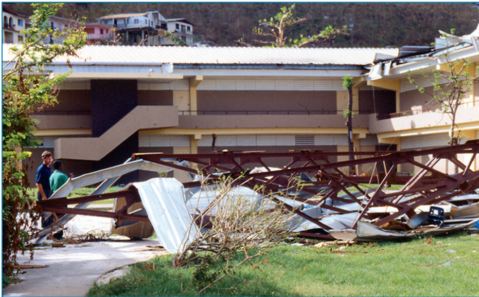
Figure 4-113: The steel truss superstructure installed as part of a steep-slope conversion blew away because of inadequate attachment. Hurricane Marilyn (U.S. Virgin Islands, 1995)
