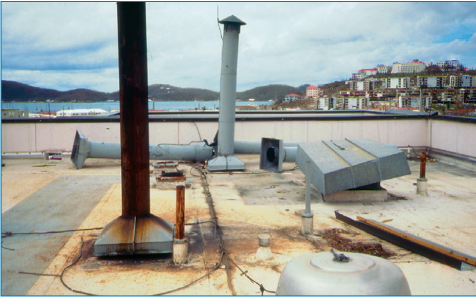
Figure 4-93: Three of the five stacks that did not have guy-wires were blown down. Hurricane Marilyn (U.S. Virgin Islands, 1995)
