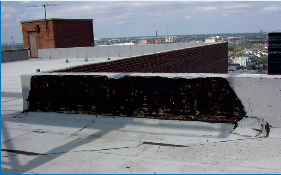
Figure 4-120: Failed base flashing adhered directly to the brick parapet. Hurricane Katrina (Louisiana, 2005)
