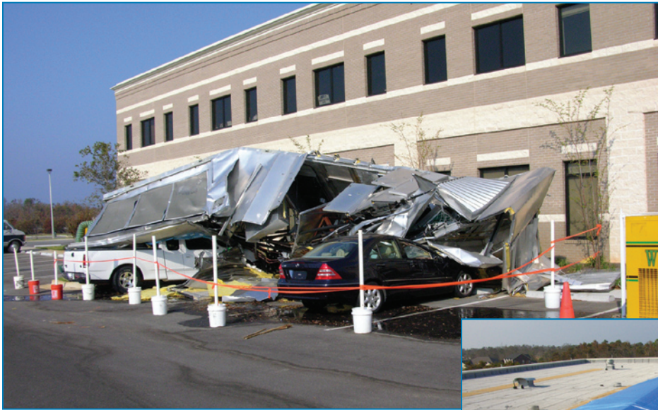
Figure 4-86: Although this 18,000-pound HVAC unit was attached to its curb with 16 straps, it blew off during Hurricane Ivan. (Florida, 2004)
