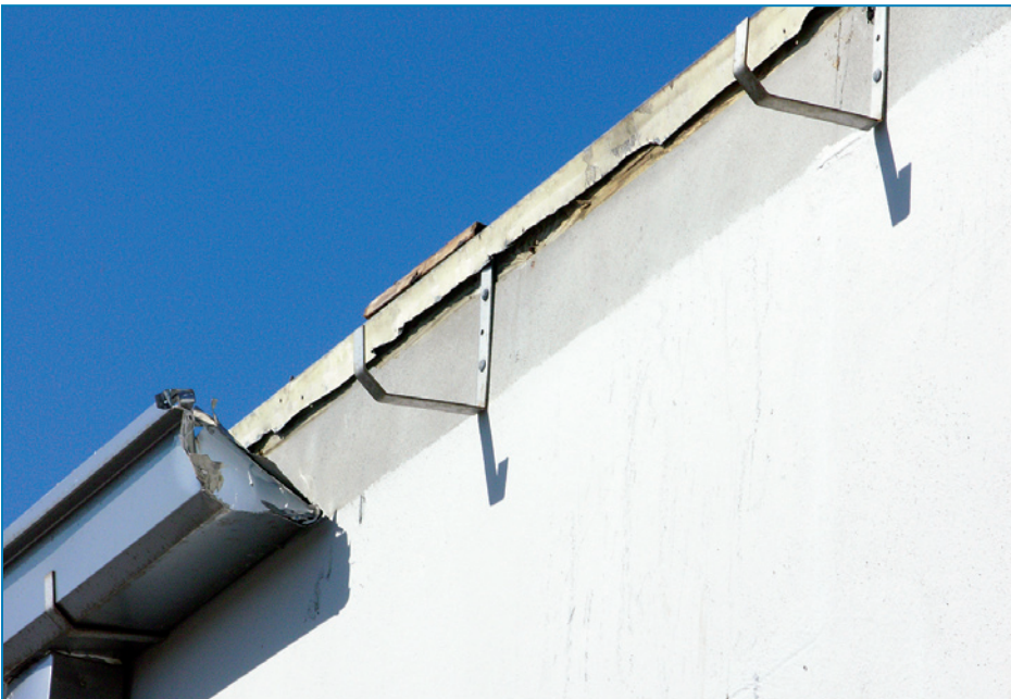
Figure 4-68: This gutter, supported by a type of bracket that provides no significant uplift resistance, failed when wind lifted it, together with the metal edge flashing that lapped into the gutter. Hurricane Francis (Florida, 2004)
