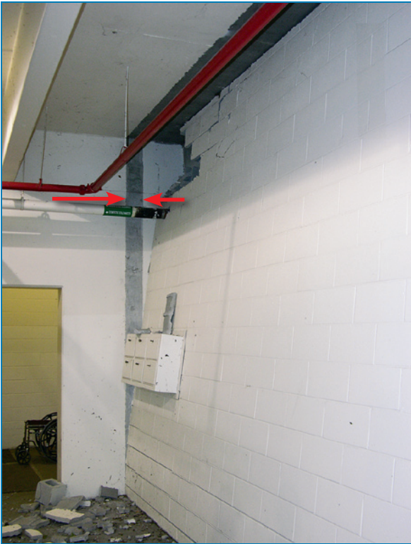
Figure 4-51: The red arrows show the original location of a CMU wall that nearly collapsed following a rolling door failure. Hurricane Charley (Florida, 2004)
