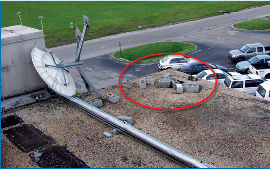
Figure 4-83: This satellite dish was held down only with CMU. Note the displaced LPS at the corner (circled).
