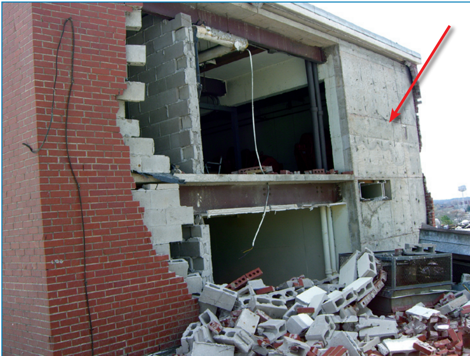
Figure 4-148: Collapsed brick veneer/CMU wall at a mechanical room. The cast-in-place concrete wall (arrow) remained, but the brick veneer was blown away.
