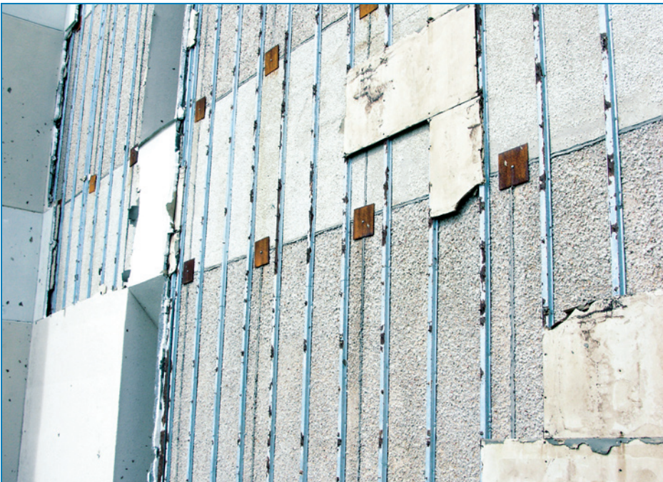
Figure 4-23: Close-up of the damaged EIFS at the hospital. In this area most of the insulation and gypsum board was blown from the steel furring channels.
