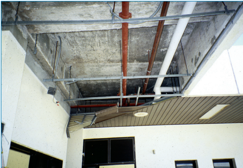
Figure 4-49: This suspended metal soffit was not designed for upward-acting wind pressure. Typhoon Paka (Guam, 1997)
