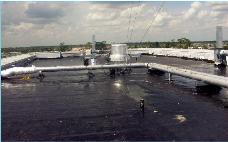
Figure 4-110: The roof membrane and some of the rooftop equipment blew off. Although the deck was cast-in-place concrete, water leaked into the patient floor below. Hurricane Charley (Florida, 2004)
