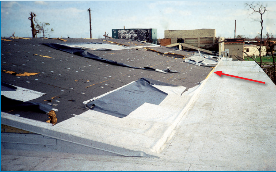
Figure 4-75: Mechanically attached single-ply membrane progressively tore after being cut by wind-borne debris. Hurricane Andrew (Florida, 1992)
