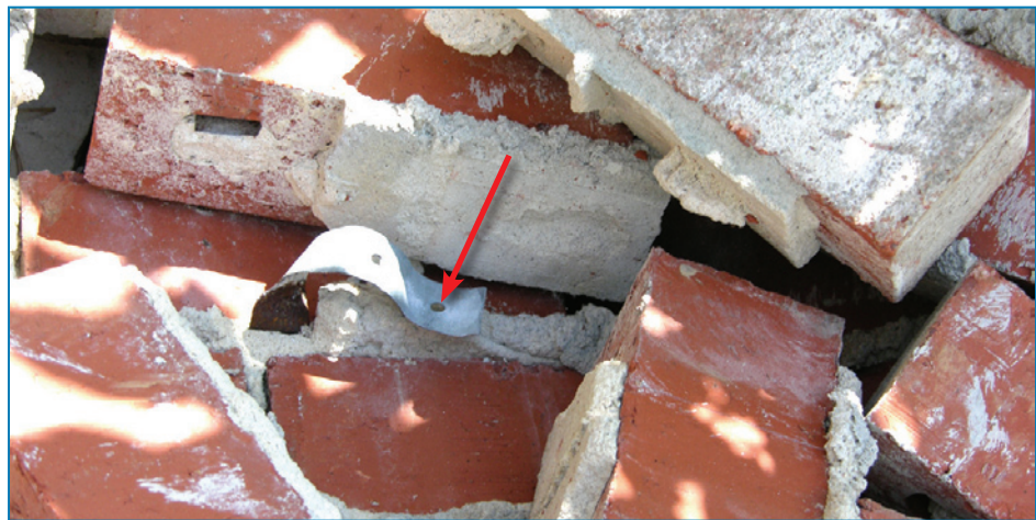
Figure 4-53: This tie remained embedded in the mortar joint while the smooth-shank nail pulled from the stud.
