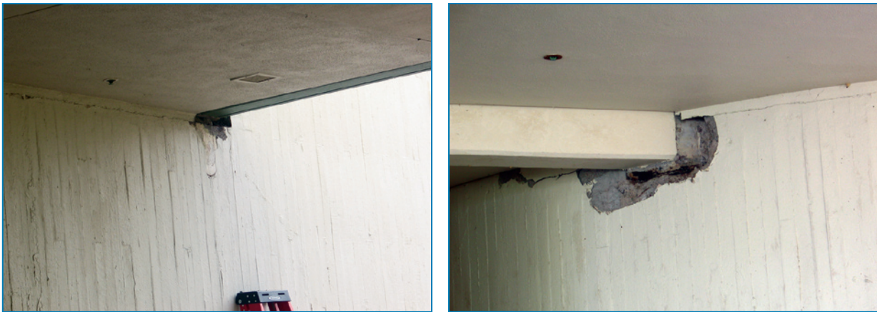
Figure 2-40: Spalling at beam connections
