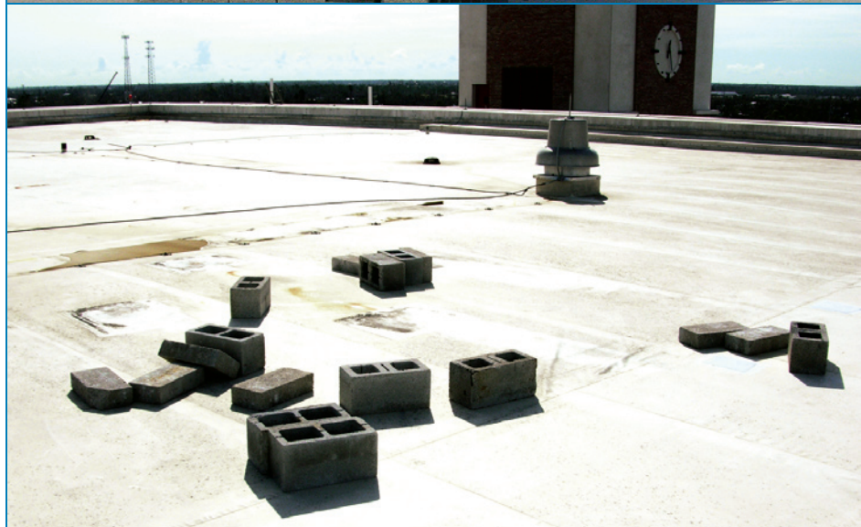
Figure 4-97: A satellite dish anchored similarly to that shown in Figure 4-96 was blown off this five-story building. Hurricane Charley (Florida, 2004)
