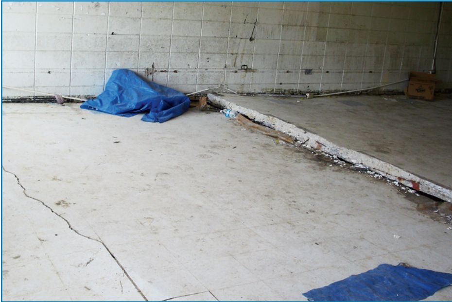
Figure 3-15: Concrete slab ruptured by hydrostatic pressure (buoyancy) induced by the floodwaters of Hurricane Katrina (2005).
