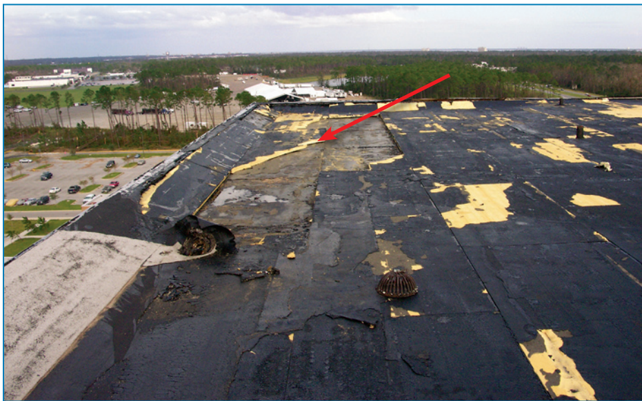
Figure 4-71: The blown off insulation (red arrow) may have initiated blow off of the roof membrane. Hurricane Ivan (Florida, 2004)
