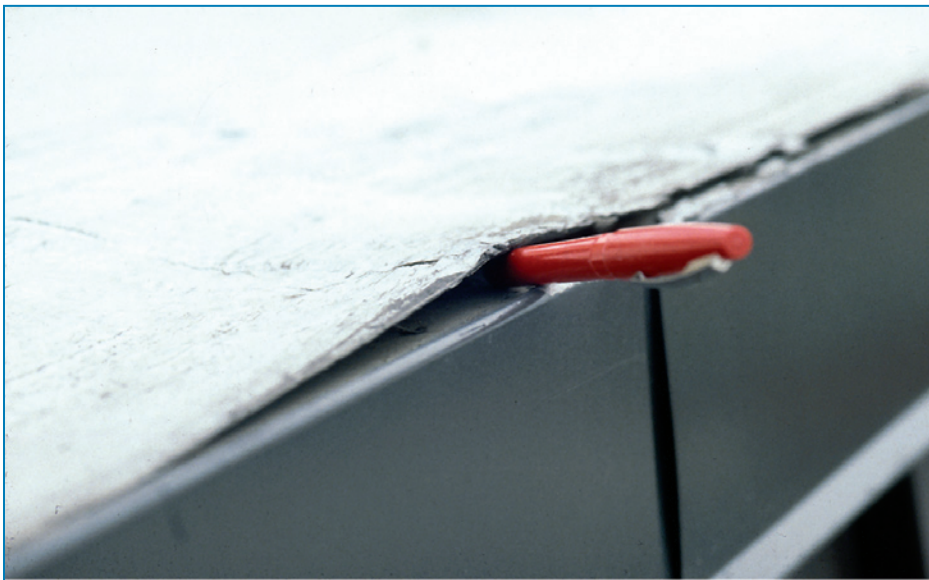
Figure 4-65: The ink pen shows an opening that the wind can catch, and cause lifting and peeling of the membrane.
