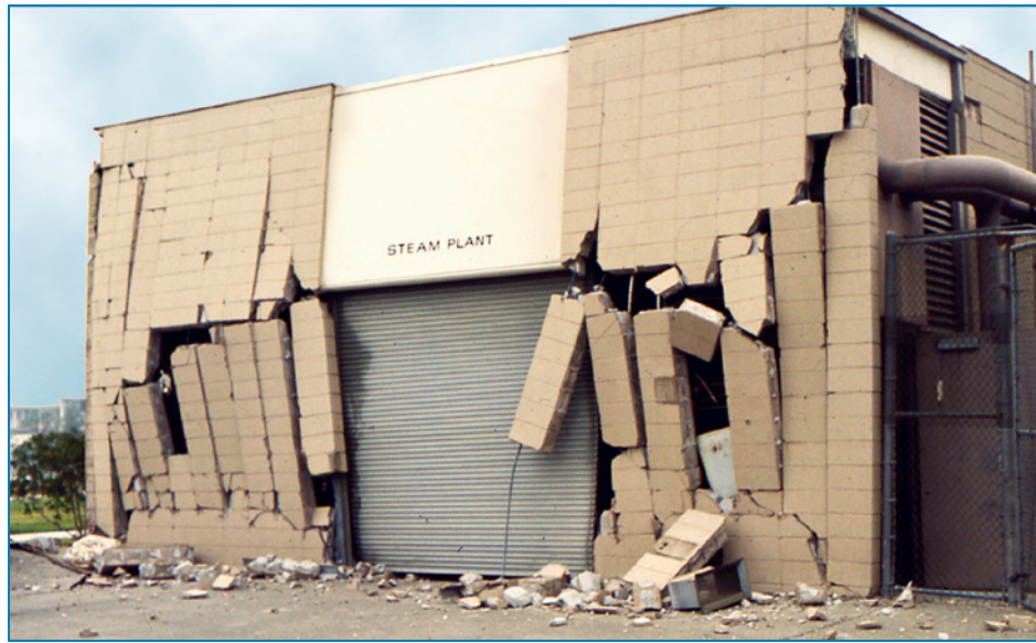
Figure 2-18: Severe damage to a poorly reinforced masonry wall on a steam plant
