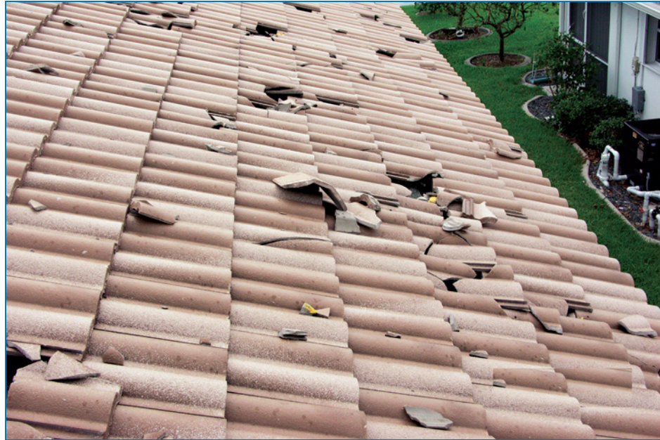
Figure 4-74: Brittle roof coverings, like slate and tile, can be broken by missiles, and tile debris can break other tiles. Hurricane Charley (Florida, 2004)
