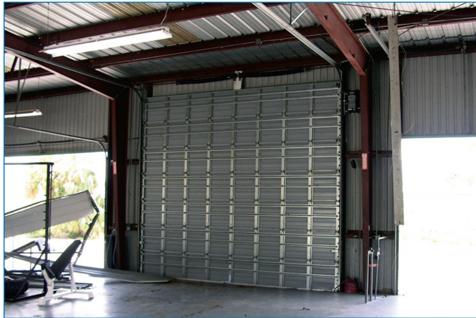
Figure 4-114: The new door in the center performed very well, but the older doors on either side of it were blown away. Hurricane Charley (Florida, 2004)
