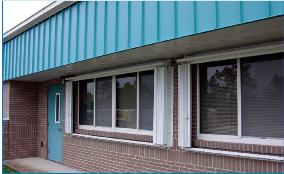
Figure 4-116: This building has accordion shutters. Hurricane Ivan (Florida, 2004)
