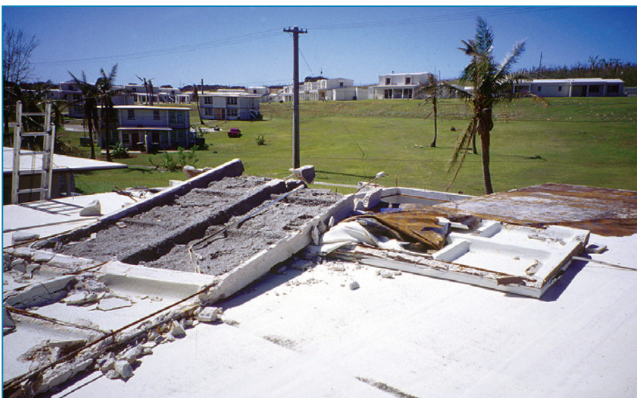
Figure 4-31: Portions of this waffled precast concrete roof deck were blown off. Typhoon Paka (Guam, 1997)
