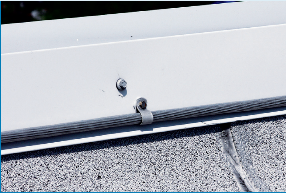
Figure 4-101: This conductor was attached to the coping with a looped connector. Hurricane Katrina (Mississippi, 2005)
