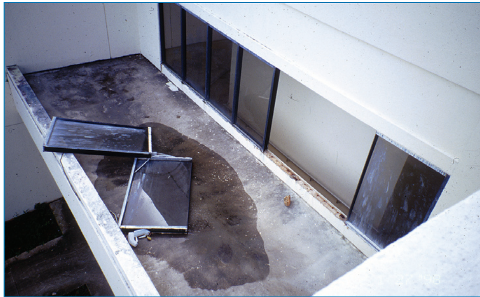
Figure 4-43: Two complete windows, including frames, blew out as a result of an inadequate number of fasteners. Typhoon Paka (Guam, 1997)
