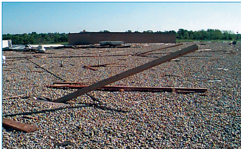
Figure 4-128: A violent tornado showered the roof with missiles. (Oklahoma, 1999)
