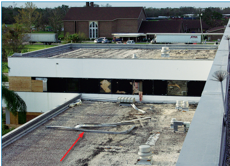
Figure 4-81: A view of the ICU from the third floor roof. The gutters (red arrow) are from the back side of the third floor roof.
