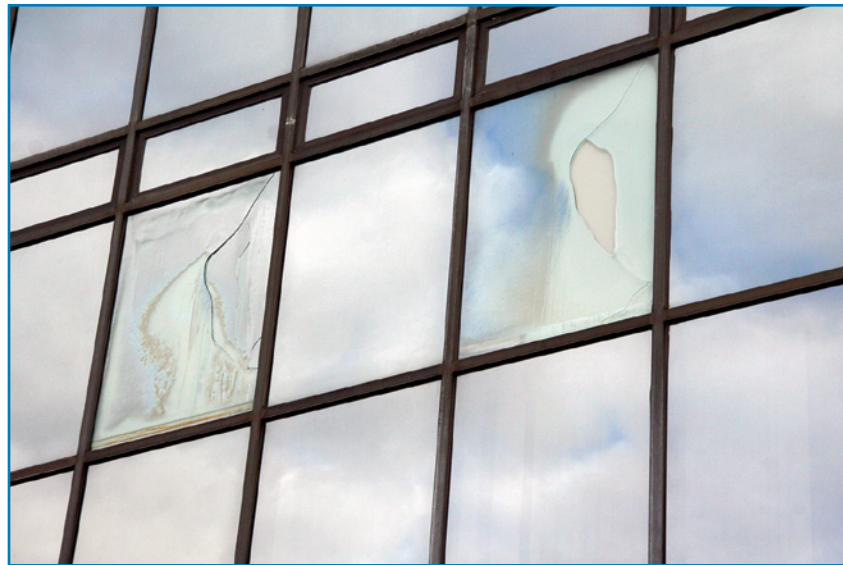
Figure 4-9: Broken windows at Touro Infirmary
