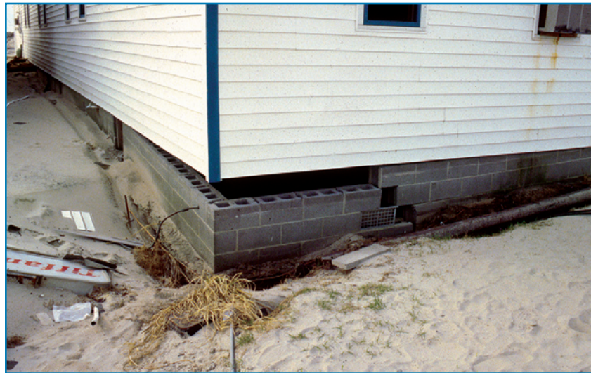
Figure 2-11: Local scour undermined this shallow foundation (also note that the building was not anchored to the foundation).
