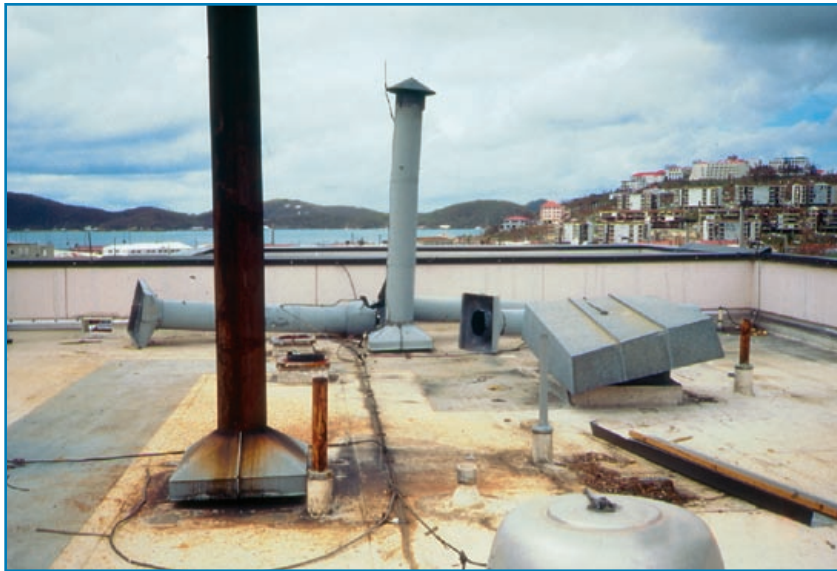
Figure 3-76: Three of the five stacks that did not have guy-wires were blown down. Hurricane Marilyn (U.S. Virgin Islands, 1995)
