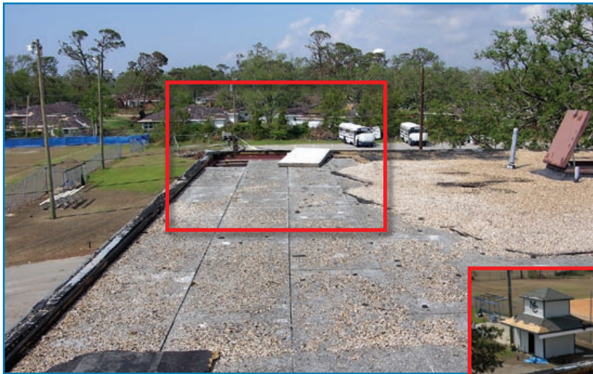
Figure 3-106: The school's built-up roof blew off after one of the cementitious wood-fiber deck panels detached from the joists. Hurricane Katrina (Mississippi, 2005)
