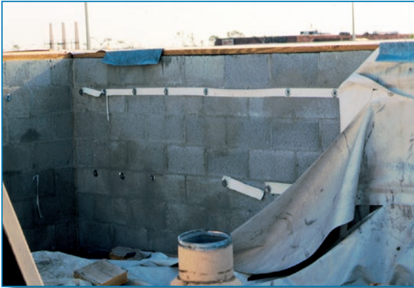
Figure 3-66: If mechanically attached base flashings have an insufficient number of fasteners, the base flashing can be blown away. Hurricane Andrew (Florida, 1992)
