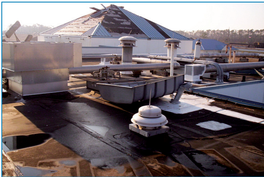
Figure 4-8: Roof damage on Hancock Medical Center
