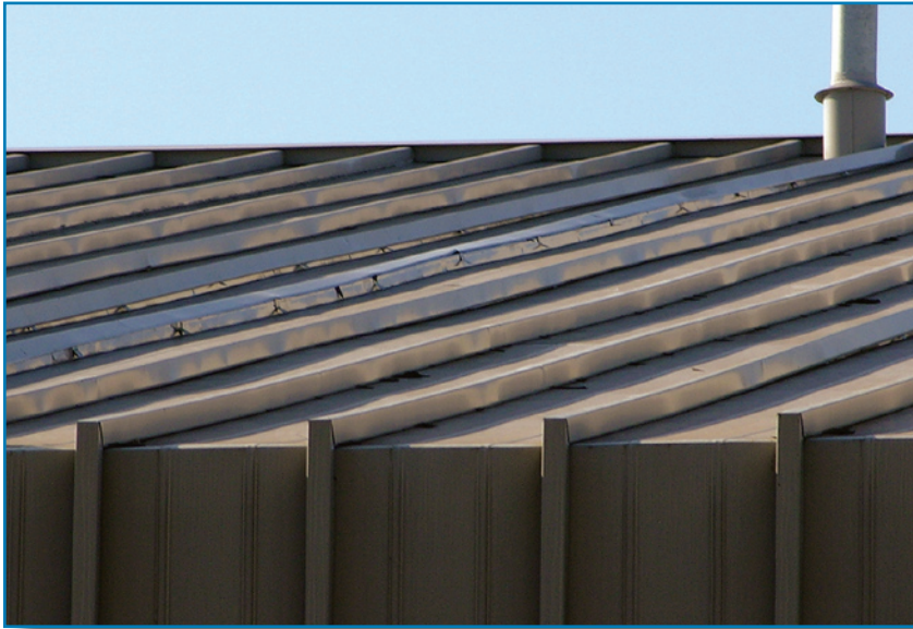
Figure 4-43: Lifted batten covers on Third District Fire Station metal roof
