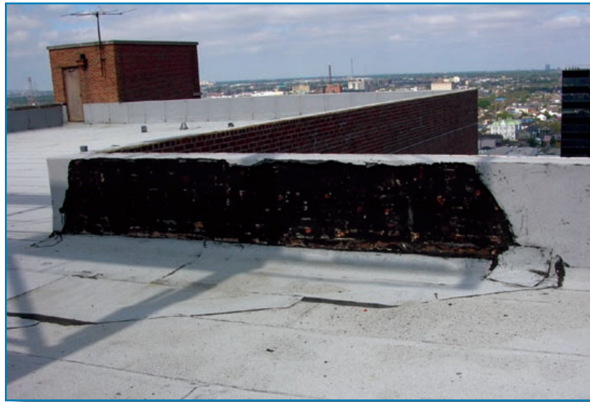
Figure 3-117: Failed base flashing adhered directly to the brick parapet. Hurricane Katrina (Louisiana, 2005)
