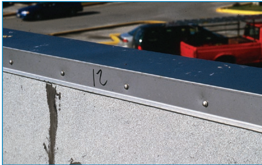
Figure 3-63: Both vertical faces of the coping were attached with exposed fasteners instead of concealed cleats. Typhoon Paka (Guam, 1997)
