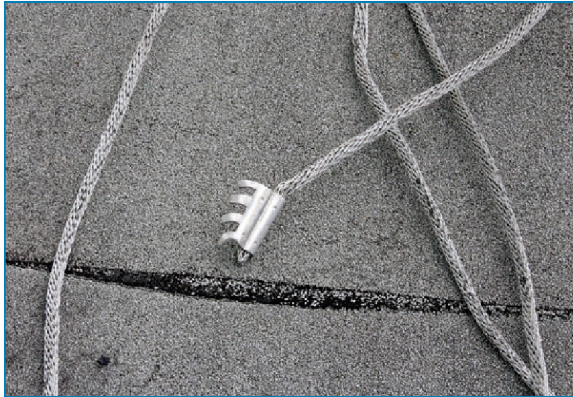
Figure 3-100: If conductors detach from the roof, they are likely to pull out from pronged splice connectors. Hurricane Charley (Florida, 2004)
