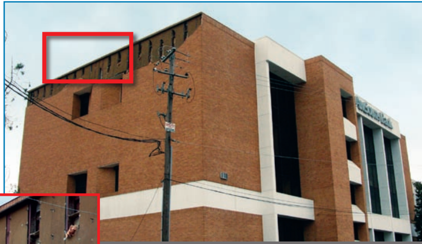
Figure 3-45: The brick veneer failure on this building was attributed to tie corrosion. Hurricane Ivan (Florida, 2004)
