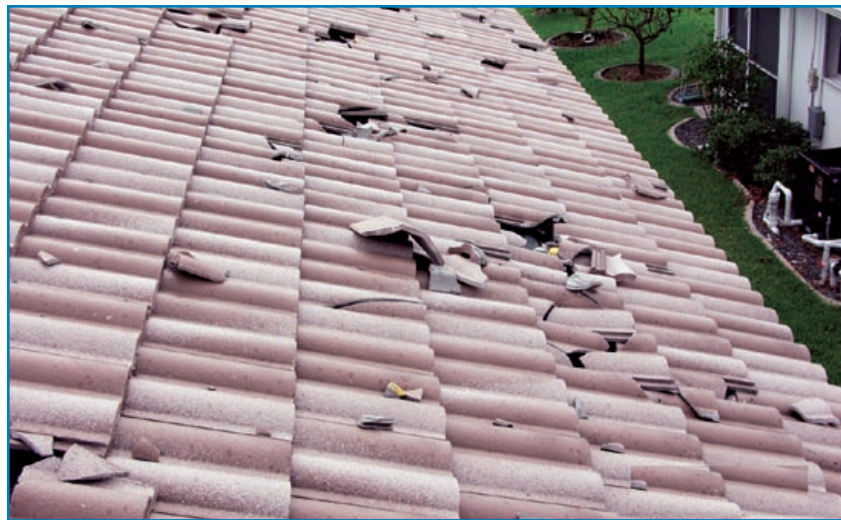
Figure 3-88: Brittle roof coverings, like slate and tile, can be broken by missiles, and tile debris can break other tiles. Hurricane Charley (Florida, 2004)
