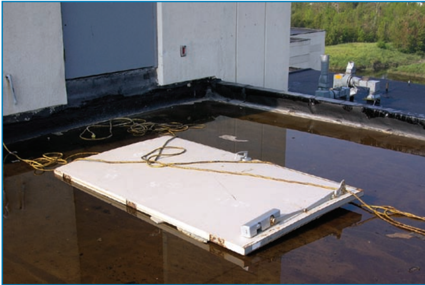
Figure 3-29: Door on a hospital penthouse blown off its hinges during Hurricane Katrina (Mississippi, 2005)
