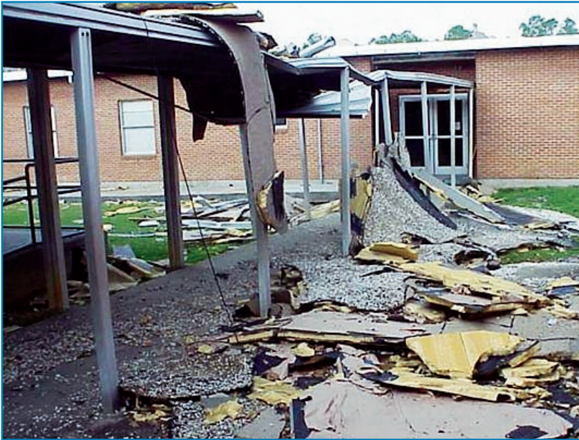
Figure 3-83: Open walkways do not provide protection from wind-borne debris. Hurricane Katrina (Mississippi, 2005)
