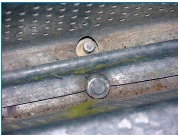
Figure 3-24: Looking down at a sidelap of a deck attached with powder-driven pins. The washer at the top pin blew through the deck.
