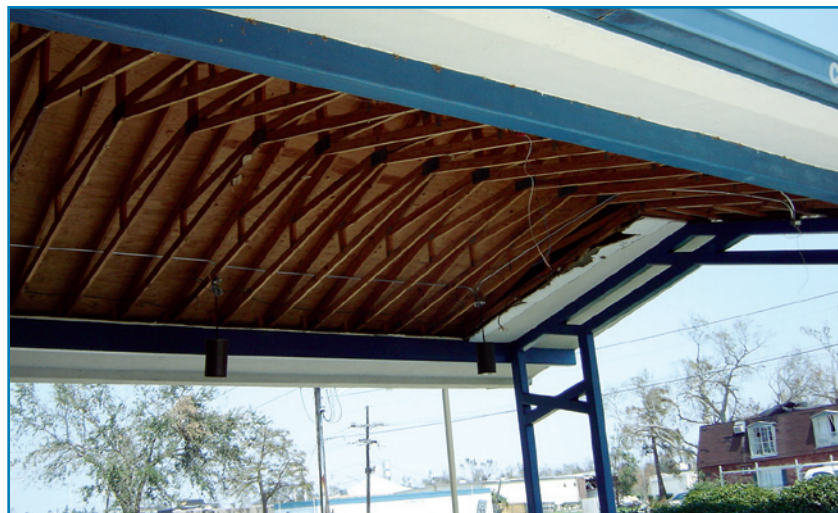
Figure 4-5: Canopy soffit damage at West Jefferson Medical Center
