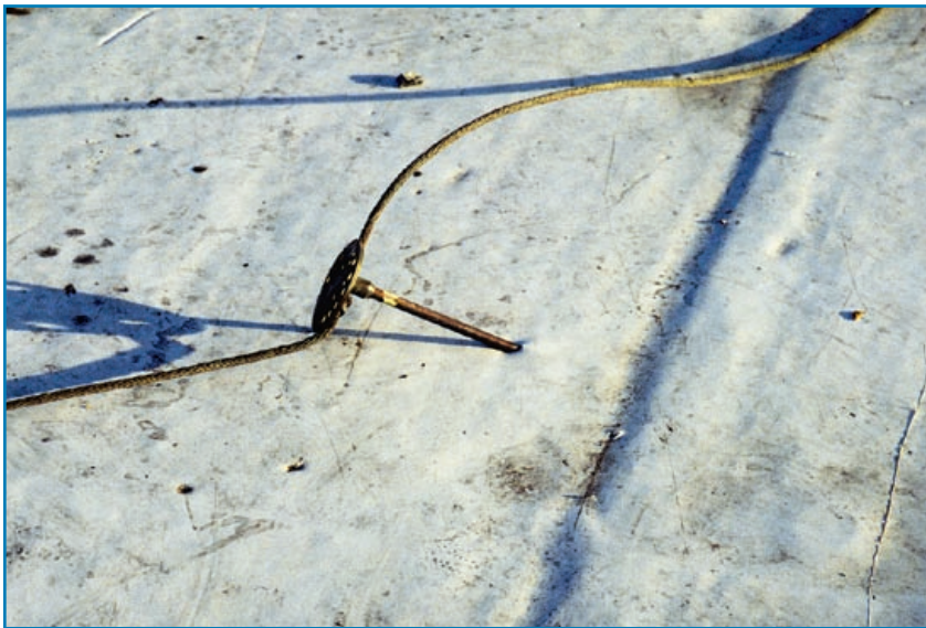
Figure 3-94: A displaced air terminal that punctured the membrane in several locations. Hurricane Marilyn (U.S. Virgin Islands, 1995)
