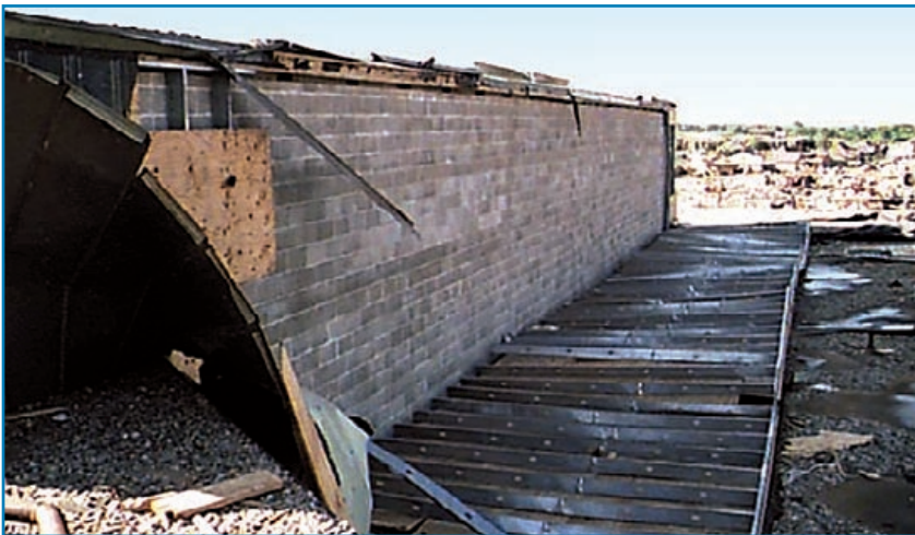
Figure 3-14: Collapsed metal stud wall—the wall was blown completely away in another part of the building. (Oklahoma, 1999)
