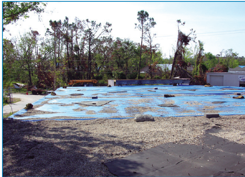
Figure 4-44: Roof damage at Hancock County EOC
