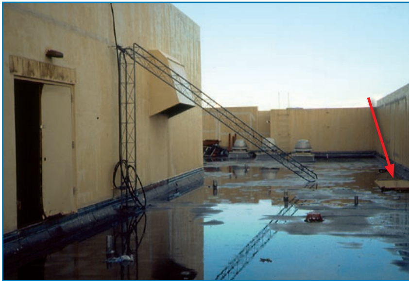
Figure 3-118: The antenna at this hospital collapsed and was whipped back and forth across the roof membrane. Hurricane Andrew (Florida, 1992)
