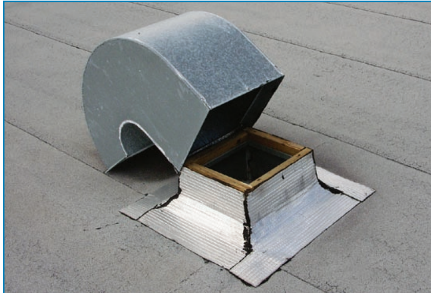
Figure 3-68: This gooseneck was attached with only two small screws. A substantial amount of water was able to enter the building during Hurricane Francis. (Florida, 2004)
