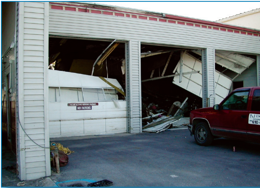
Figure 4-45: Damaged apparatus bay doors at Port Sulphur Volunteer Fire Department.
