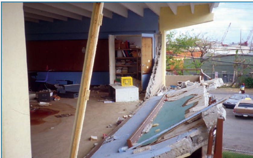
Figure 3-15: The unreinforced CMU wall collapsed at a school during Hurricane Marilyn. (U.S. Virgin Islands, 1995)
