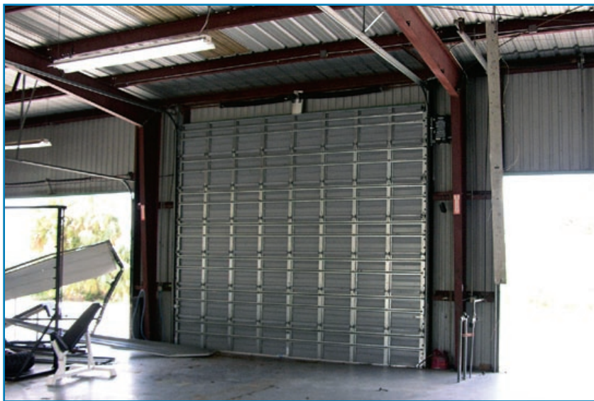
Figure 3-109: The new door in the center performed very well, but the older doors on either side of it were blown away. Hurricane Charley (Florida, 2004)
