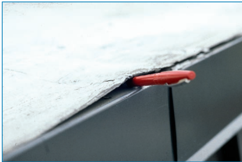
Figure 3-61: The ink pen shows an opening that the wind can catch, and cause lifting and peeling of the membrane.
