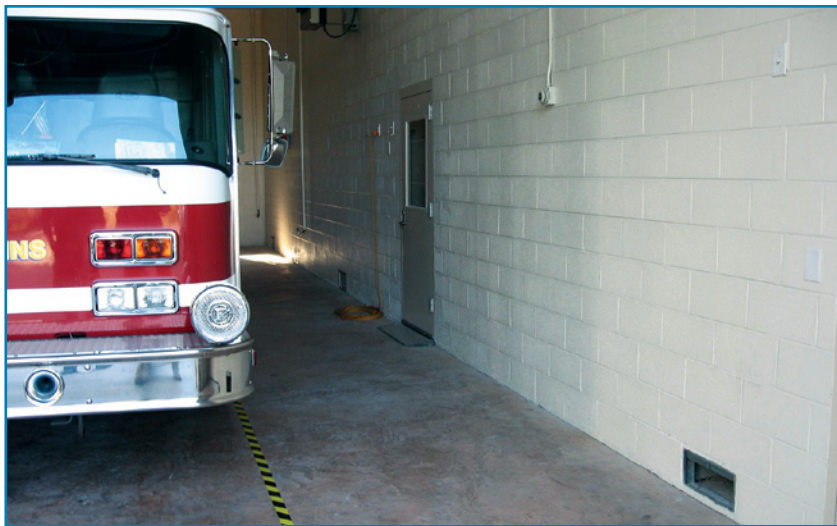
Figure 2-35: The enclosed entry and storage area to the right of the fire truck bays were retrofitted with flood openings.
