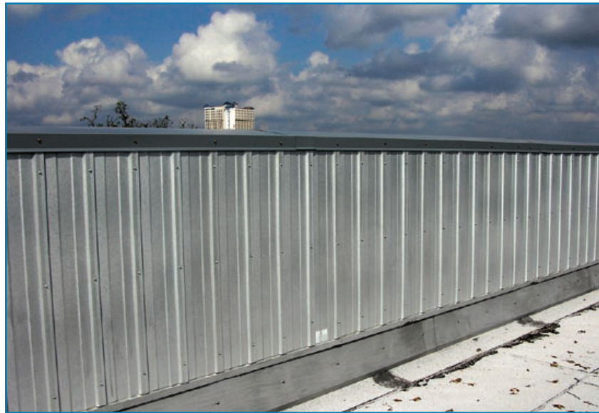
Figure 3-93: Base flashing protected by metal panels attached with exposed screws. Hurricane Katrina (Mississippi, 2005)
