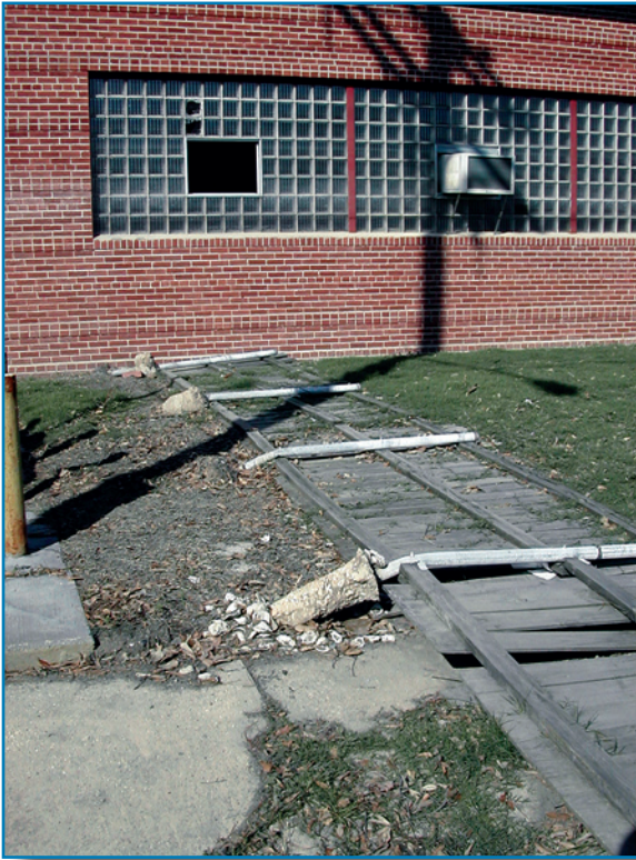
Figure 2-12: Katrina's storm surge flooding knocked down this fence adjacent to a fire station (2005).
