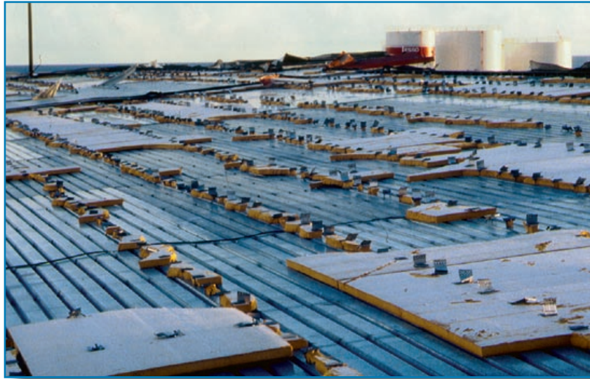
Figure 3-87: Significant interior water damage and facility interruption occurred after the standing seam roof blew off. Hurricane Marilyn (U.S. Virgin Islands, 1995)
