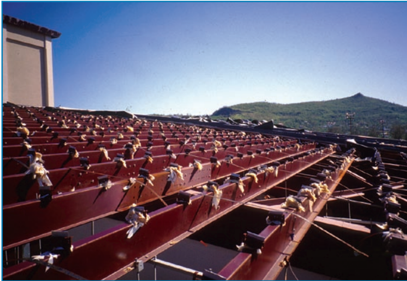
Figure 3-17: A massive quantity of water entered the building after the roof blew off. Typhoon Paka (Guam, 1997)
