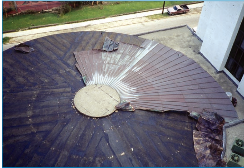
Figure 3-86: Because this roof system incorporated a secondary membrane, the ICU was not evacuated after the copper roof blew off. Hurricane Andrew (Florida, 1992)
