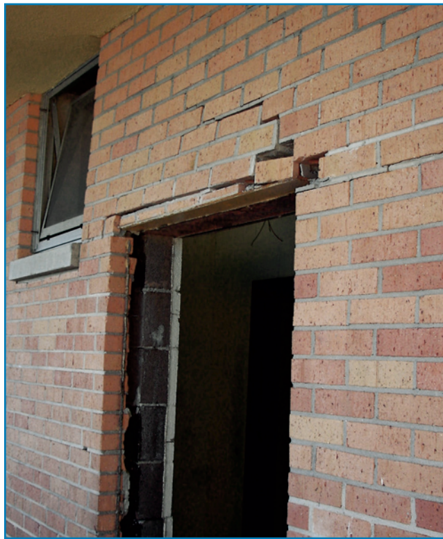
Figure 2-28: Brick facing separated from the masonry wall at Port Sulpher High School, LA.
