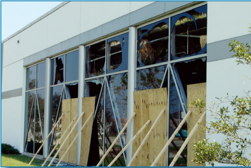
Figure 4-10: Broken windows at West Jefferson Medical Center
