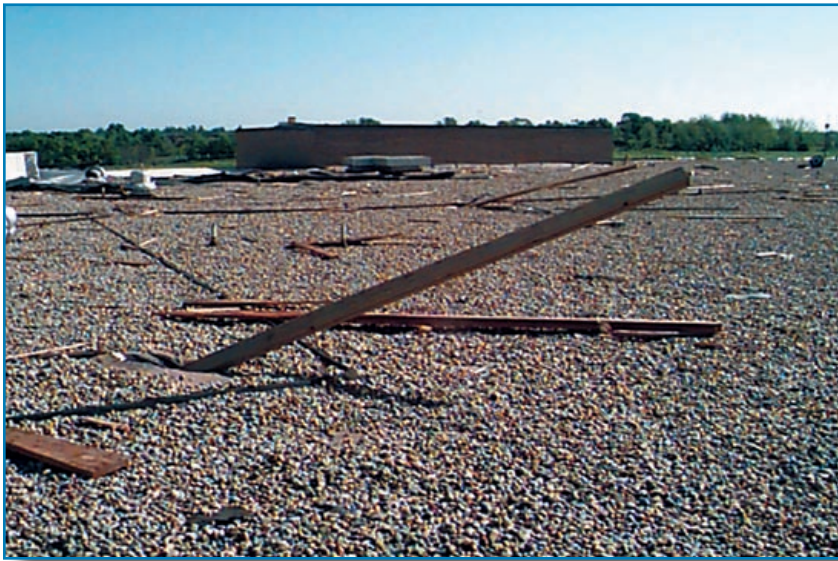
Figure 3-103: A violent tornado showered the roof of this school with missiles. (Oklahoma, 1999)
