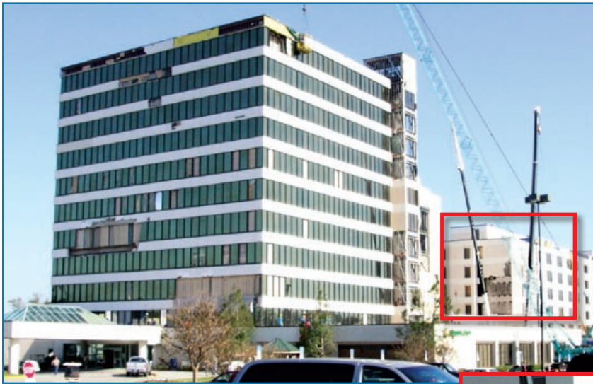
Figure 3-56: EIFS debris blown off the hospital building in the background (red square) broke numerous windows in the MOB in the foreground. Hurricane Ivan (Florida, 2004)
