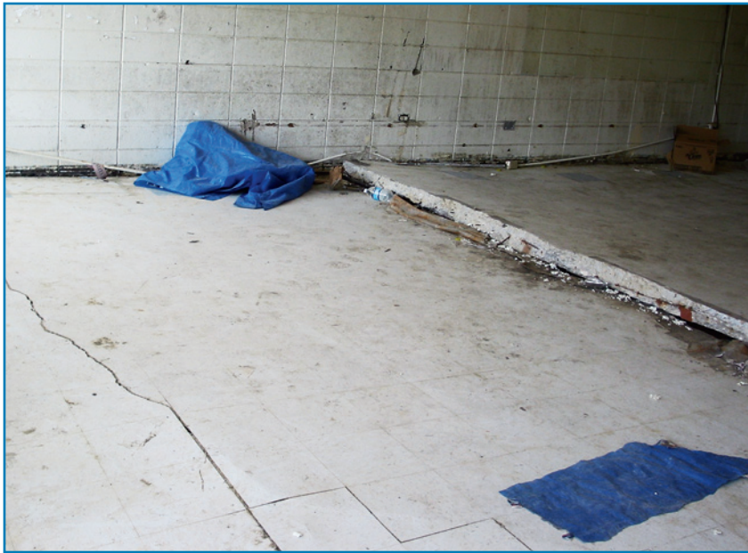
Figure 2-15: Concrete floor ruptured by hydrostatic pressure (buoyancy). Hurricane Katrina (2005)
