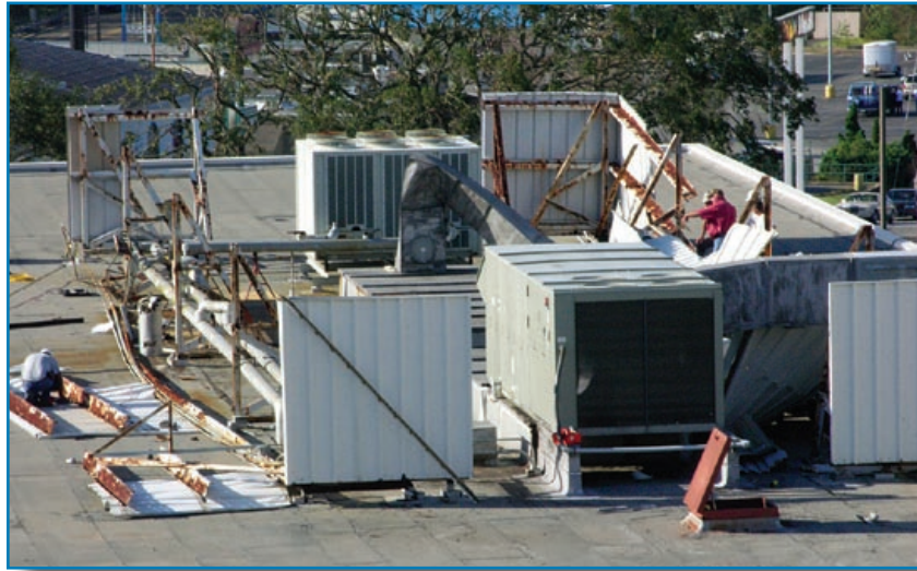
Figure 3-77: Equipment screen panels, such as these blown away at a hospital, can break glazing, puncture roof membranes, and cause injury. Hurricane Ivan (Florida, 2004)
