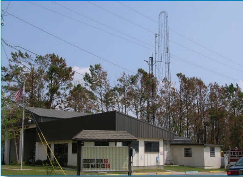
Figure 3-80: The antenna tower at this fire station buckled. Hurricane Katrina (Mississippi, 2005)
