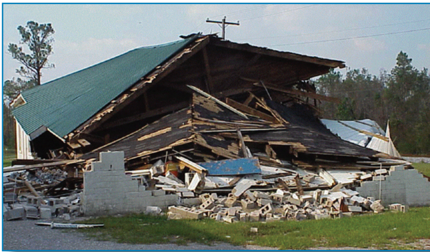
Figure 4-21: Collapsed portion of the Lyman Elementary School Building
