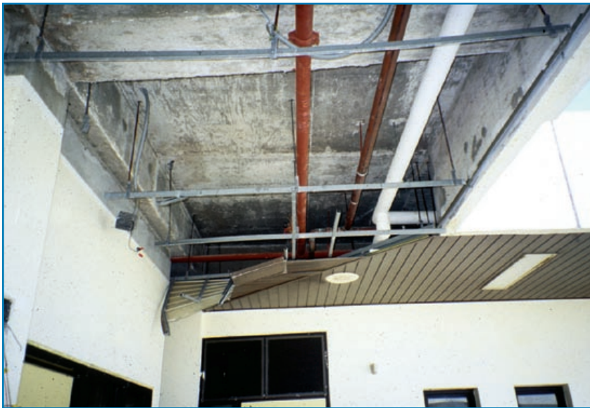
Figure 3-42: This suspended metal soffit was not designed for upward-acting wind pressure. Typhoon Paka (Guam, 1997)
