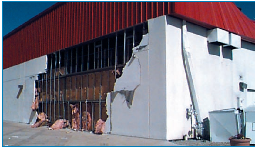
Figure 3-54: EIFS blow-off at building corner. In places, metal fascia was also blown in. Tornado (Oklahoma, 1999)
