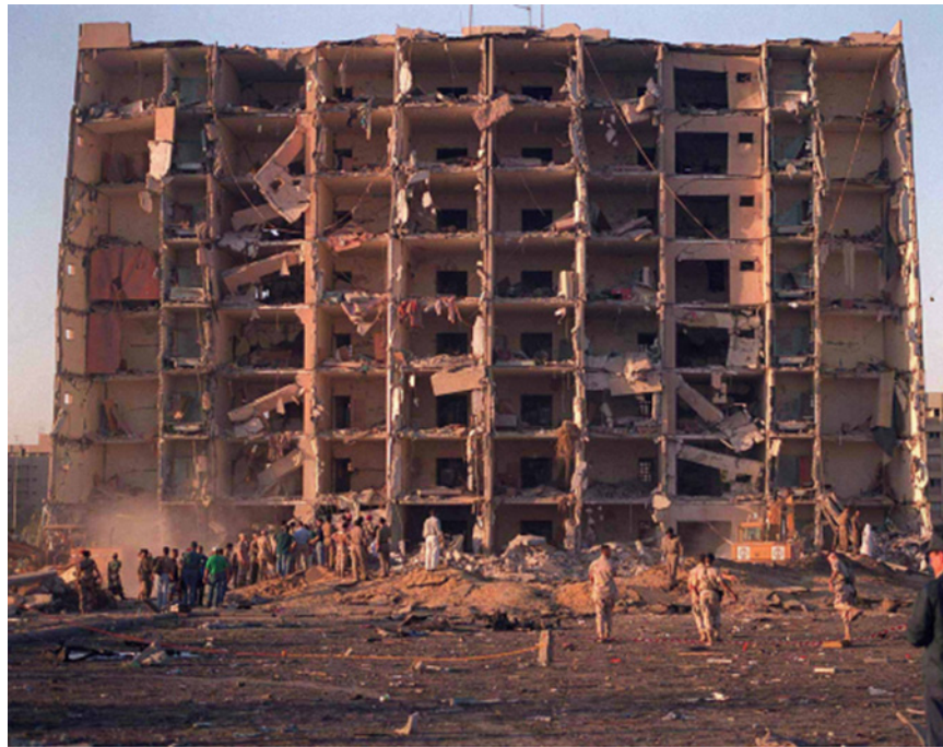
Figure 4-4 Exterior view of Khobar Towers exterior wall failure
