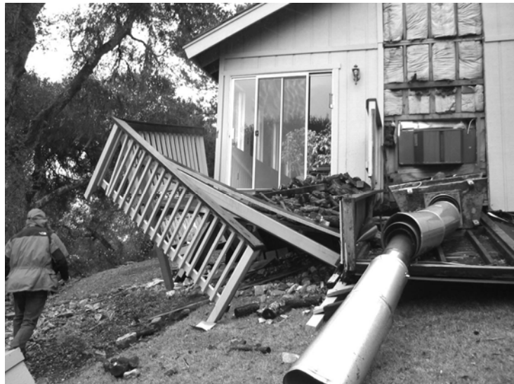
Figure 7-8 Collapsed factory-built chimney, light-frame enclosure, and deck after the San Simeon earthquake. Photo courtesy of Josh Marrow, Simpson Gumpertz and Heger Inc.
