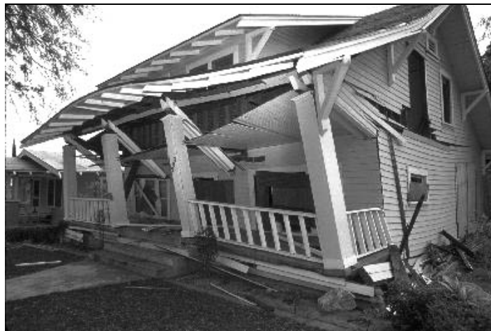
Figure 9-5b A house with severe damage due to cripple wall collapse. Photo Courtesy of FEMA.
