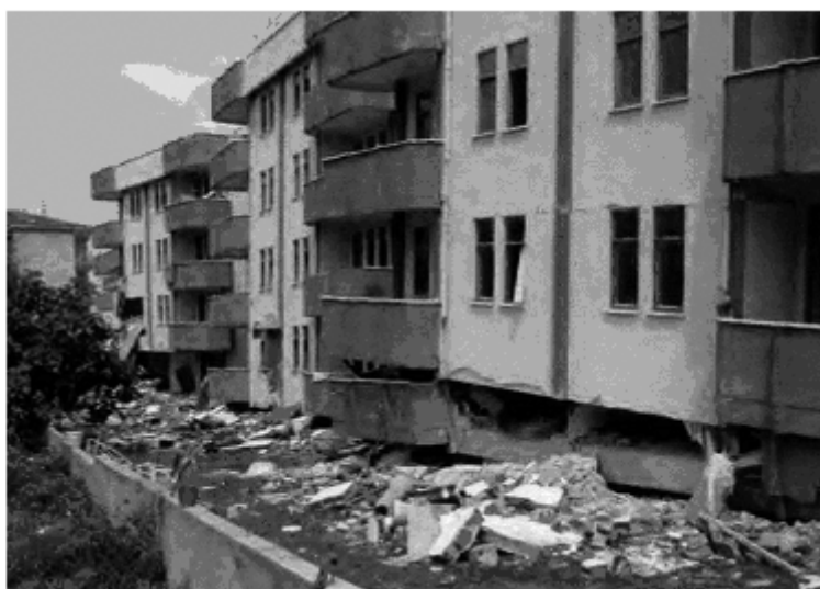
Figure 2-16 Apartment building experiencing soft- and weak-story behavior in the Northridge earthquake. The two balcony rails with little separation at the center of the photo illustrate the collapse of the lowest story.
