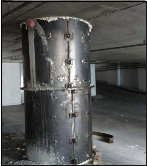
Damaged columns with completed encasement
