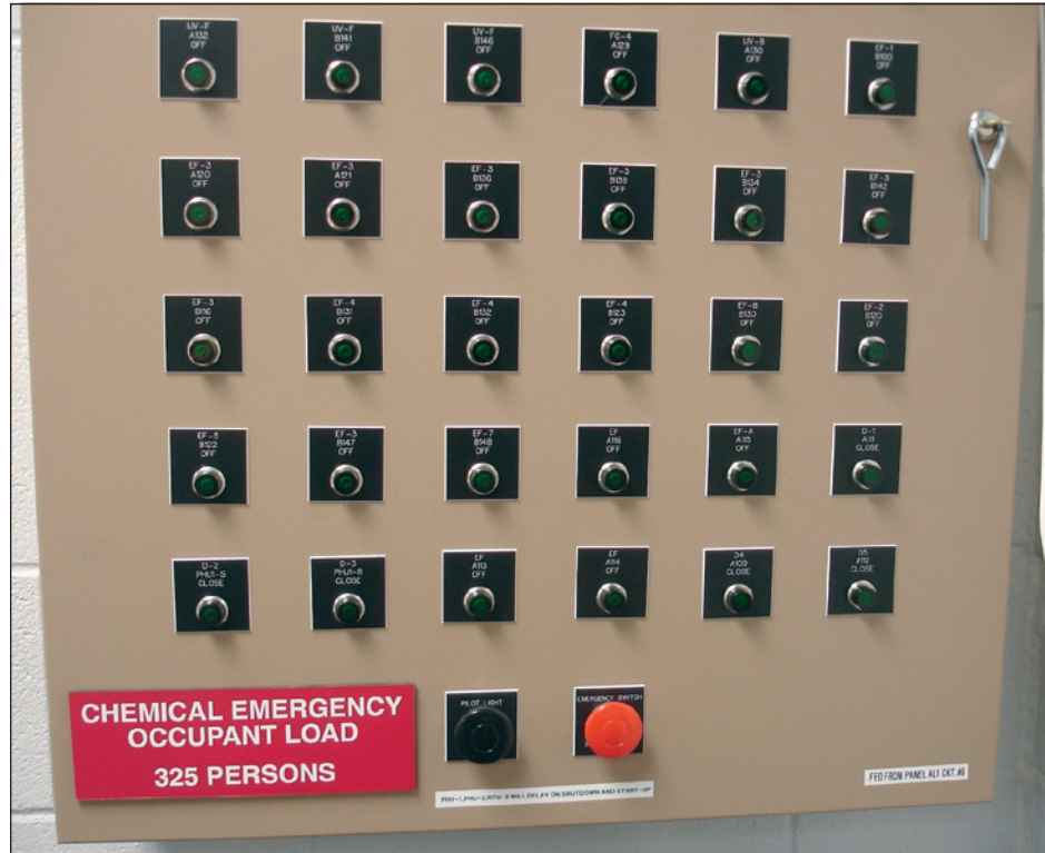
Figure 5-4: A sheltering control panel in a school with a fan-shutdown switch (red push switch at lower center) and indicator lights for status of dampers and fans
