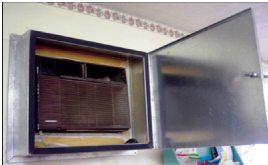
Figure 5-3: Manually operated damper for sealing an air conditioner in a safe room
