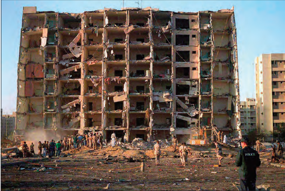
Figure 3-36: Khobar Towers, Dhahran, Saudi Arabia, 1996
