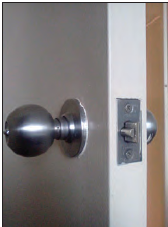
Figure 100: Example of fire door in commercial building
