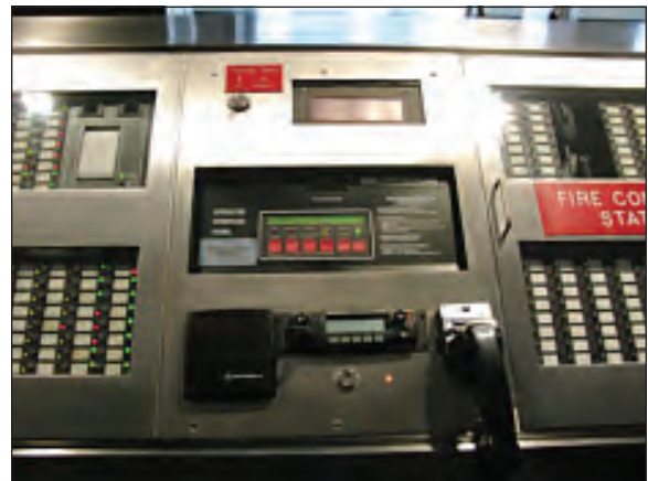
Figure 102: Example of fire alarm control panel in commercial building
