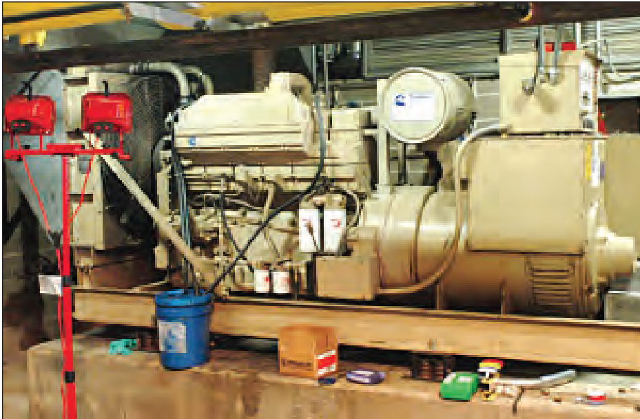
Figure 105: Example of a generator found in a commercial building
