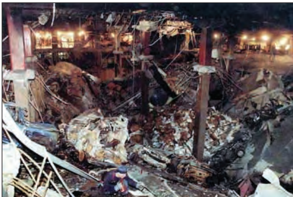
Figure 1-4: Underground damage after the 1993 World Trade Center bombing
