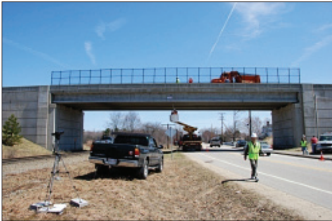
Figure 3-32: Digital Camera Set up for Digital Image Correlation at Rollins Road Bridge
