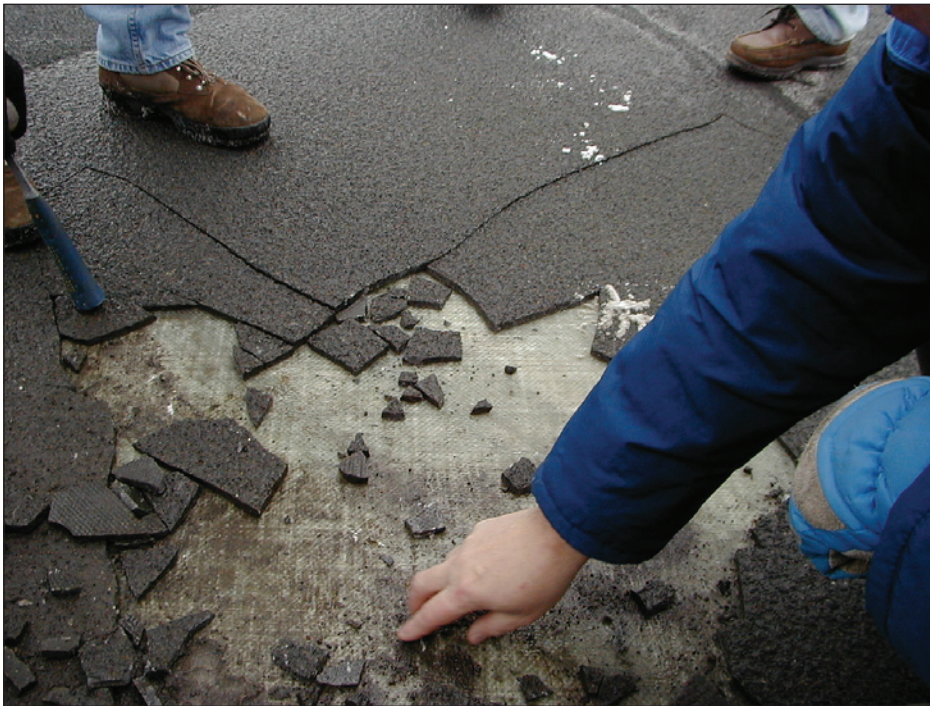
Figure 3-49: Wearing Surface Debonded from FRP Deck
