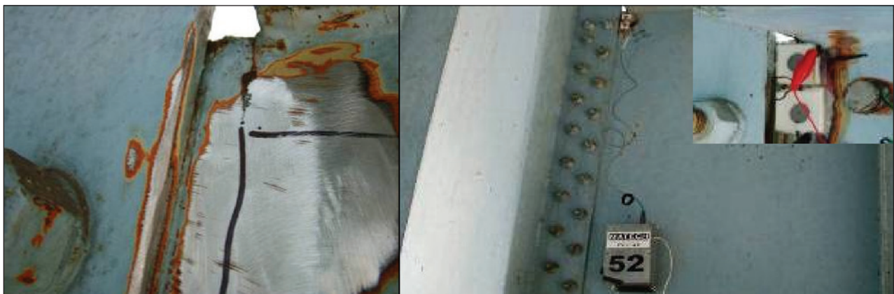
Figure 5-26: Typical cracked coped detail at the floor beam to girder connection. Photo on the right shows the detail with the EFS installed.
