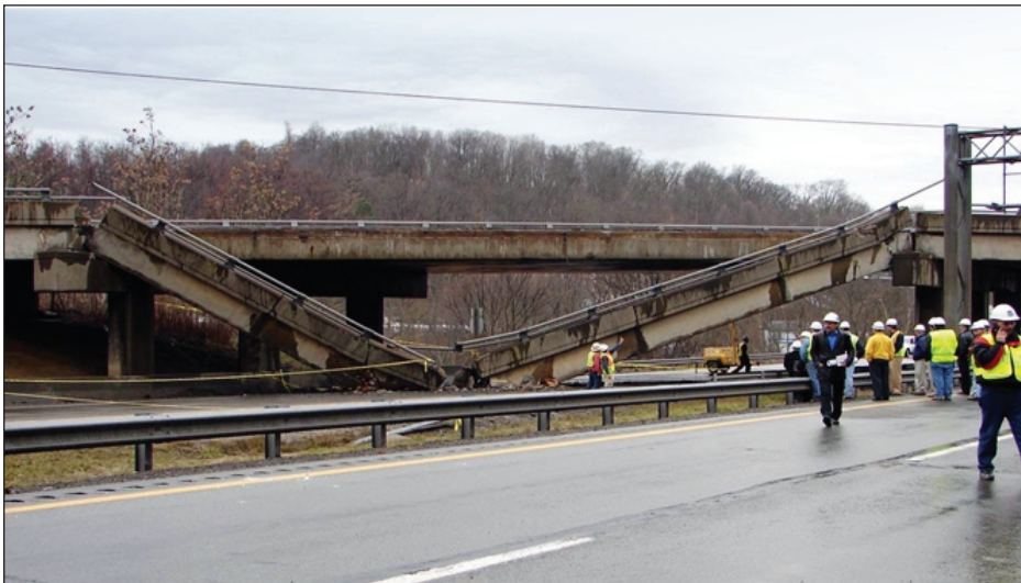
Figure 3-2: Box Beam Bridge Failure in Pennsylvania
