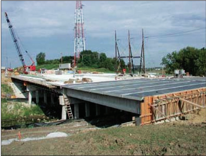
Figure 3-46: Prefabricated FRP deck being installed on prefabricated prestressed concrete beams. Bettendorf, Iowa.
