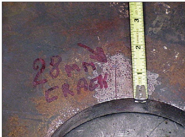
Figure 3-8: Cracked eye-bar of suspension bridge
