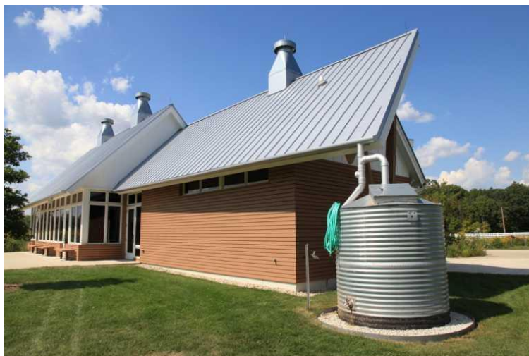
Figure 1. Picture of a rainwater rooftop collection system with an outdoor, aboveground storage tank. Notice that the gutter drainage includes a first flush diverter (the portion of pipe bypassing the storage tank). 1
