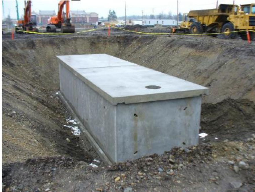
Figure 8. A concrete rainwater collection vault used in the renewal barracks project at JBLM. (Source: USACE, Seattle District)
