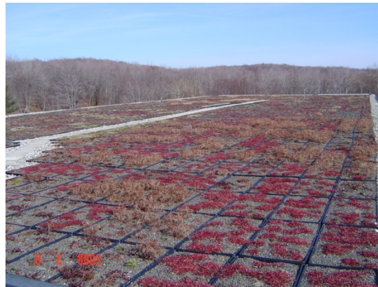
Figure 5. Modular Green Roof trays (Source: USACE, Baltimore District)
