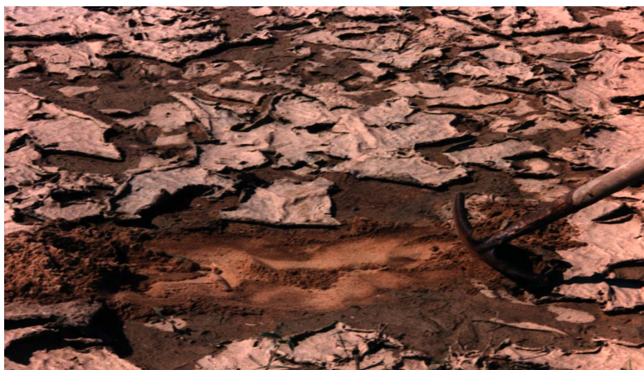
Figure 3. Dried matted material on the surface of a sand filter.
