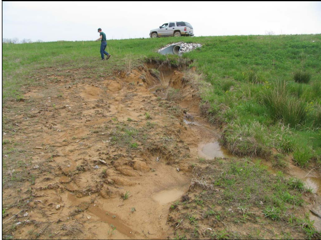
Figures A-4 and A-5: Gully erosion due to inadequate drainage system protection.
