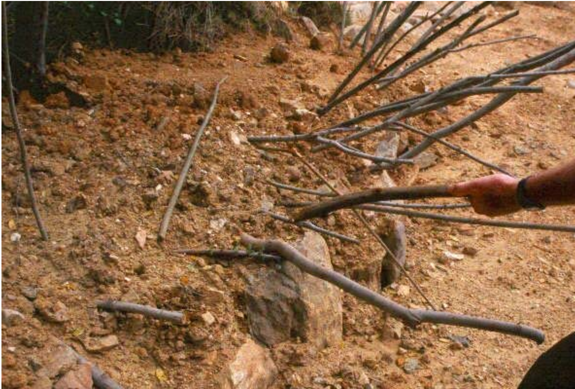
Figure B5. Live staking on a hill slope, done during dormancy (BioDRAW®).
