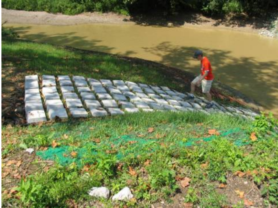
Figure C14. Demonstration site 1 month post-construction, looking at upstream southwest corner (see Figure C9).
