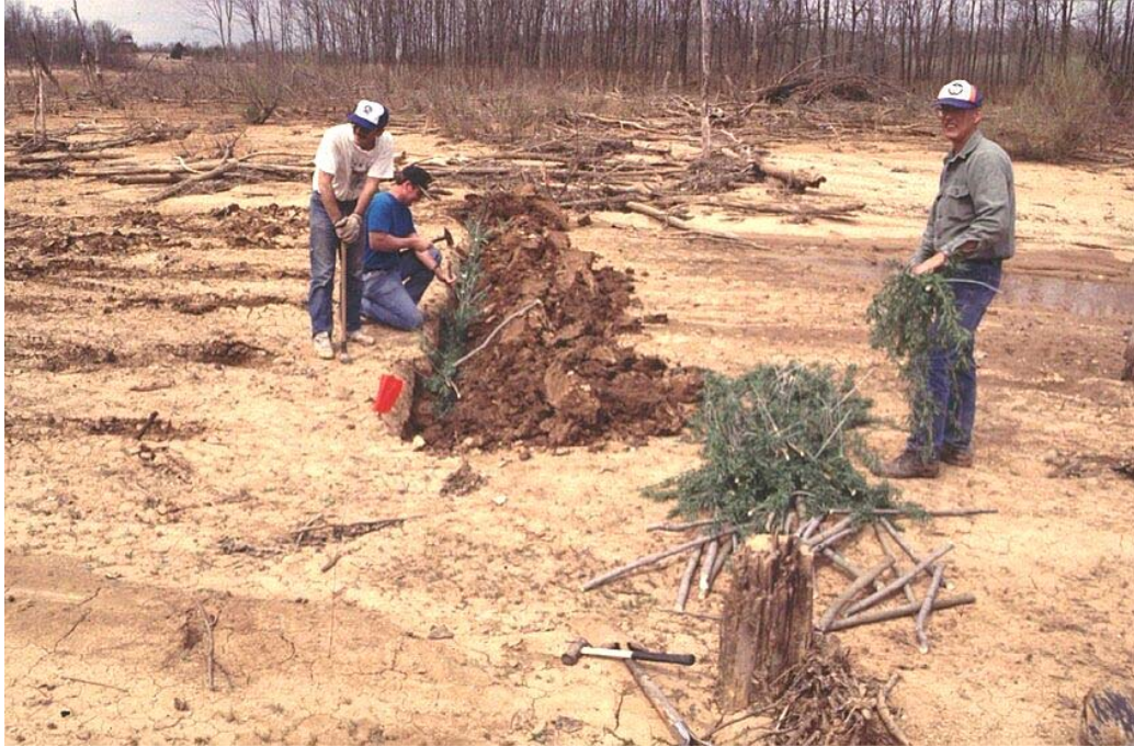
Figure B3. Live staking in combination with bundles/wattles at Fort Leonard Wood, MO (J. Proffitt, Fort L. Wood).
