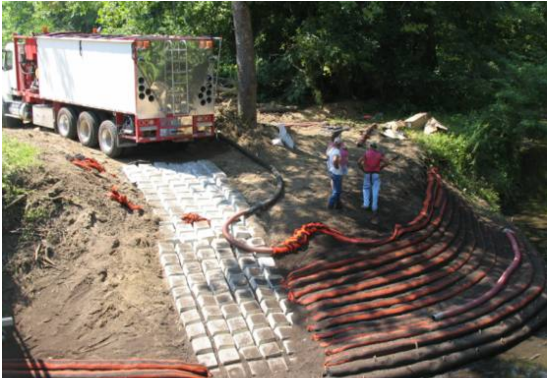
Figure C9. Demonstration site during construction, southwest. A cabled-concrete™ access ramp was installed along with a Filtrex™ compost-sock system.
