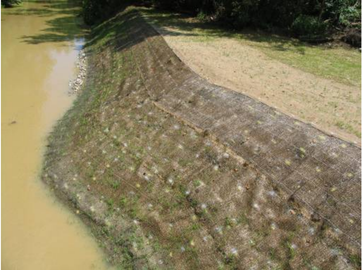
Figure C16. Demonstration site 1 month post-construction, looking at downstream southeast corner. A series of toes were installed along this bank; far west had a fiber-coir biolog with native wetland species, then a section with only a fiber-coir log, followed by a section with minimal riprap, and the final section had only the erosion control blanket.
