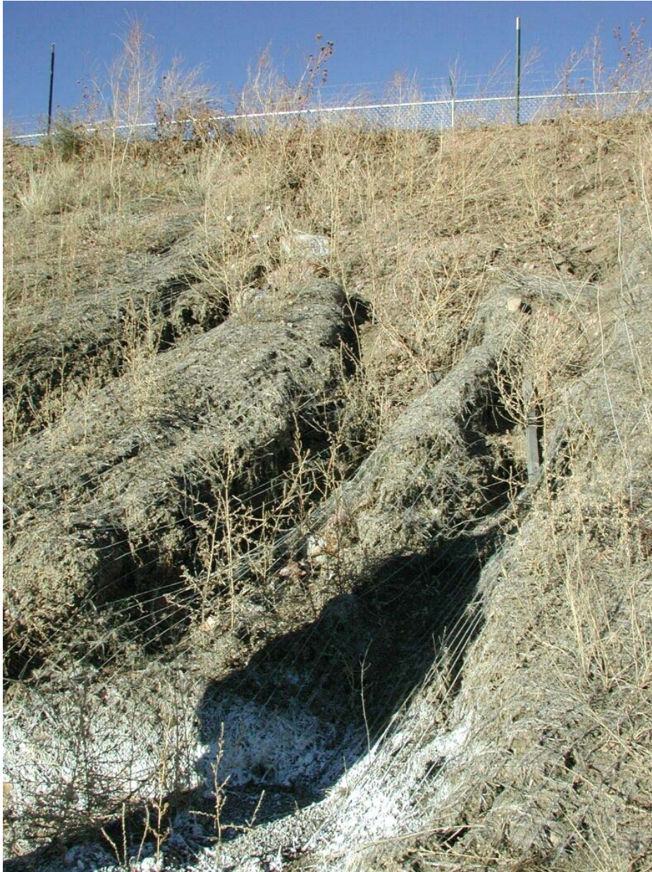
Figure B10. Improper choice and installation of an erosion control blanket along a streambank resulted in failure.
