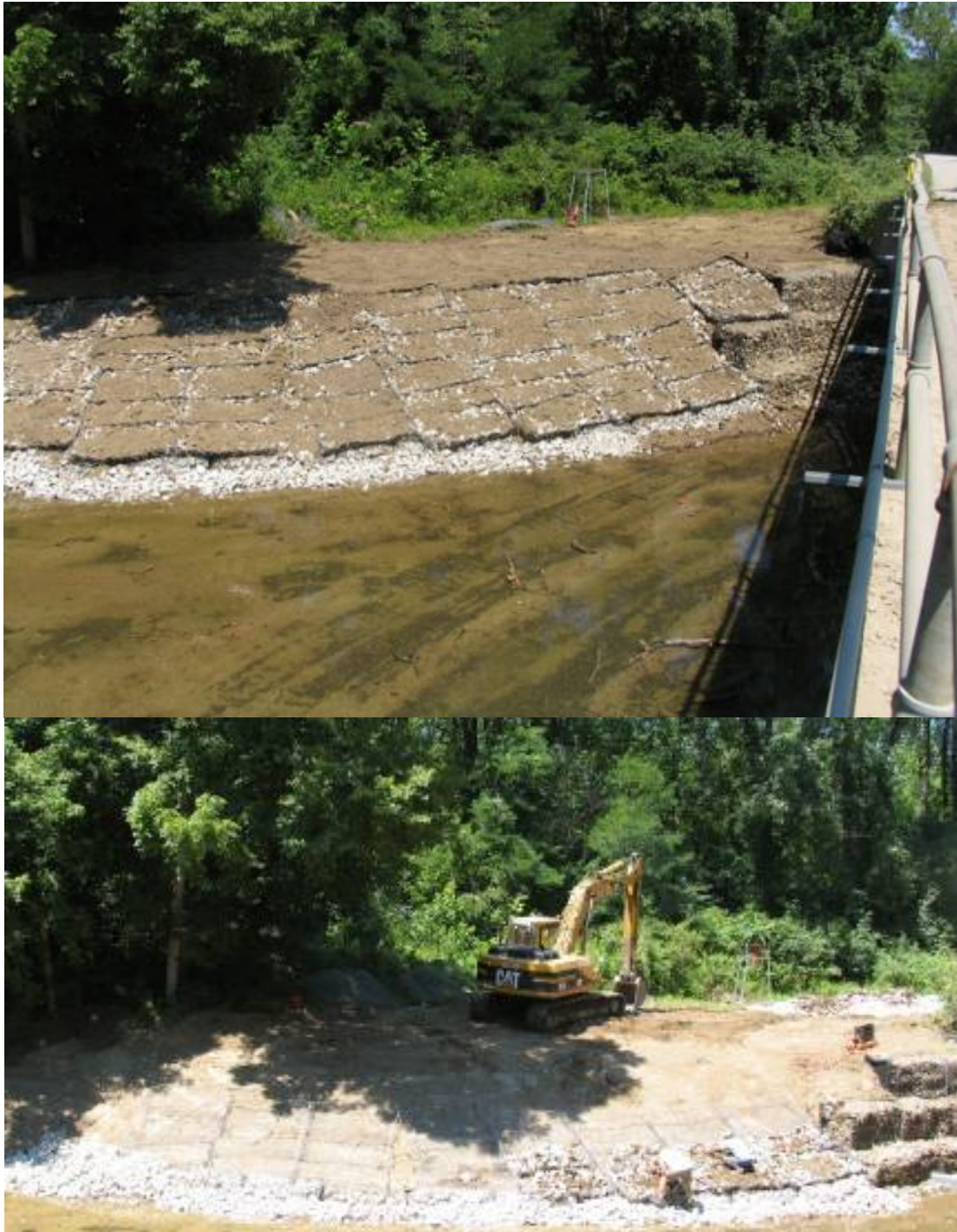
Figures C10 and C11. Demonstration site during construction, northwest. A combination of gabion baskets and gabion mattresses with a riprap toe was installed. Slopes were kept to 2:1, and the gabion mattresses were inoculated with soil and native seeds and overlaid with an erosion control blanket. The top of the streambank was treated with a straw-filled polynet erosion control blanket while a jute blanket was used within the mattresses.
