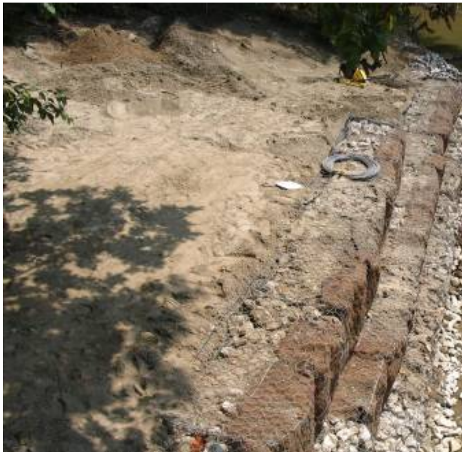
Figure C13. Demonstration site during construction, looking from top of bridge downstream at northeast corner. This view illustrates incorporation of erosion control blankets within gabion baskets and the riprap shelf/toe that was installed to help rebuild the bank.
