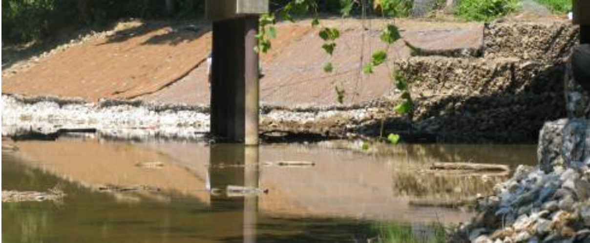
Figure C12. Demonstration site during construction, looking upstream to northwest corner. This view illustrates incorporation of erosion control blankets.
