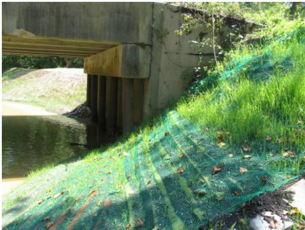
Figure C15. Demonstration site 1 month post-construction, looking downstream from southwest corner. East of the access ramp, filtrex™ overlaid the socks with an erosion control netting (LockDown Netting™).
