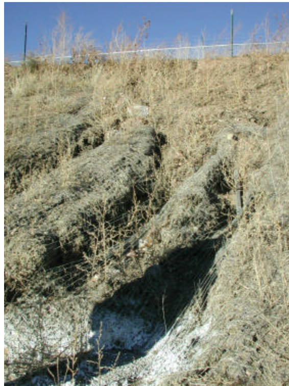
Figure B27. Improper installation and choice of erosion control blanket resulted in failure.
