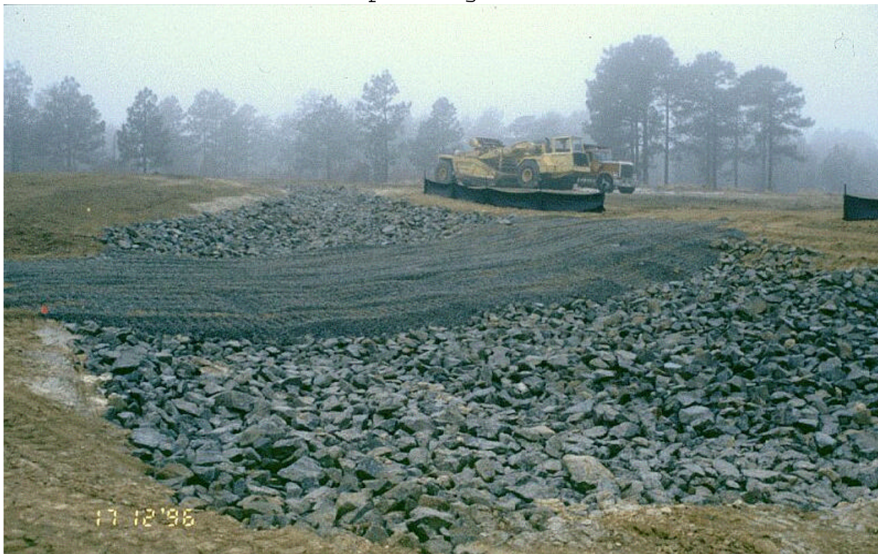
Figure B19. Riprap used on military installation to harden crossing and act as a French drain during high flows.
