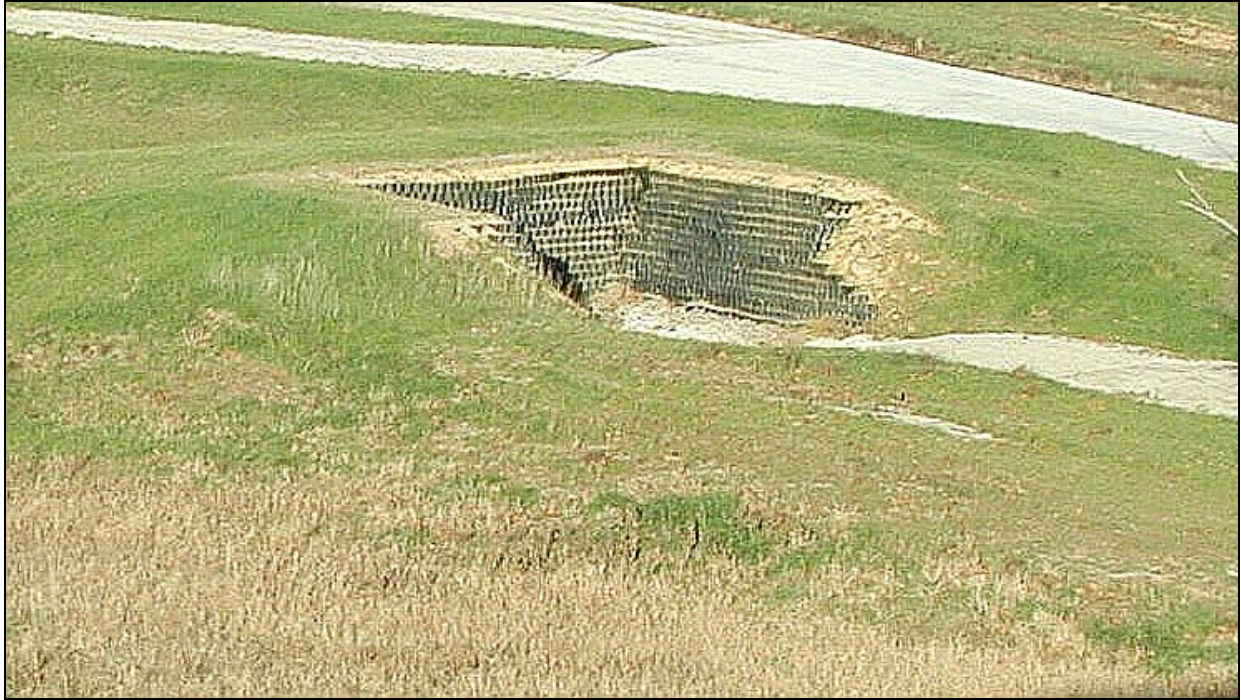
Figure B31. Cellular confinement system used in the construction of a Bradley misfire revetment.
