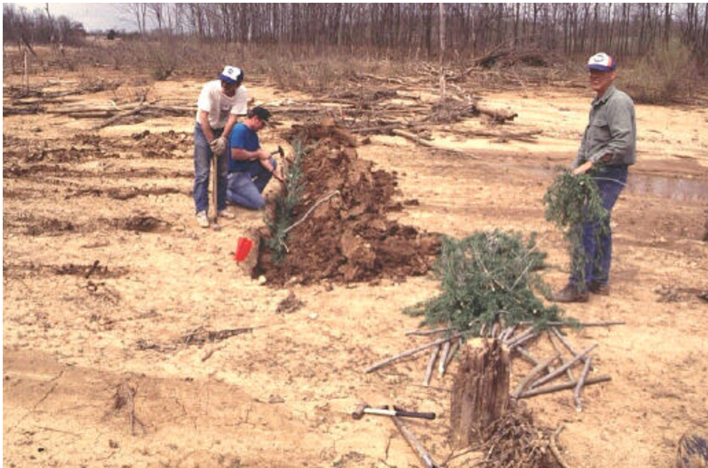
Figure B11. Live staking in combination with bundles/wattles at Fort Leonard Wood (J. Proffitt, Fort L. Wood).
