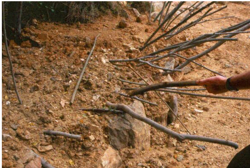
Figure B10. Live staking on a hill slope, done during dormancy (BioDRAW®).
