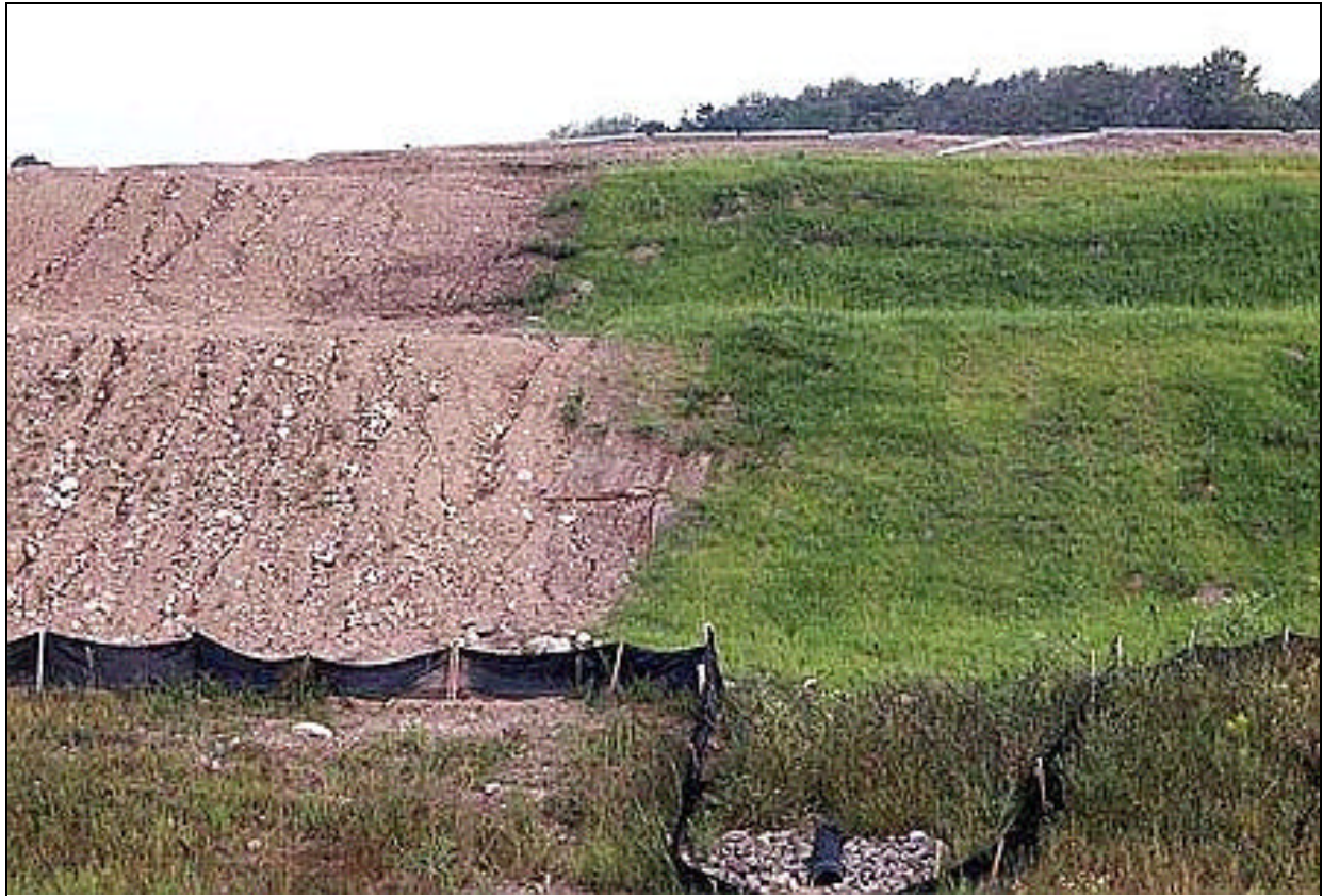
Figure B37. Contrasting terracing system with and without vegetation, illustrating the importance that vegetation has in erosion control (source: IECA).
