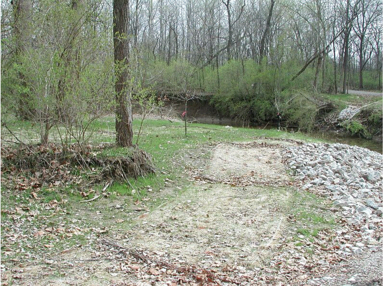
Figure B6. Camp Atterbury used biodegradable erosion control blankets, placed willow wattles as check dams, and planted trees along a disturbed stream bank to help armor the bank against erosion. Note the exposed roots and higher elevation of the mature tree and shrubs.
