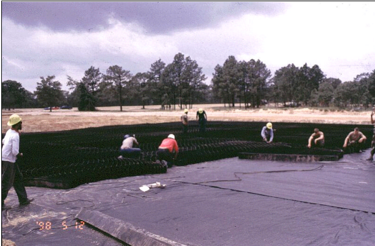
Figure B30. A cellular confinement system with geotextile is being used to harden a helipad and tank trail at Fort Bragg, NC.
