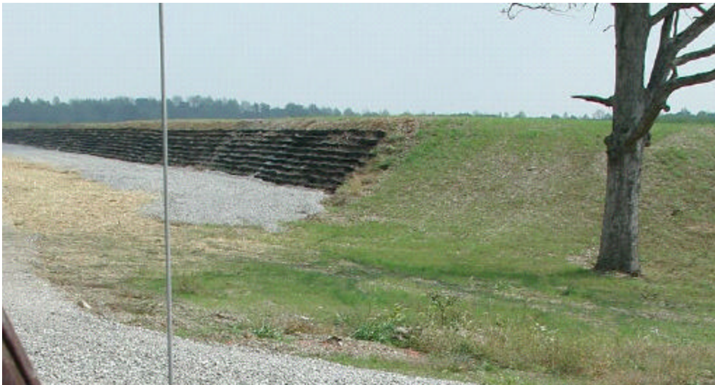
Figure C8. Backside of the MPTR berm. Many of the berms were composed of over 40 layers of GeoWeb ® , obtained by Camp Atterbury after Operation Desert Storm.
