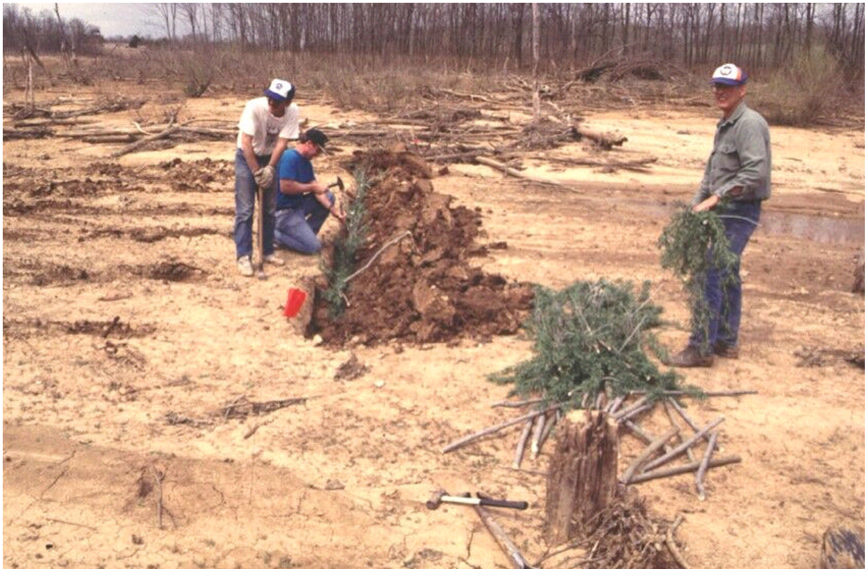
Figure C9. Installation of wattle and post system along a sediment basin at Fort Leonard Wood (J. Proffit, Fort Leonard Wood).
