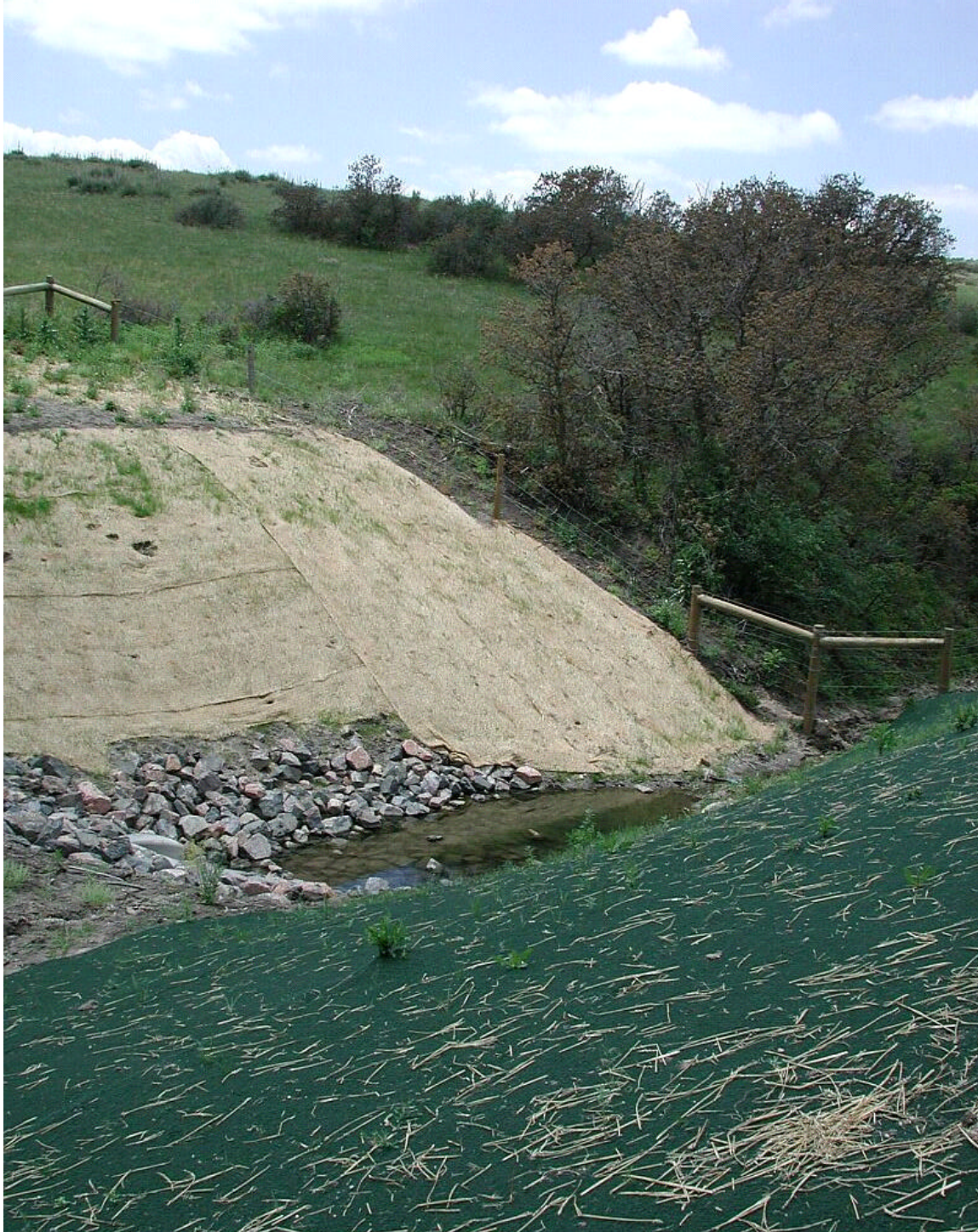
Figure B29. Demonstration of two different blankets, biodegradable jute and synthetic polymer, indicate that the biodegradable blanket performed better. The synthetic blanket had increased erosion underneath, which could have been a result of poor grading.
