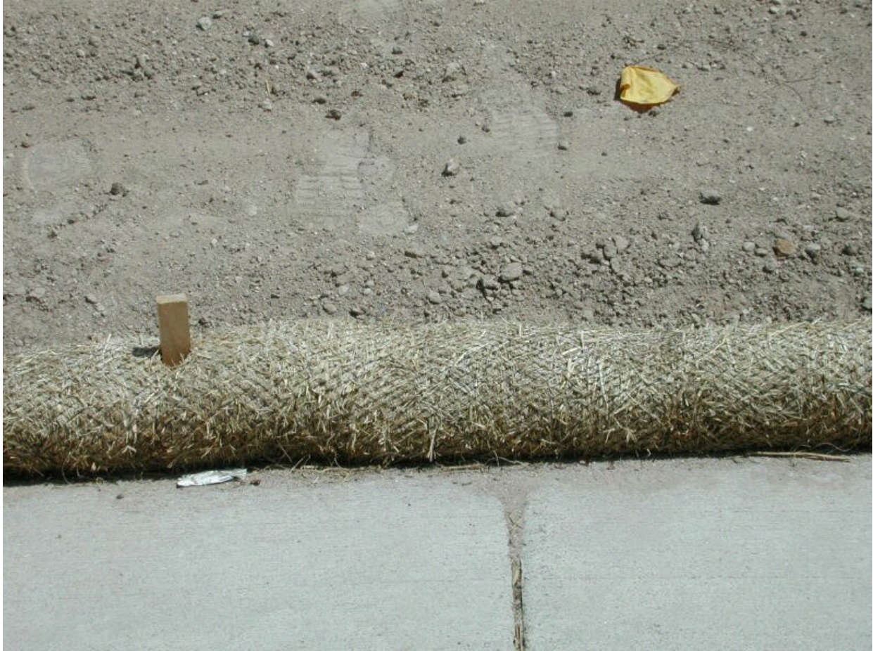
Figure B16. Straw log used to control sediments on a construction site in Colorado.
