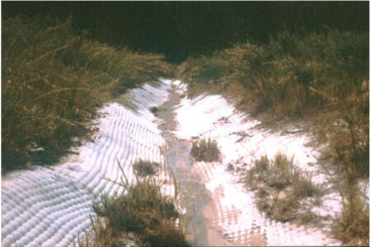
Figure B28. A permanent structural mat was chosen to help stabilize this waterway and increase its longevity (source: USDA).
