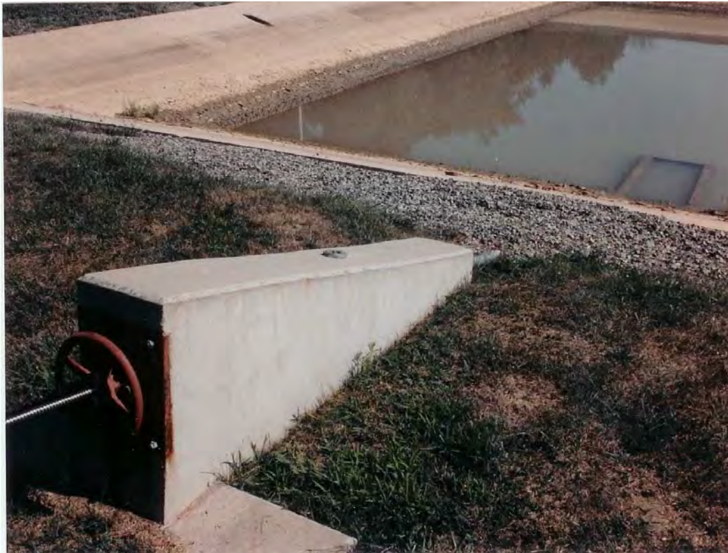
Figure A-35. Nearly empty equalization basin – outlet box and outlet valve wheel are shown (photo by ERDC-CERL).
