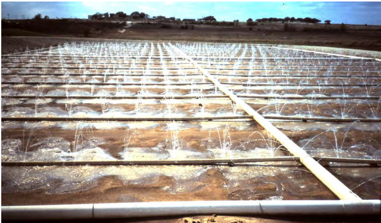
Figure A-25. Sand filter being dosed (photo by ERDC-CERL).
