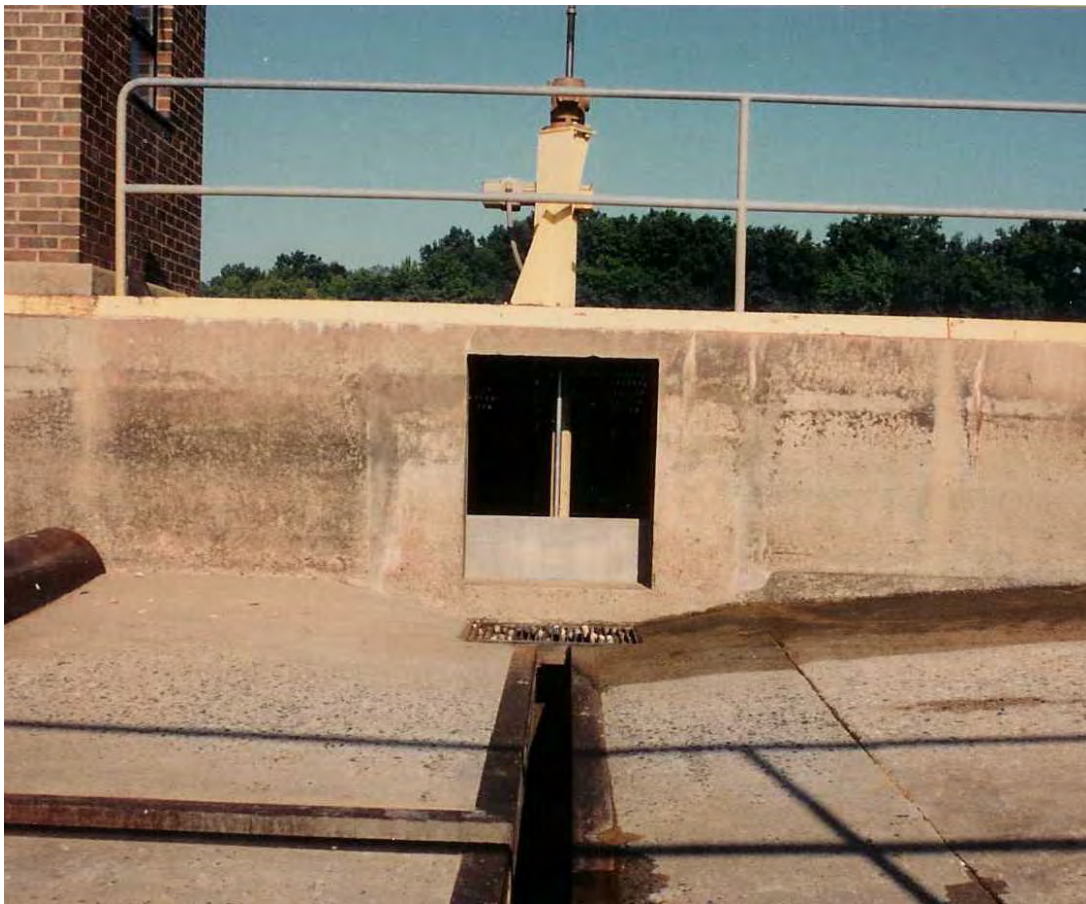
Figure A-12. Water level control structure (photo by ERDC-CERL).
