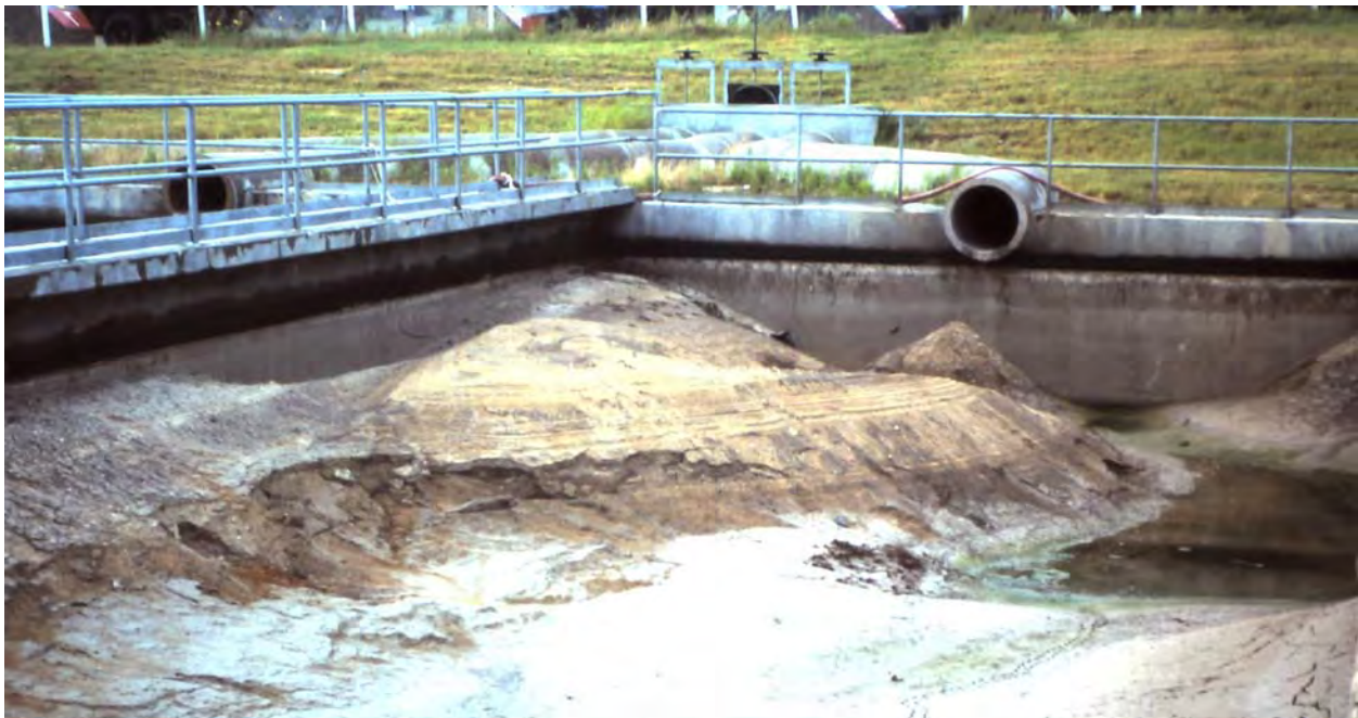
Figure A-31. Drained sedimentation basin prior to a cleanout (photo by ERDC-CERL).
