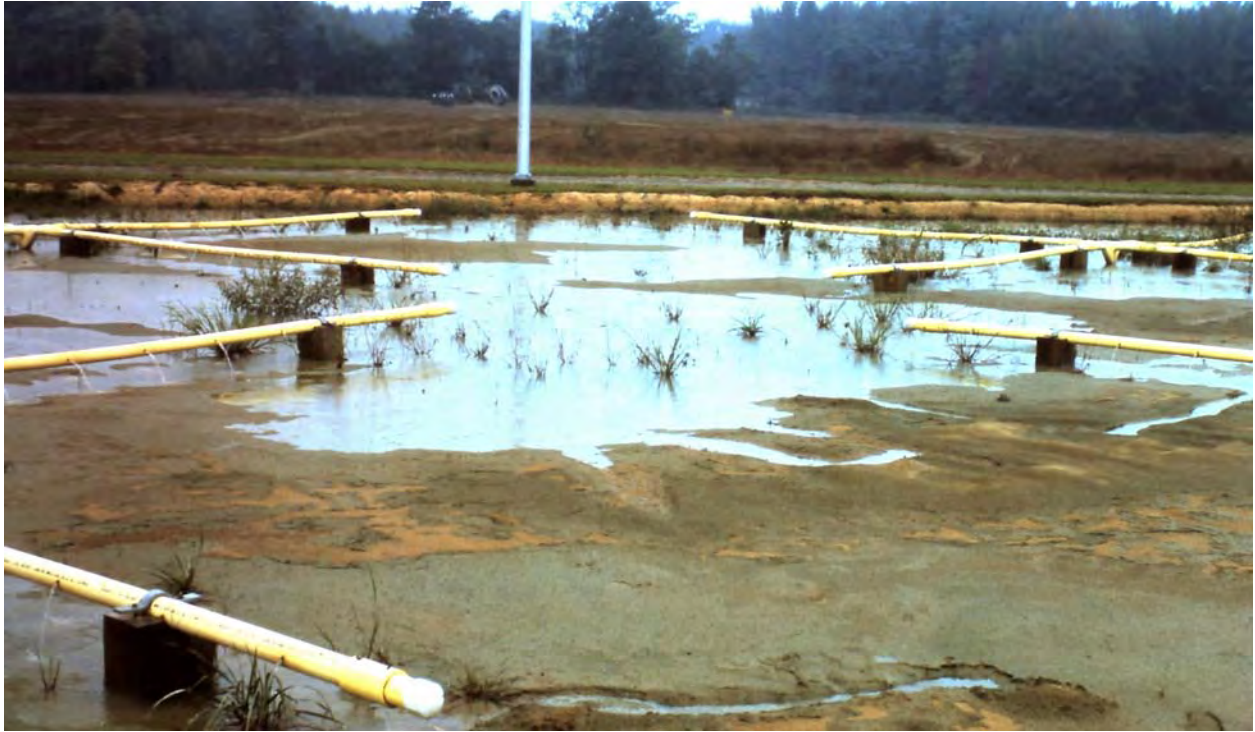
Figure A-36. Ponding on an intermittent sand filter (photo by ERDC-CERL).
