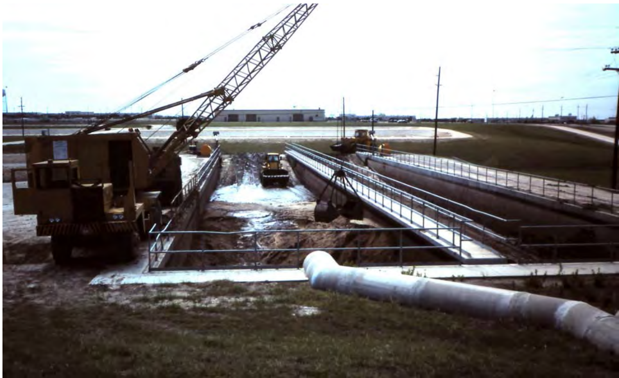
Figure A-33. Front-loader and clamshell crane used to clean out basin (photo by ERDC-CERL).
