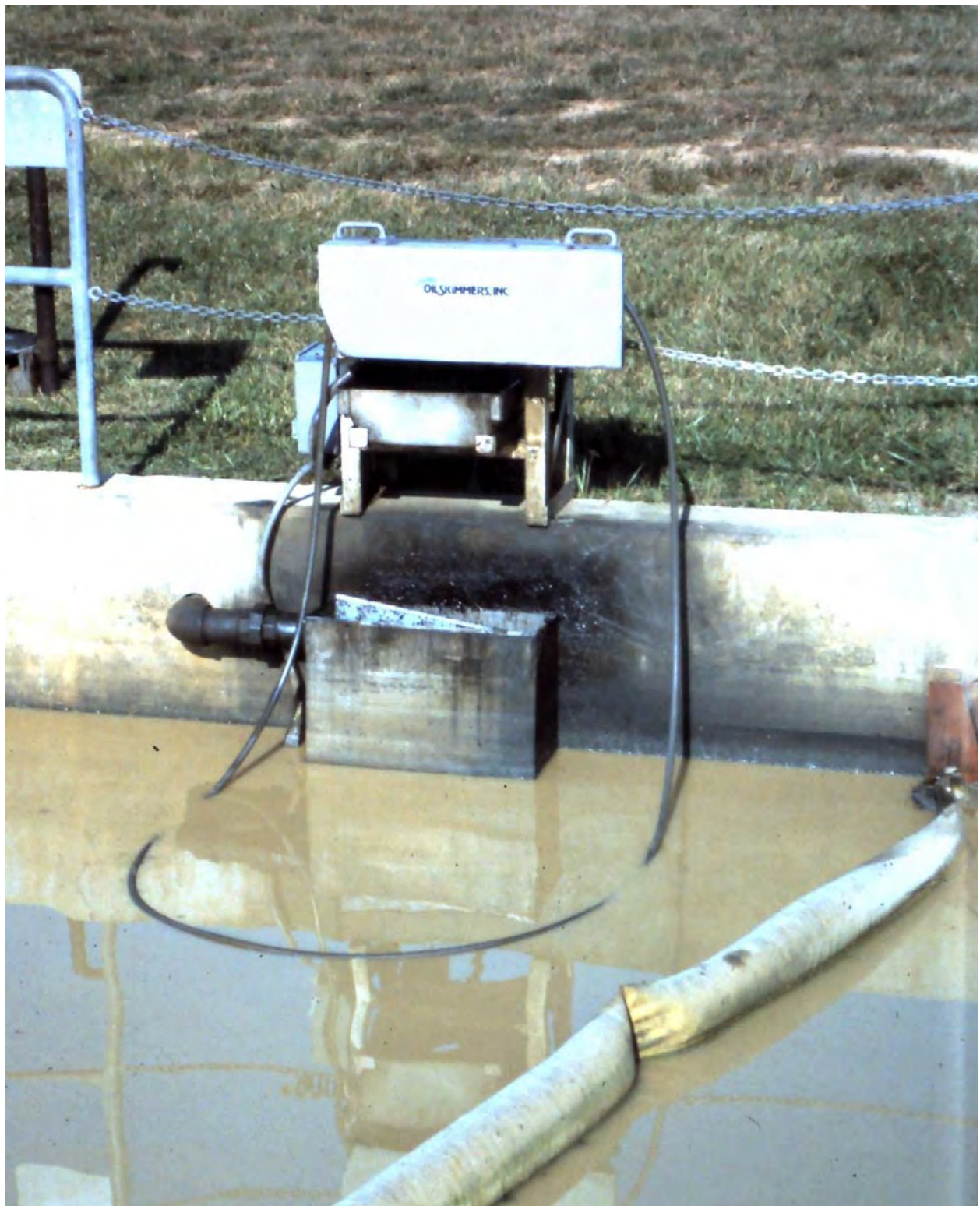
Figure A-22. Floating tube oil skimmer (photo by ERDC-CERL).
