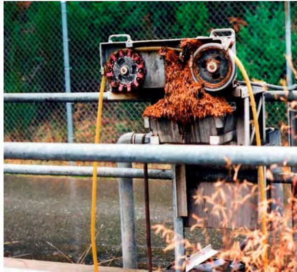
Figure A-30. Oil skimmer clogged with pine needles (photo by ERDC-CERL).
