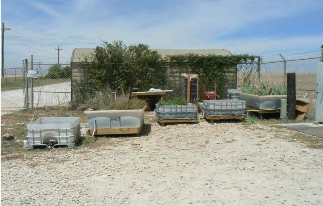
Figure A-14. Complete microbial mat and polishing treatment system (View 1).
