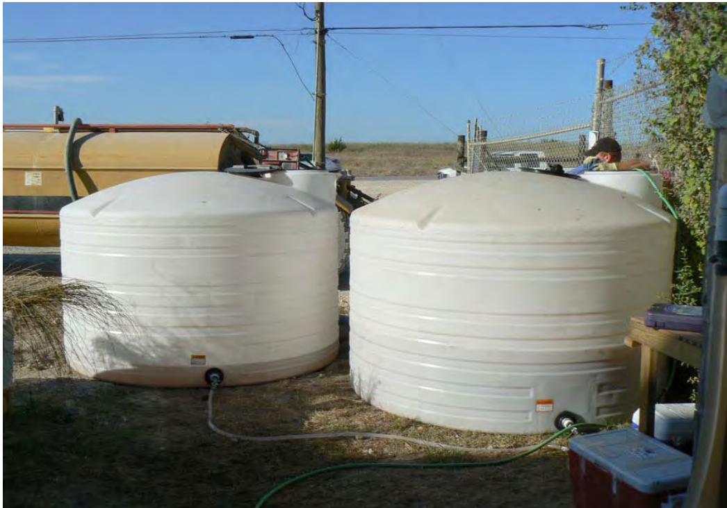
Figure A-2. Leachate storage tanks.
