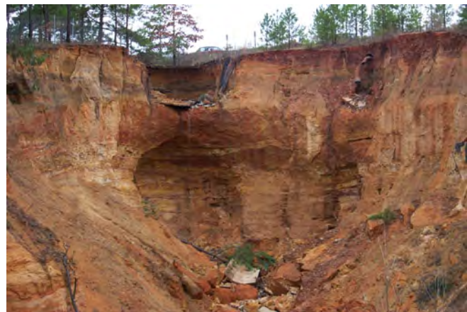
Figure A-3. This gully at Kelley Hill, Fort Bragg, started at the stormwater outfall.
