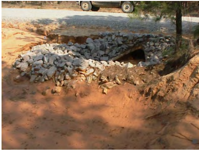
Figure A-4. Riprap placed around this culvert inlet is not the appropriate solution to the erosion problem.
