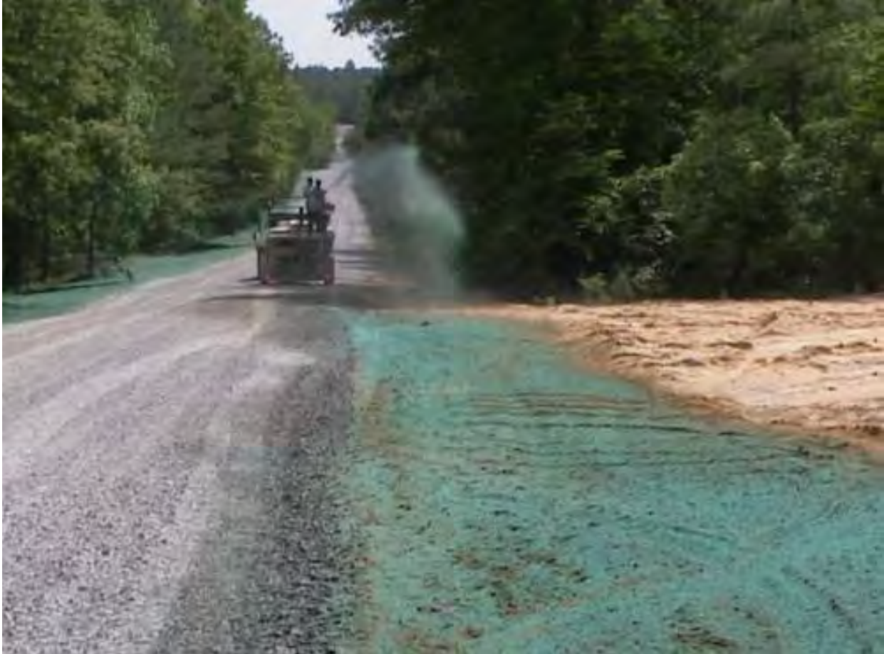
Figure B-4. The hydroseeding process sprays seed, mulch, and other materials that have been mixed with water.
