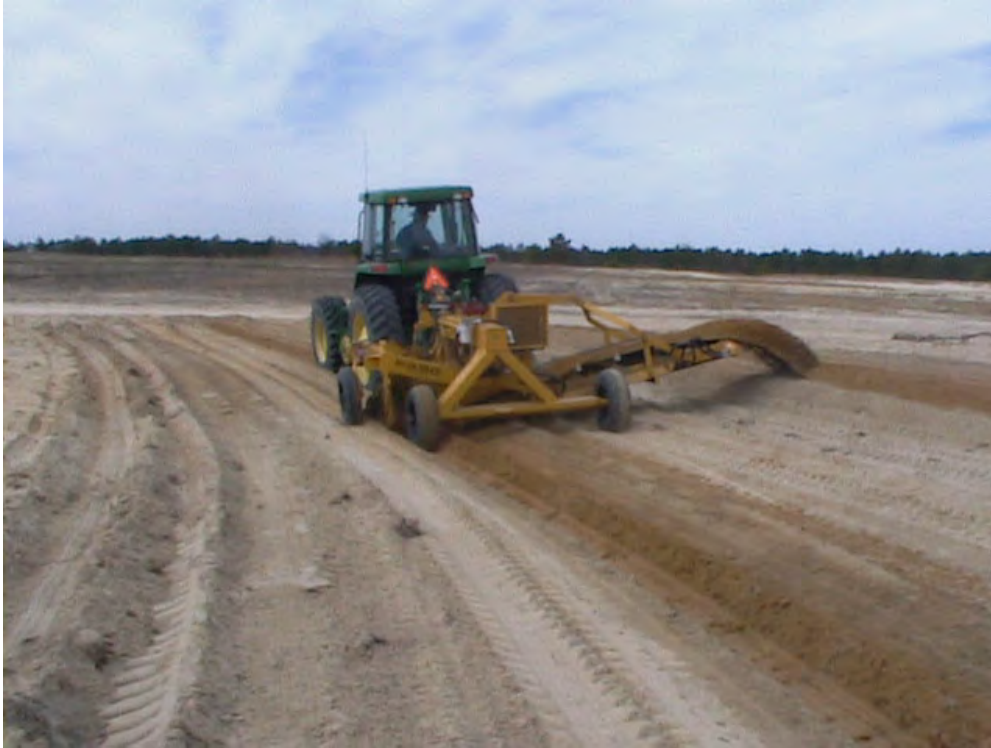
Figure C-15. Using in-house labor for terrace construction and seeding, Fort Bragg's revegetation costs have come down substantially compared with commercial contracting costs.
