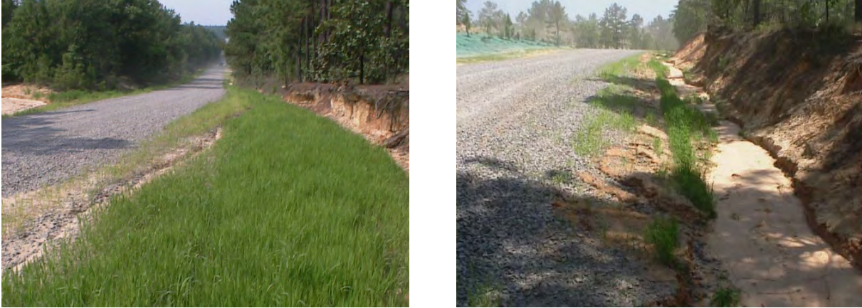
Figure C-18. McKellers Road – Adequate checkdams and in-time repairs would have prevented a complete washout.
