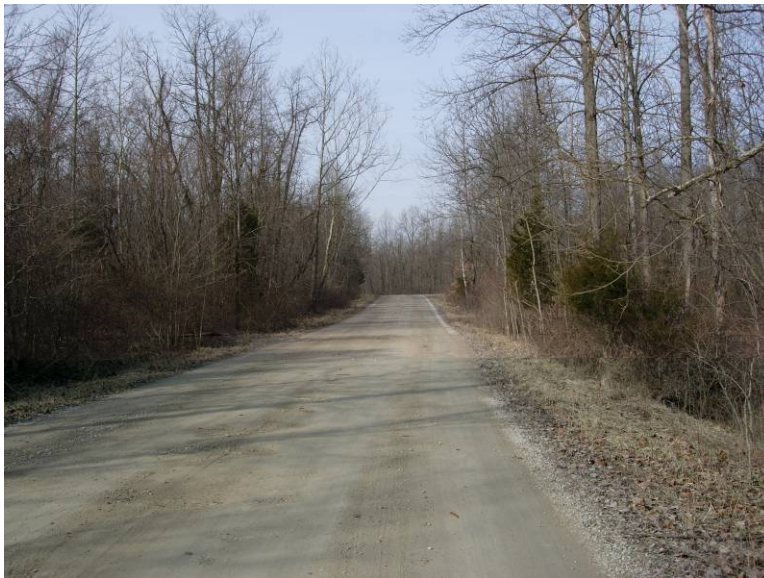
Figure B.4. Semi-improved road with moderate erosion at Camp Atterbury
