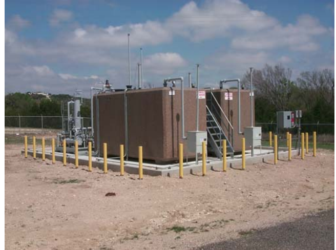
Fixed Fuel Filtration Unit
