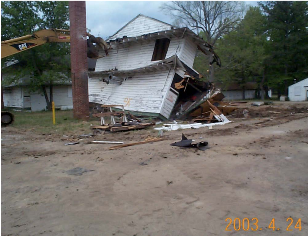
Figure B-6. Using a track hoe to tip remnant building shell after salvage at Fort McClellan in 2003 (Joyce Baird, ERDC-CERL).
