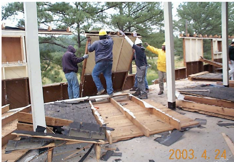
Figure B-3. Removing upper floor wall panels at Fort McClellan in 2003 (Joyce Baird, ERDC-CERL).
