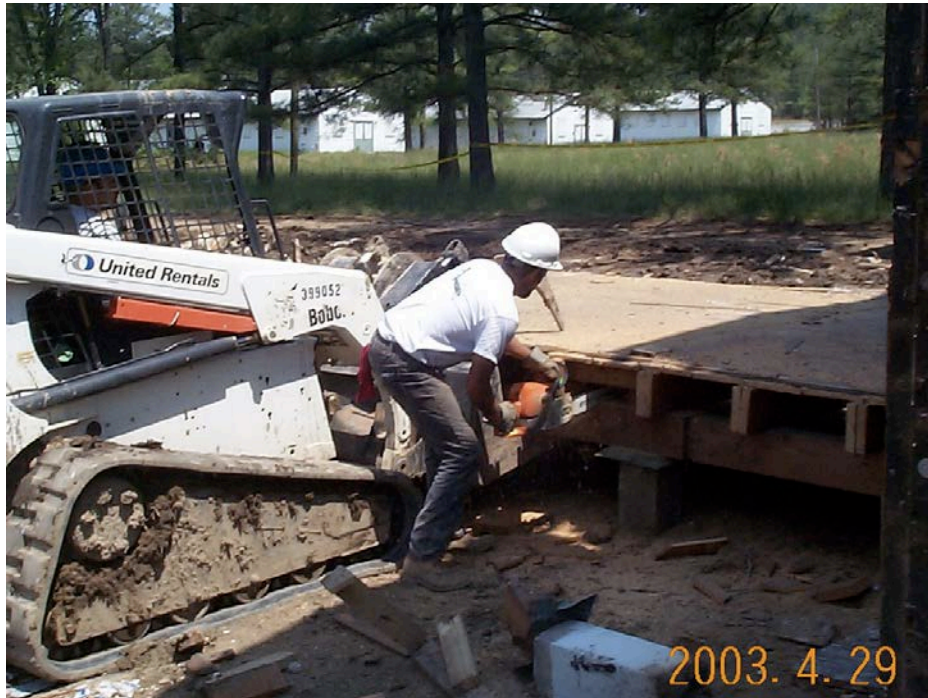
Figure B-4. Cutting floor panels at Fort McClellan in 2003 (Joyce Baird, ERDC-CERL).
