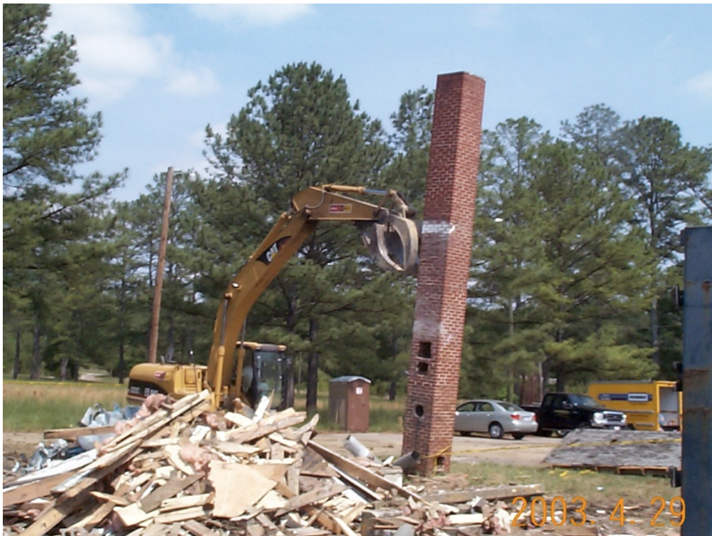
Figure B-7. Tipping chimney separately with track hoe to break apart bricks for potential recycling at Fort McClellan in 2003 (Joyce Baird, ERDC-CERL).
