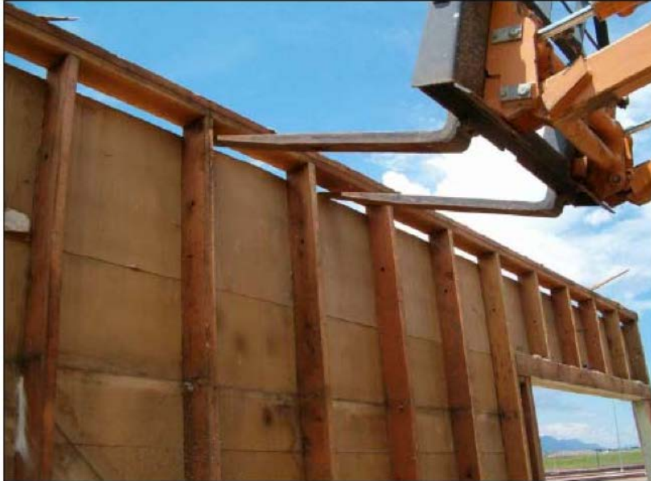
Figure B-13. Reach forklift removing exterior walls of Building 227 at Fort Carson (Innovar 2005).
