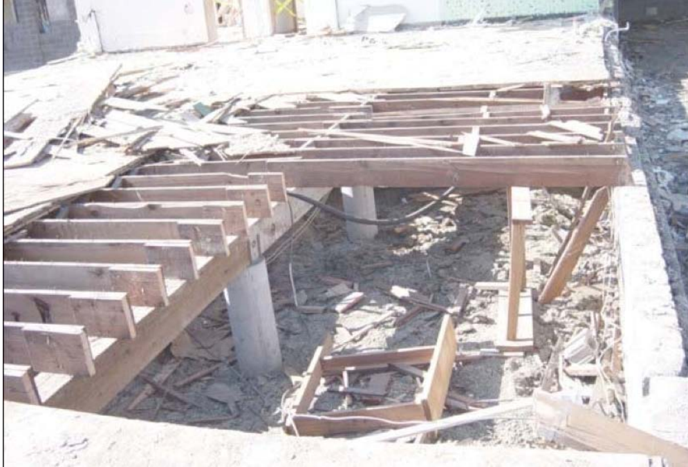
Figure B-11. Floor joist and concrete piers exposed during deconstruction of Building 6288 (Innovar 2005).
