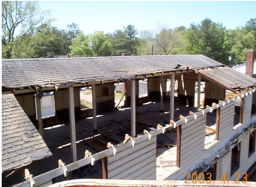
Figure B-2. Removing roof panels at Fort McClellan in 2003 (Joyce Baird, ERDC-CERL).
