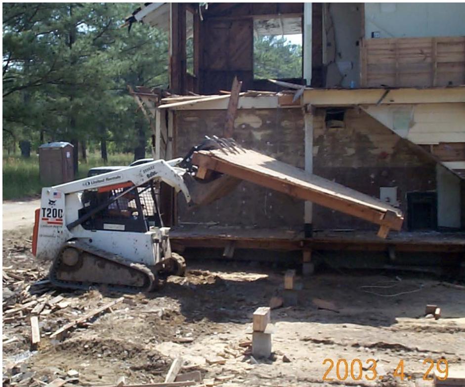
Figure B-5. Moving floor panels with skid steer at Fort McClellan in 2003 (Joyce Baird, ERDC-CERL).
