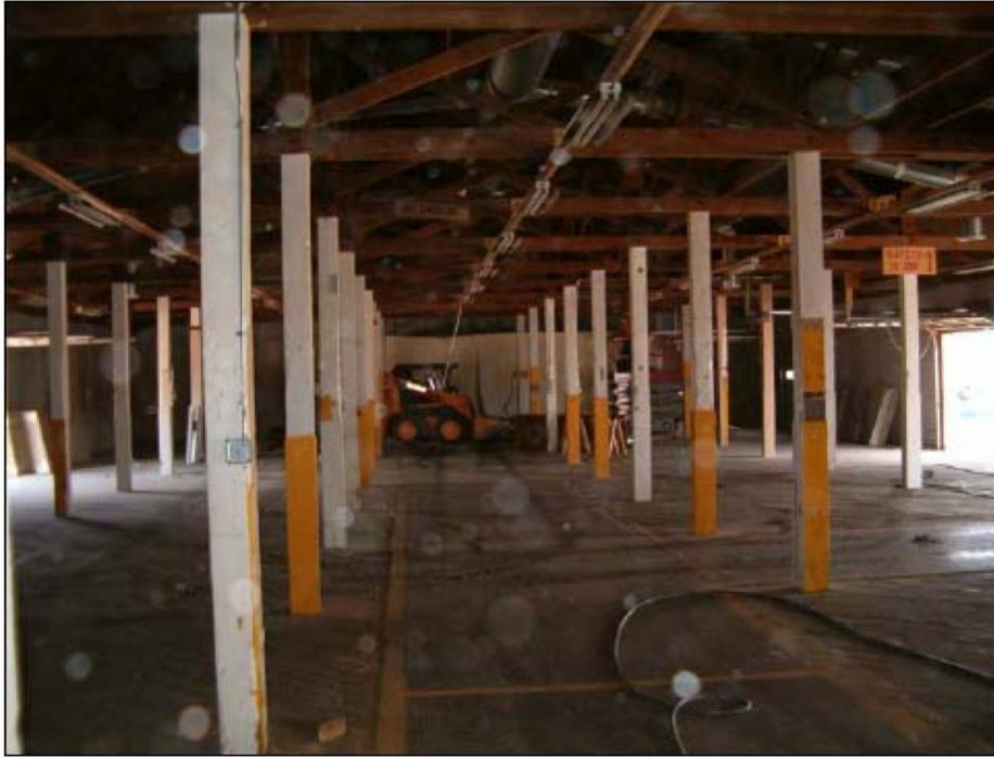
Figure B-12. Interior view of columns and roof structure in Building 227 at Fort Carson (Innovar 2005).
