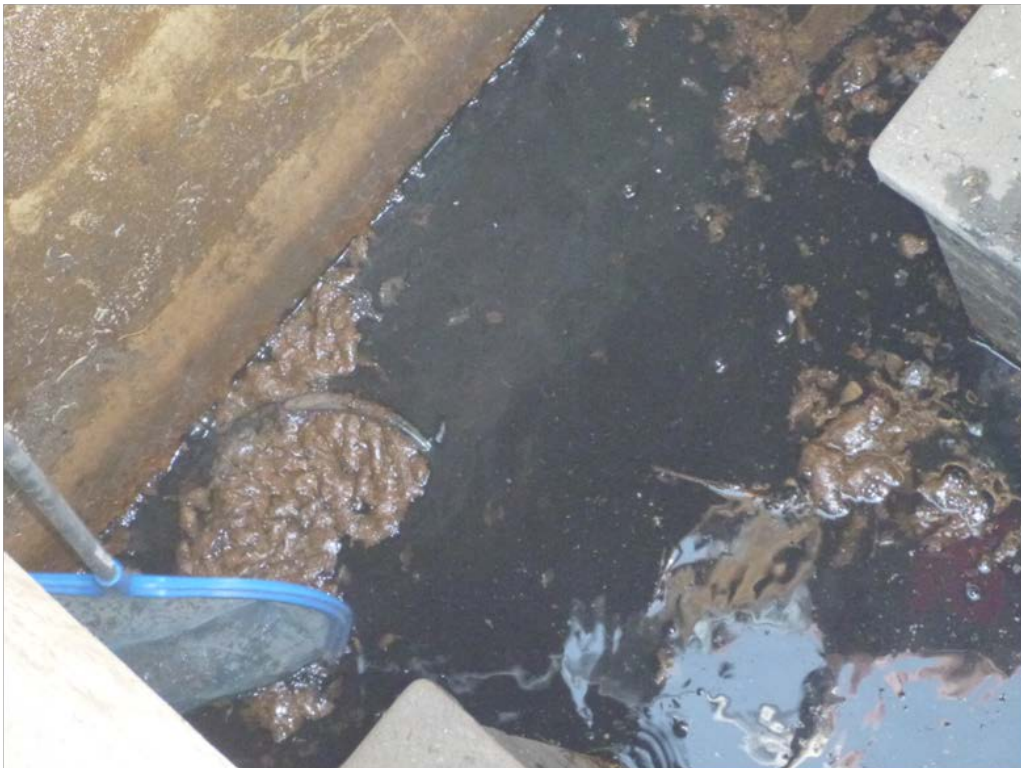
Figure B-24. Oil and algae growth in pre-treatment area.
