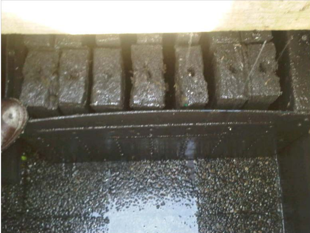
Figure B-23. Pre-treatment chamber.
