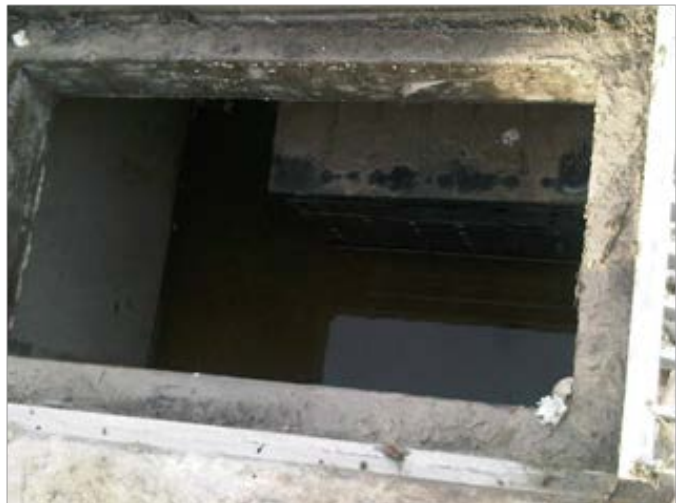
Figure B-22. Typical accumulation in settling area.
