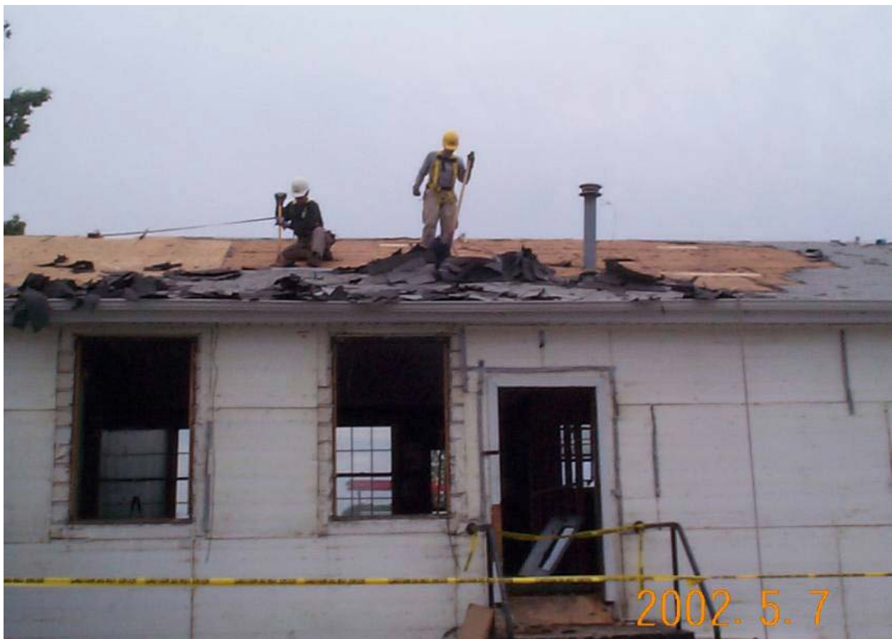
Figure C-1. Removal of asphalt shingles during deconstruction of a World War II-era Army barracks.
