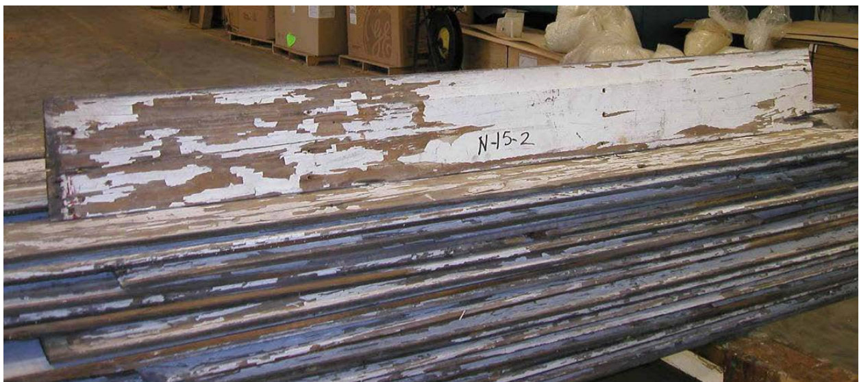
Figure D-4. Salvaged wood siding containing lead-based paint.
