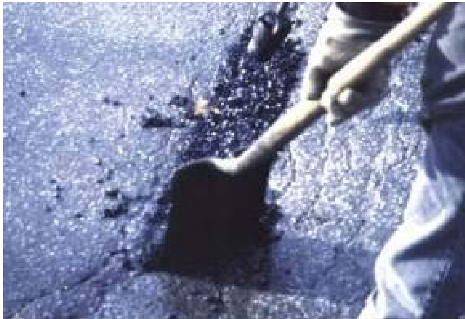
Figure C-5. Pot hole filled with cold-patch.
