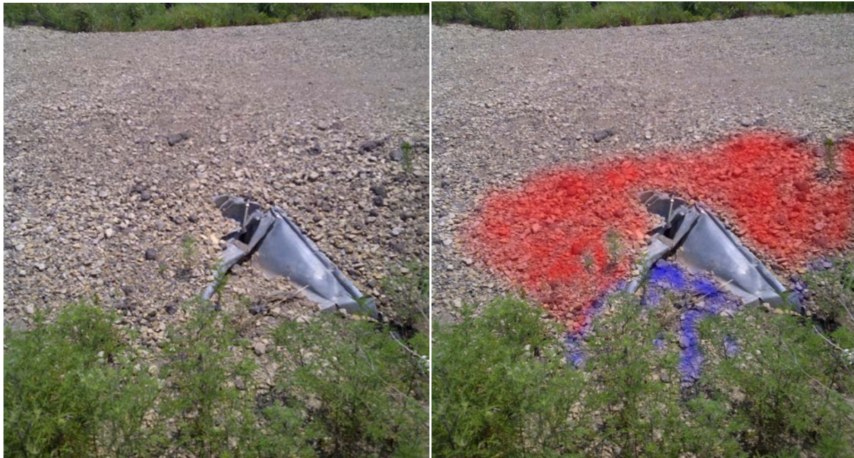
14 15 Figure C-3. Damaged culvert blocks subsurface water passage, causing water to 16 flow over the road. Subsequent erosion of gravel is indicated by larger rocks 17 remaining at the top and sides (red area), and smaller rocks being washed 18 into the depression (blue area) (ERDC-CERL).
