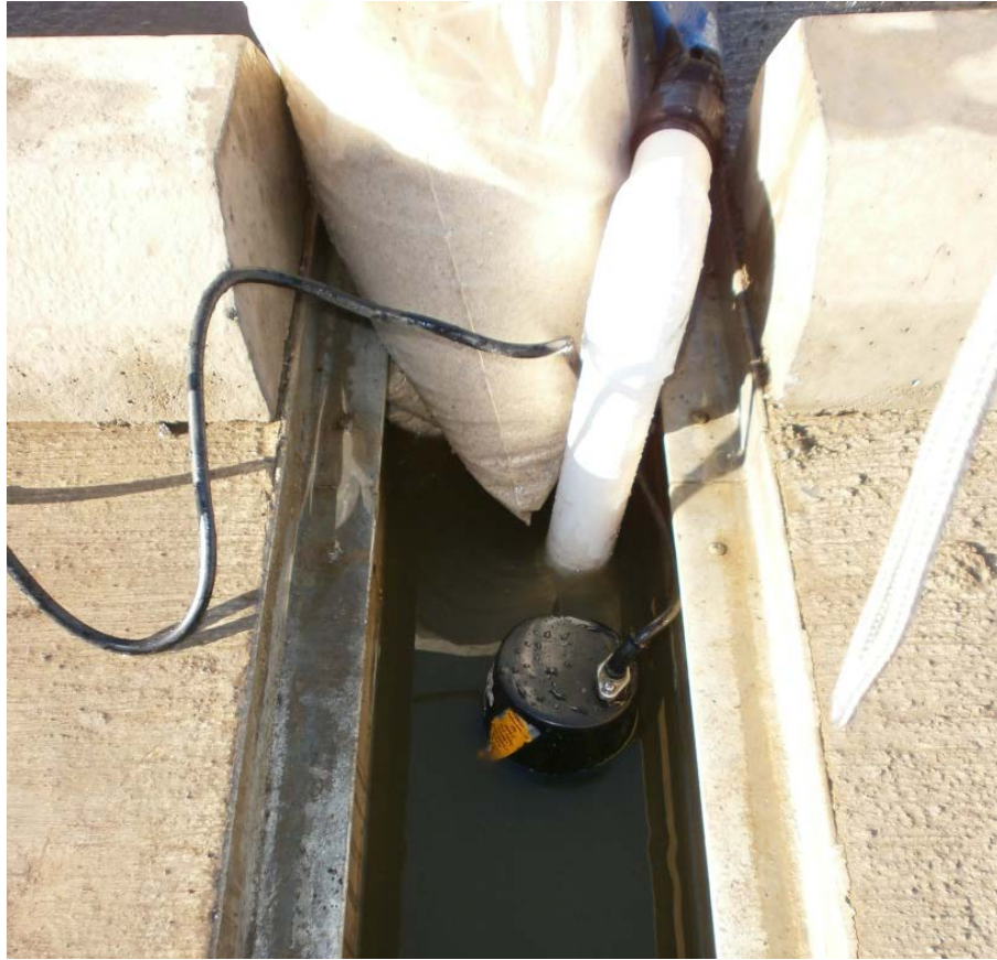
Figure B-8. Sump pump emerged in trough.
