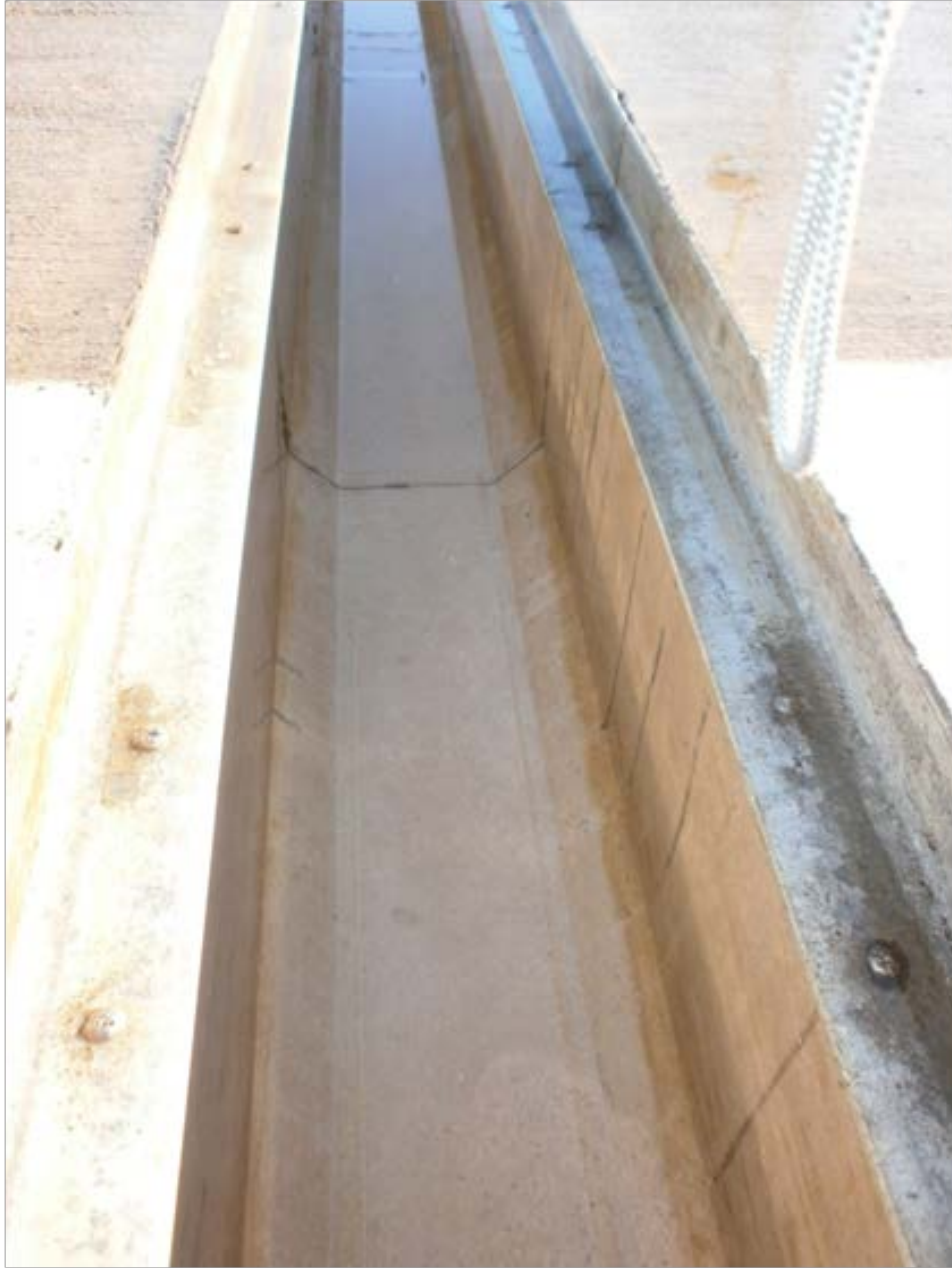
Figure B-5. Clean trough before washing.
