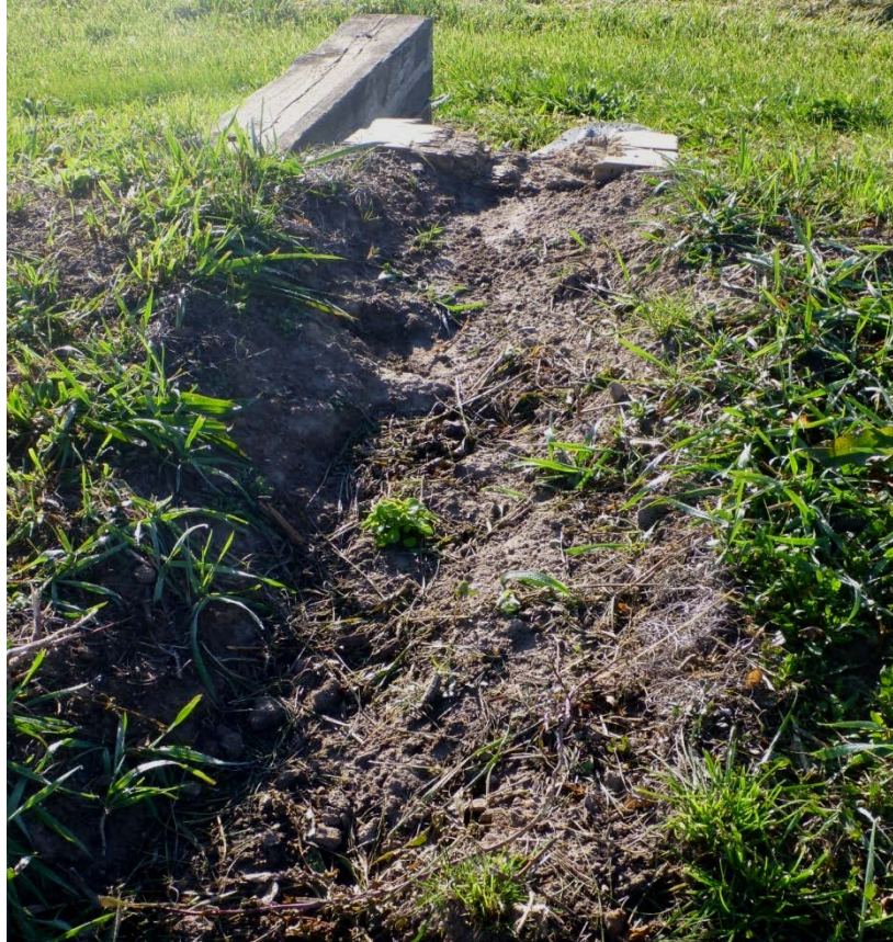
Figure B-4. Berm failure and timber beam damage (top of photo) resulting from projectile impacts at Camp Atterbury demonstration site (ERDC-CERL 2012).
