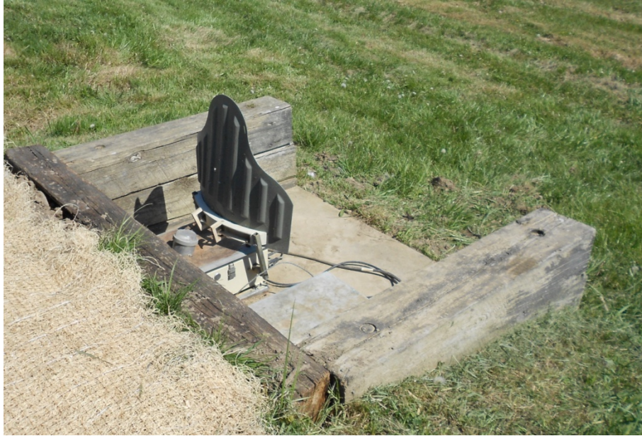
Figure B-2. A typical SIT emplacement with treated timber at Camp Atterbury demonstration site (ERDC-CERL 2012).
