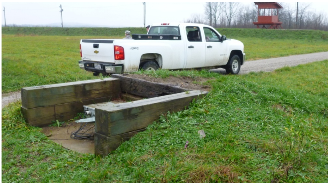
Figure B-1. A typical SIT emplacement berm at Camp Atterbury demonstration site (ERDC-CERL 2011).
