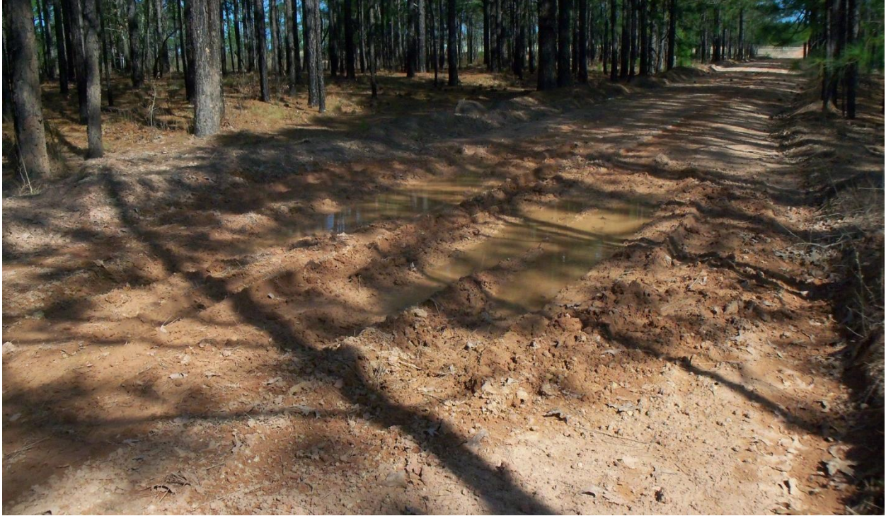
Figure B-9. Wet area on road develops when water accumulates in larger rills and gullies from being unable to run off the road (Phillips and Jordan).
