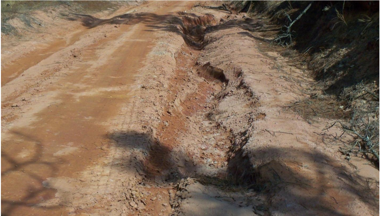
Figure B-7. Larger gully on side of road, formed as a result of water running down the road at higher velocity (Phillips and Jordan, Inc.).
