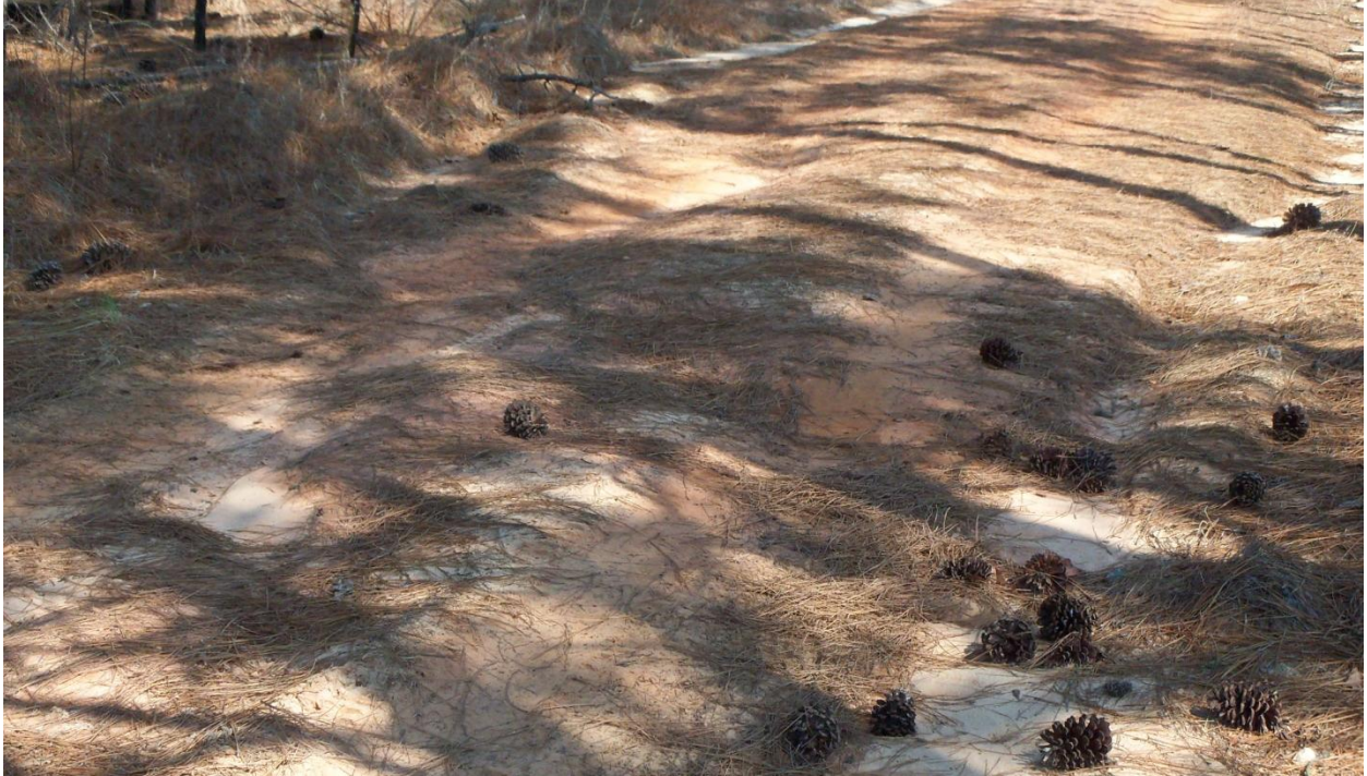
Figure B-5. Rills and small gullies forming along and in the road (Phillips and Jordan, Inc.).
