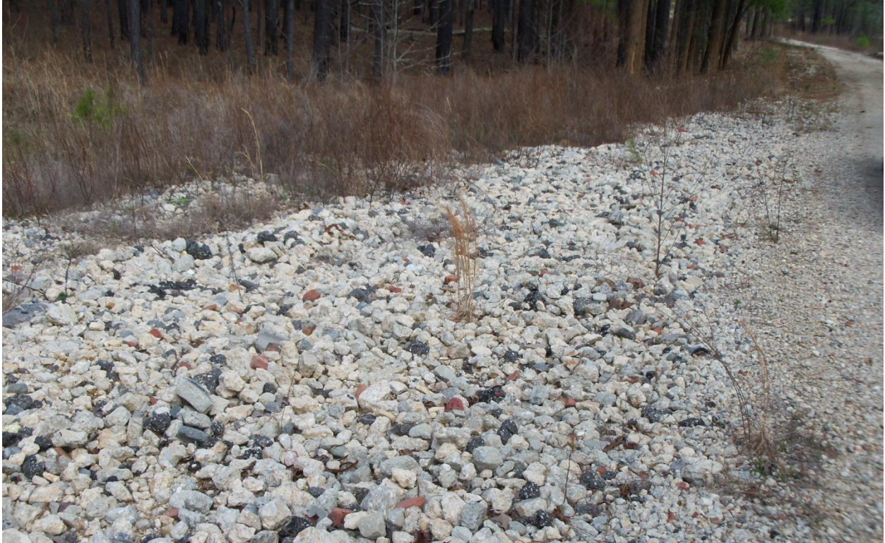
Figure B-15. Riprap along trail for erosion control (Phillips and Jordan, Inc.).
