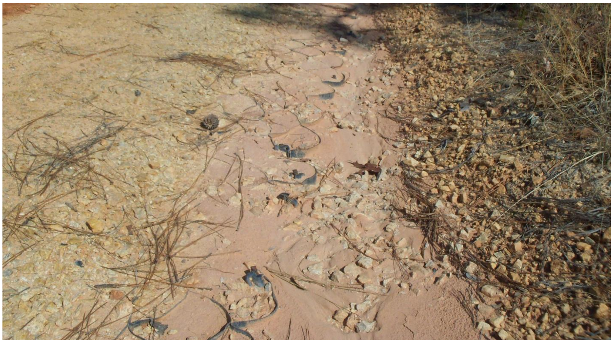
Figure B-18. Erosion control mat visible along road, showing there is little erosion except some fines leaving (Phillips and Jordan, Inc.).
