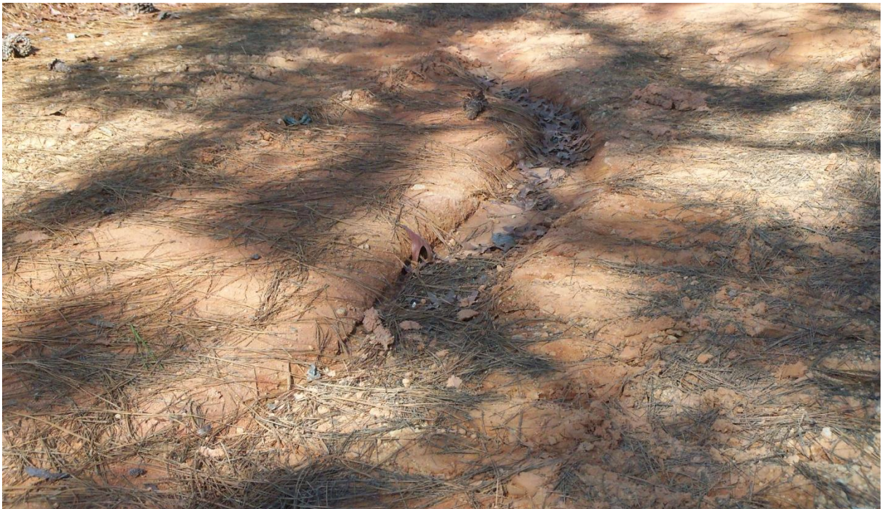
Figure B-6. Close-up of a rill in the road, which is deepening as water continues to be unable to get off the road (Phillips and Jordan, Inc.).
