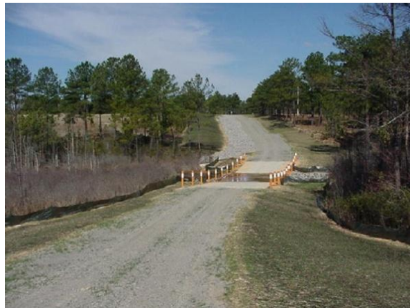
Figure C-5. Concrete stream crossing without adequate drainage (Phillips and Jordan).
