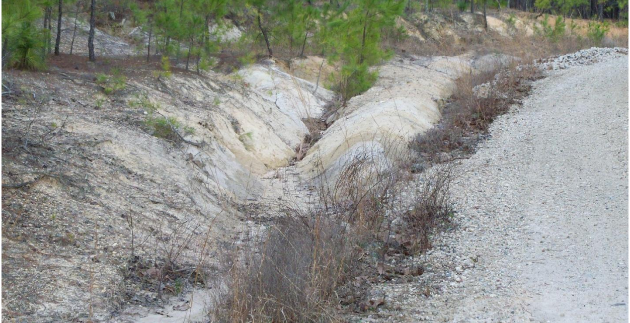
Figure B-11. Gully along road due to runoff from area adjacent to the road (Phillips and Jordan, Inc.).
