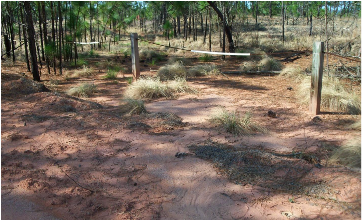
Figure B-10. Deposition of sediment along road, carried by gullies (Phillips and Jordan, Inc.).
