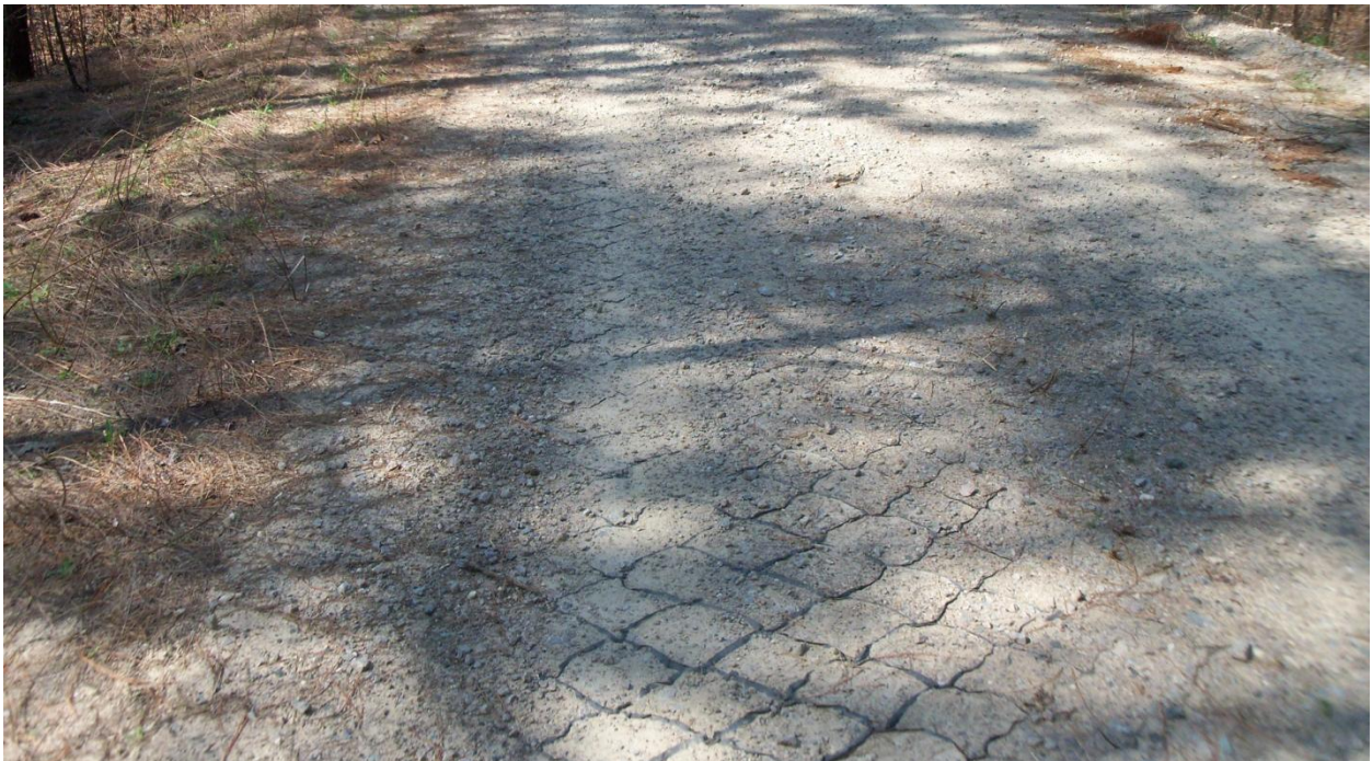
Figure B-16. Erosion control mat (Geoweb®) visible in road surface (Phillips and Jordan, Inc.).
