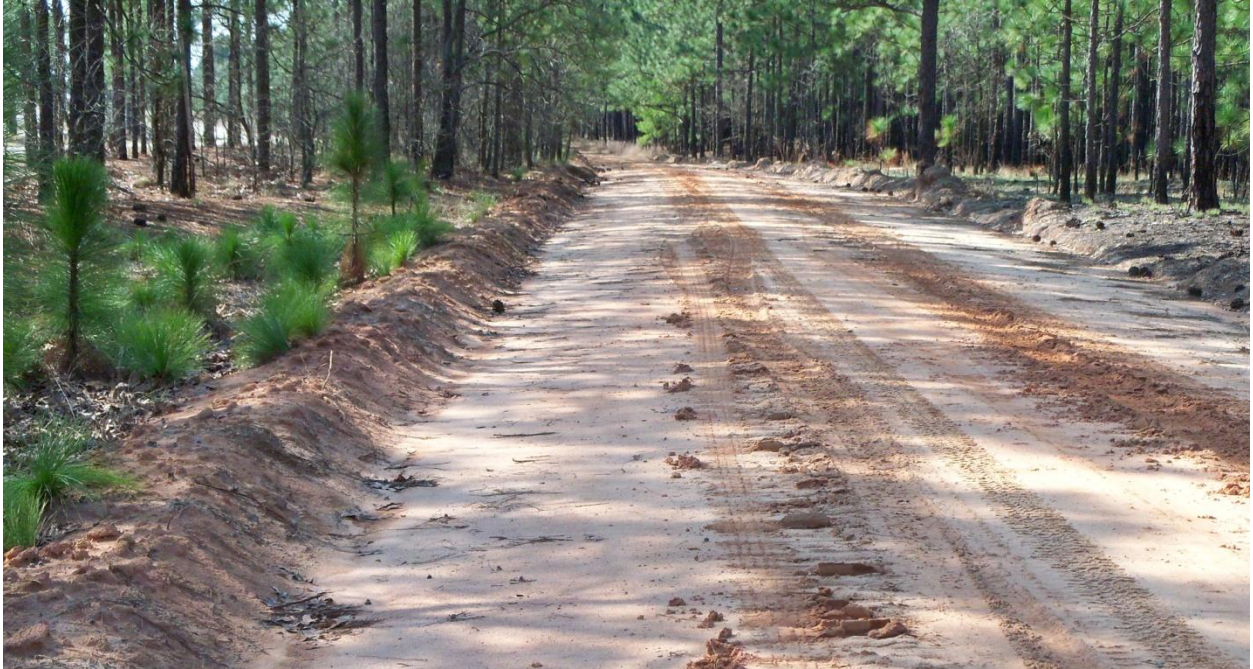
Figure B-3. Note ridges of soil along each side of the road that prevent water from running into forest. Ridges were formed as a result of grading (Phillips and Jordan, Inc.).
