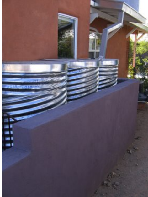
Figure C-54. Cistern system (photo courtesy of Technicians for Sustainability).
