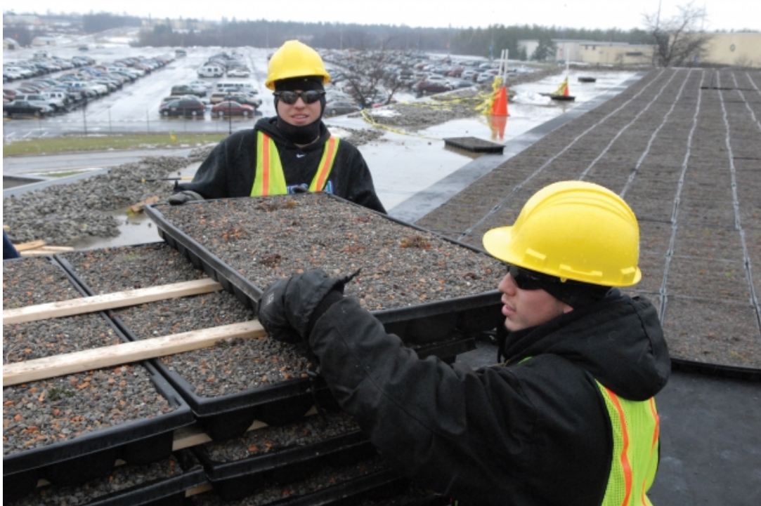
Figure C-24. Installation of a green roof on Building 11's Wing C at Fort Hood, TX (photo by Steve Grzedzinski).
