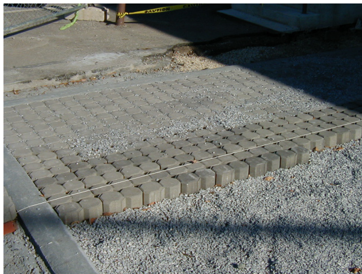
Figure C-36. Permeable pavers at Washington Navy Yard (Low Impact Development Center, Inc.).
