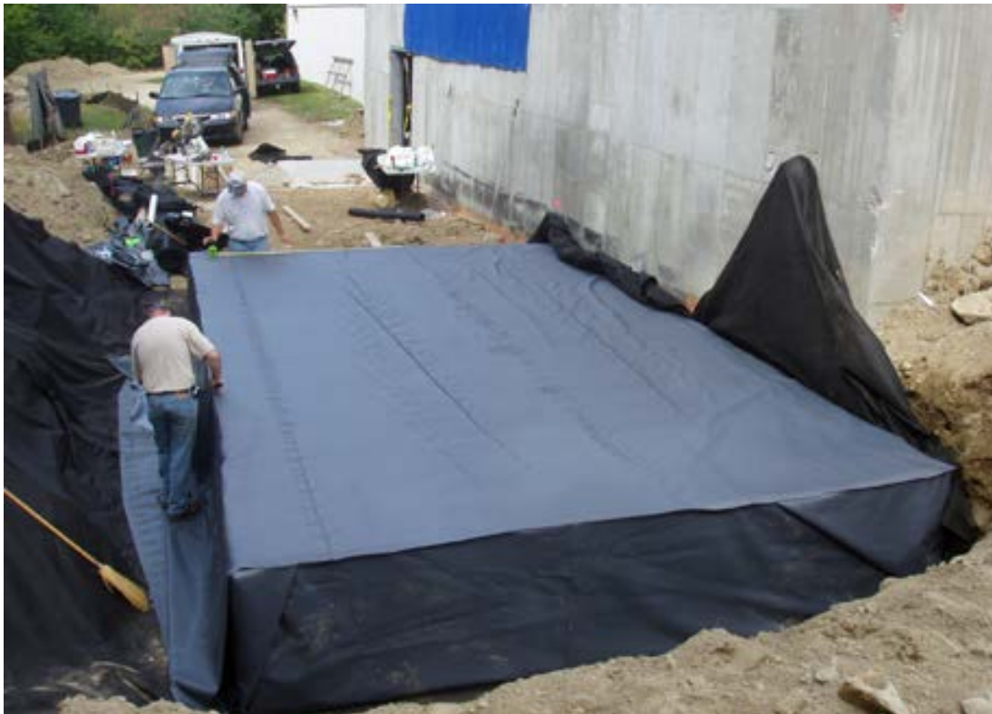
Figure C-57. Construction of a large underground cistern (photo courtesy of Rainwater Recovery Systems, LLC).
