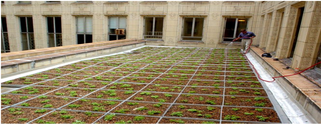
Figure C-30. Carnegie Mellon University green roof maintenance in Pittsburgh, PA (courtesy of Kelly Lockett).
