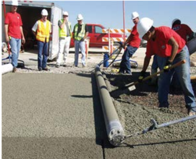
Figure C-44. Installation of pervious concrete using a Bunyan roller screed (photo courtesy of Dan Huffman, NRMCA).
