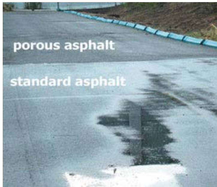
Figure C-47. Porous vs. standard asphalt after rain event (photo courtesy of Cahill Associates).
