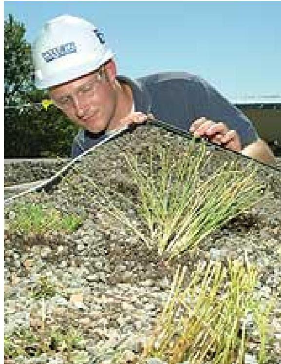
Figure C-23. Installation of a green roof on the Headquarters Building at Tobyhanna Army Depot, PA (photo by Steve Grzedzinski).
