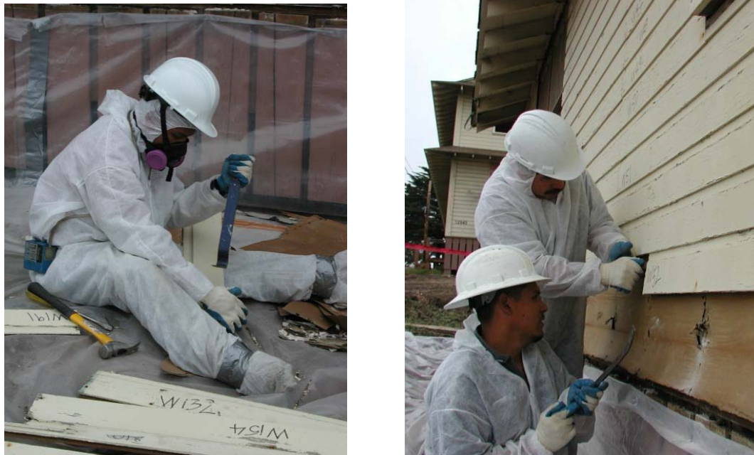
Figure A-12. Deconstruction workers during negative assessment (left, note personal air-monitor pump worn on belt) and following the negative assessment (right).
