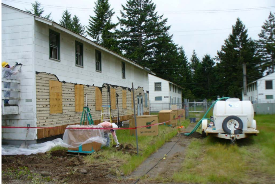
Figure A-9. Hazardous material removal (cement-asbestos siding), prior to deconstruction at Fort Lewis.
