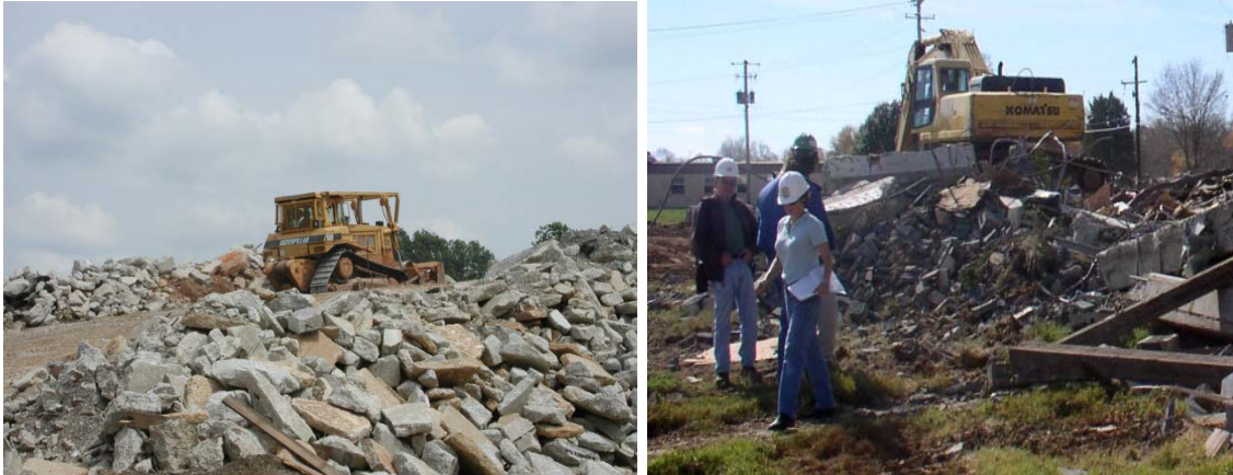
Figure A-17. Clean (left) and comingled (right) concrete rubble (Photo on the right by Wilmot Associates).
