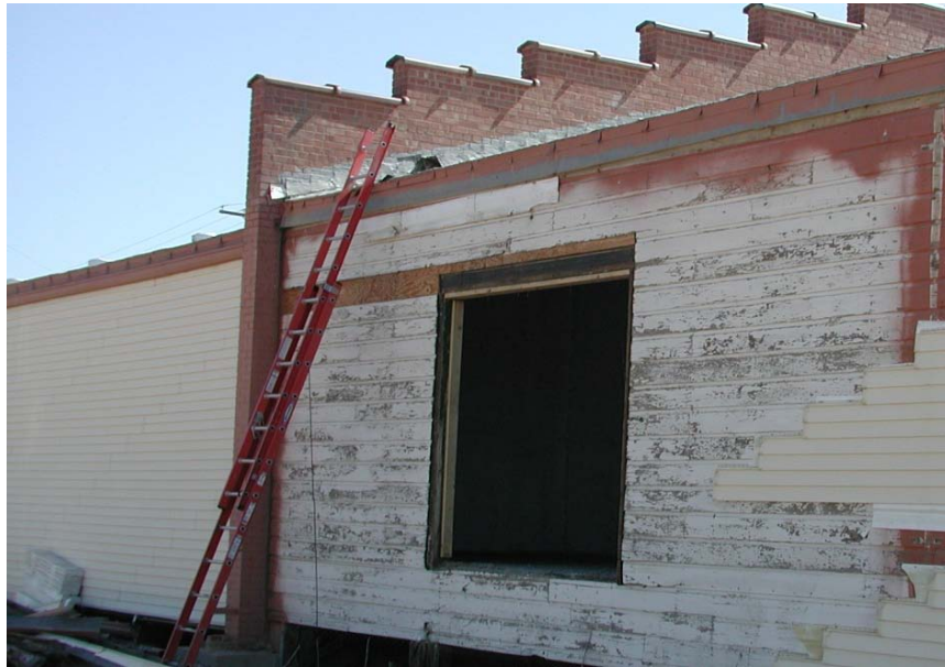
Figure A-10. Exterior siding painted with lead based paint at Fort Carson.
