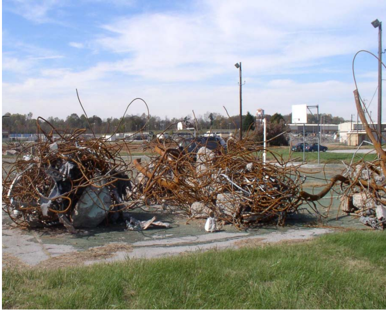
Figure A-22. Tangled reinforcing bar that resulted from improper sizing of concrete debris prior to recycling and under-capacity equipment selected by the contractor (Photo by Wilmot Associates).
