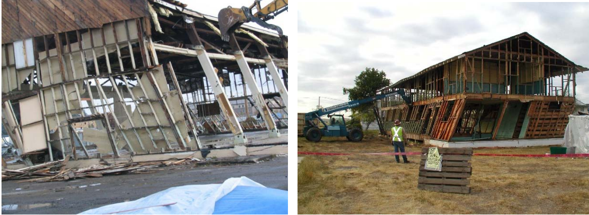
Figure A-33. Tipping a physical fitness center at Fort Lewis and a barracks at Camp Roberts for on-the-ground disassembly.
