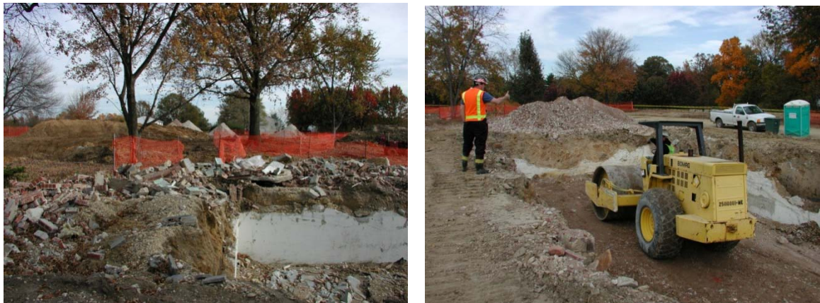
Figure A-18. Mixed brick and concrete rubble (left) recycled into engineered fill (right) at Andrews AFB.
