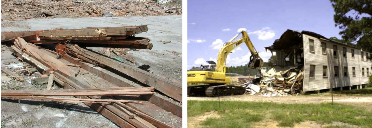
Figure A-30. Solid 12-in. x 18-in. x 24-ft Douglas Fir columns destroyed by wrecking at Fort Ord (left) and FRP demolition at Fort Polk (right)(Photo on the right is by USACE Huntsville Engineering Support Center).
