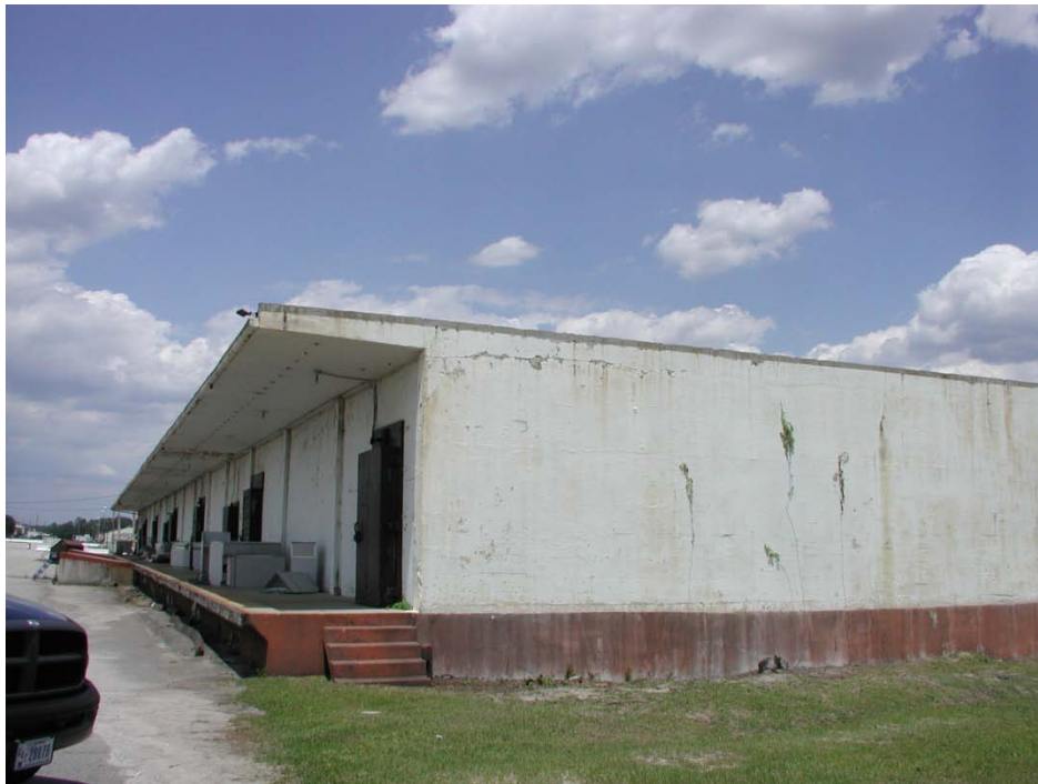
Figure A-13. Reinforced concrete building painted with lead-based paint at Fort Jackson.
