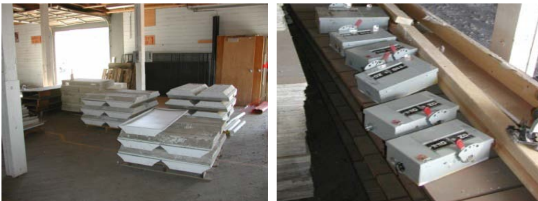
Figure A-6. Electrical components recovered for reuse from buildings at Fort Carson.
