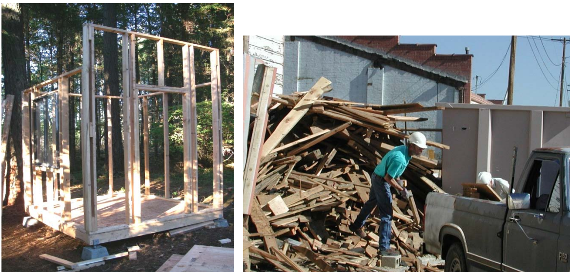
Figure A-34. Deconstruction lumber used for troop construction training at Fort Lewis (left) and deconstruction scrap wood offered to Fort Carson personnel.
