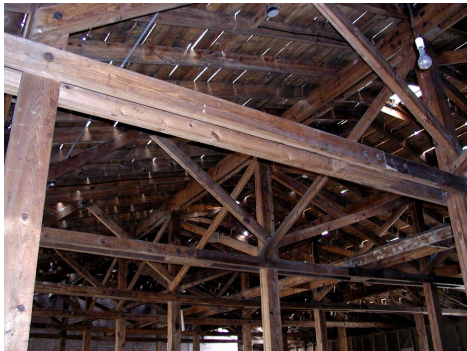
Figure A-11. Unpainted framing lumber at Fort Campbell (above) and Fort Gordon (below).
