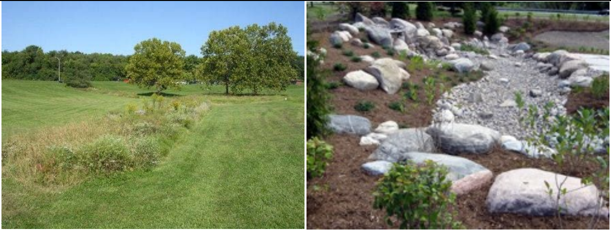
Figure H-60. Left: Vegetative Swale (Unified Government of Wyandotte County and Kansas City 2011); Right: Dry stone swale (ISMP 2010).
