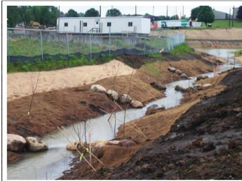
Figure H-48. Watercourse restoration utilizing bioengineering (Bioengineering Group, Inc., University of Iowa Stormwater & Bioengineering Design n.d.).
