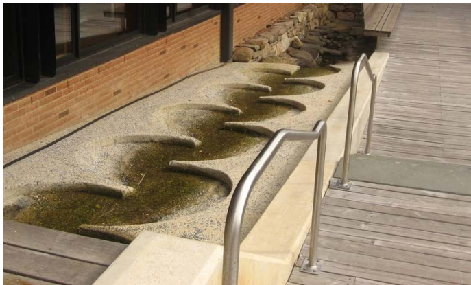
Figure H-29. A sculpted gutter feature along a walkway to convey stormwater (EPA 2008g).
