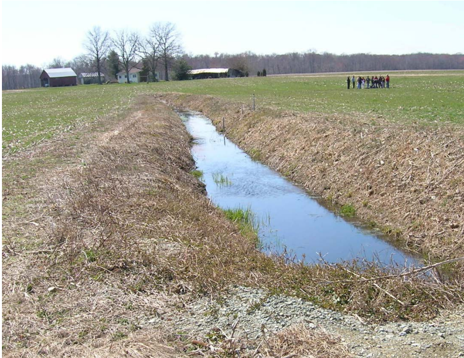
Figure H-2. Drainage ditch in an agricultural field near Ruthsburg, Maryland (Wicks 2008).
