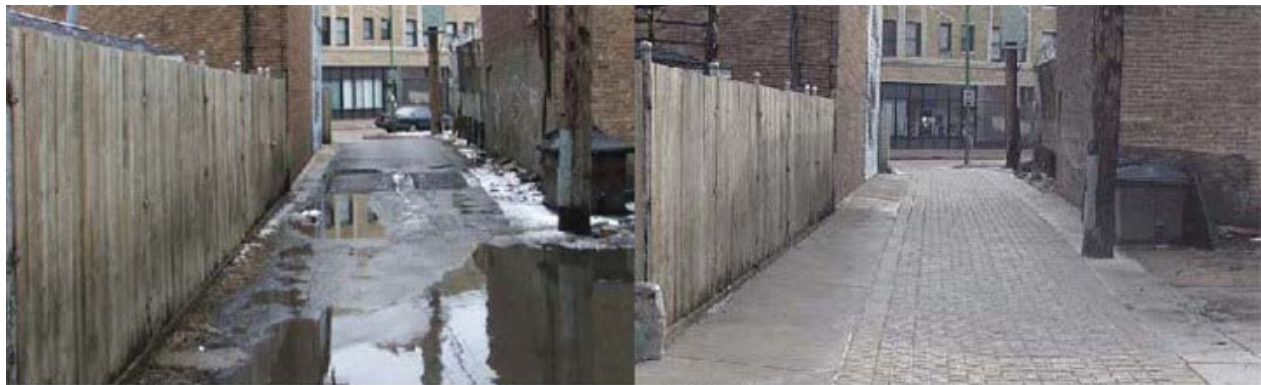
BEFORE: Alley with impermeable pavement and poor drainage
