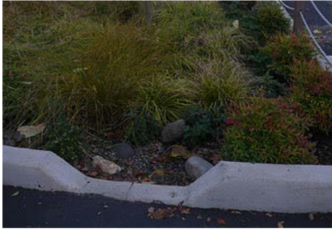
Figure H-38. Curb cut from paved area, allowing water to run off into vegetated areas (EPA 2008a).
