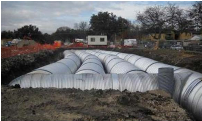
Figure H-16. Stormwater detention / infiltration system utilizing corrugated metal (Contech Construction Inc. 2011).
