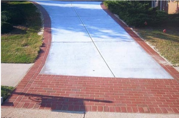
Figure H-43. Cast-in place concrete, stamped with a brick pattern and dyed red (Professional Concrete 2010).
