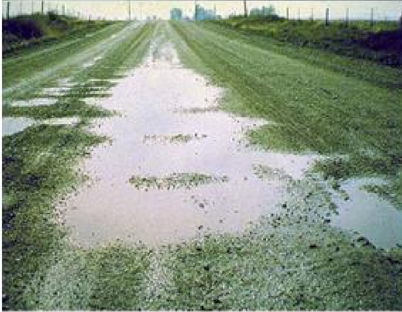
Figure A-10. Water quickly collects when the road crown is lost.
