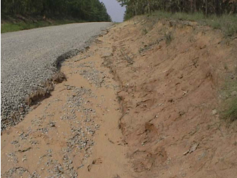
Figure A-3. Shoulder erosion is the most frequent source of degradation to dirt and gravel roads on Army lands.
