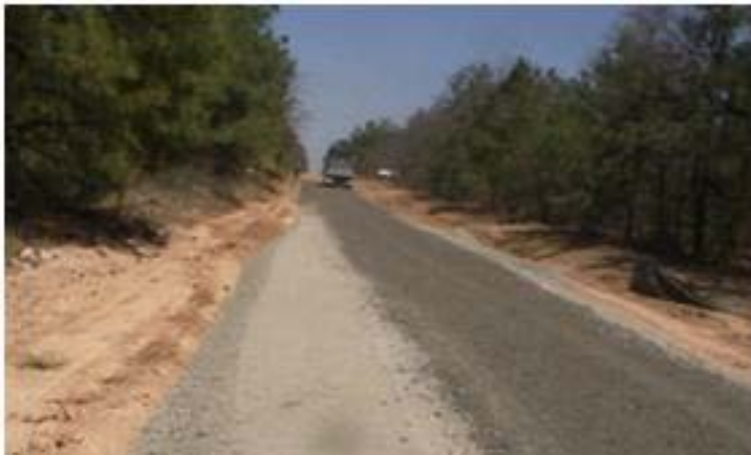
Figure A-1. Addition of aggregate to earthen surfaces improves road stability and durability.
