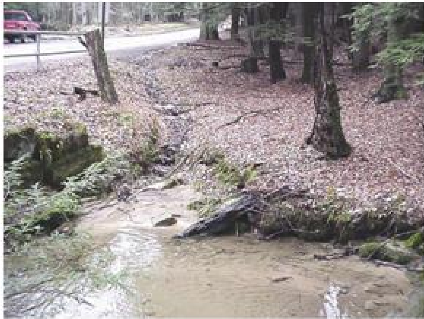
Figure A-5. Military roads can be sources of uncontrolled drainage from topographic high spots.
