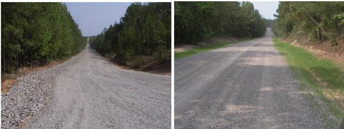
Figure A-13. Riprap and grass-lined ditches along road shoulders can provide good drainage.
