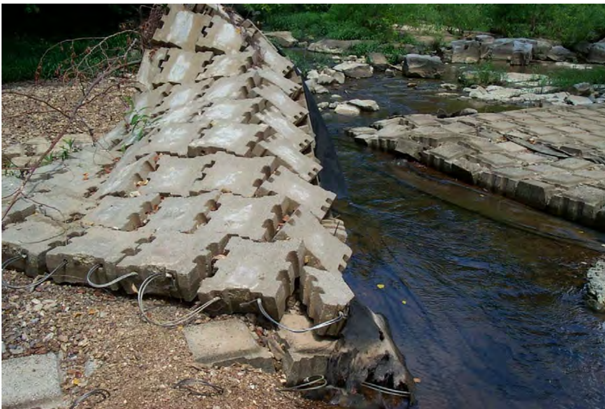
Figure C-5. Articulated concrete was not sufficiently anchored (photo by Chris Collins, Fort Campbell, KY).
