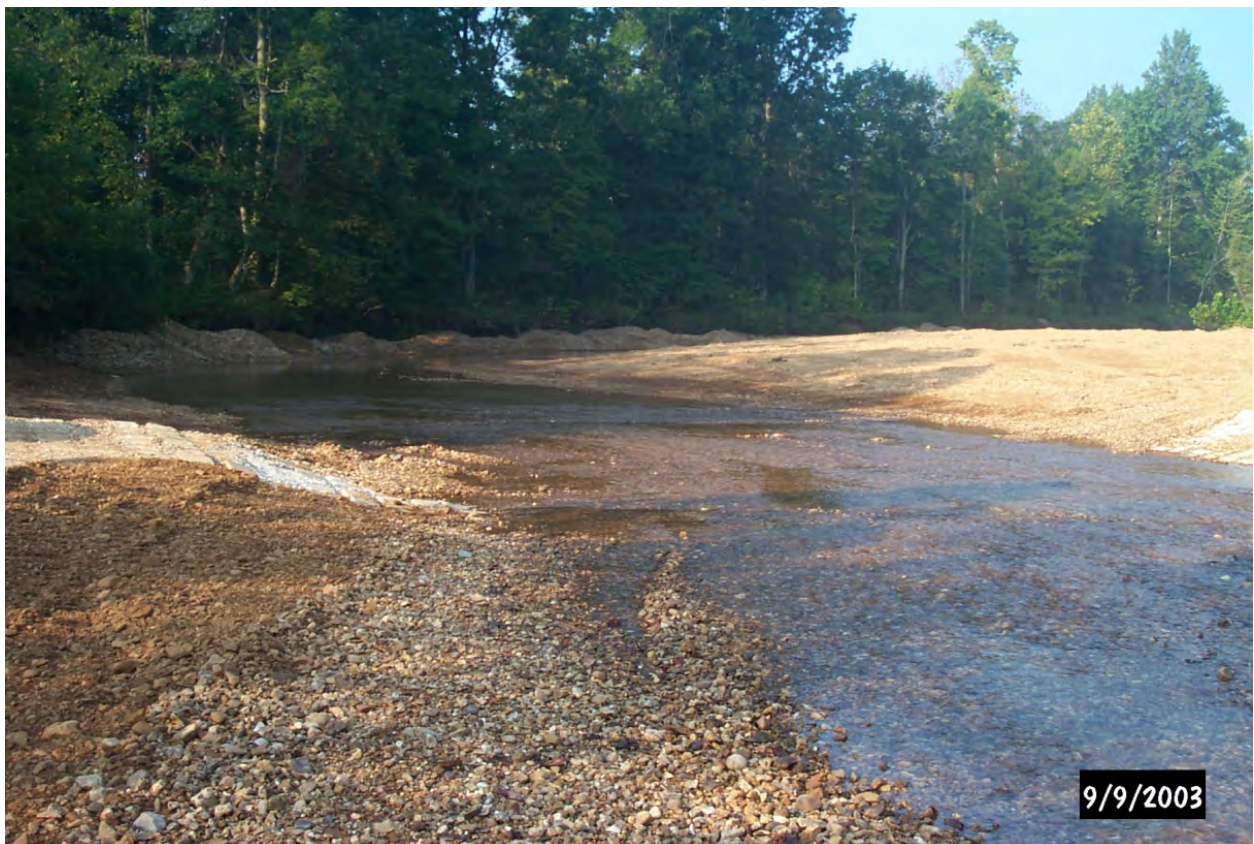
Figure A-1. This completed articulated concrete crossing is an example of an unvented ford (photo by Chris Collins, Fort Campbell, KY).
