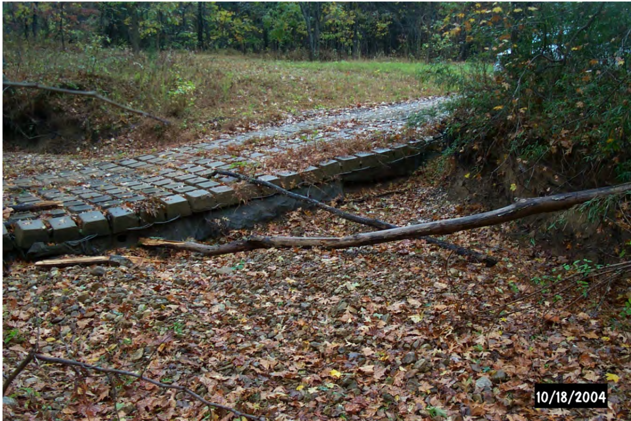
Figure C-3. Scouring has occurred on downstream edge of crossing (photo by Chris Collins, Fort Campbell, KY).
