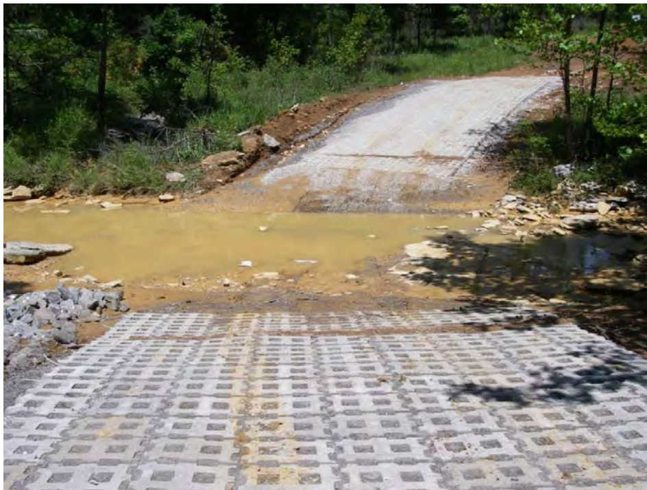
Figure C-7. Interlocking blocks on approaches (photo by Scot Serafin, Fort Knox, KY).
