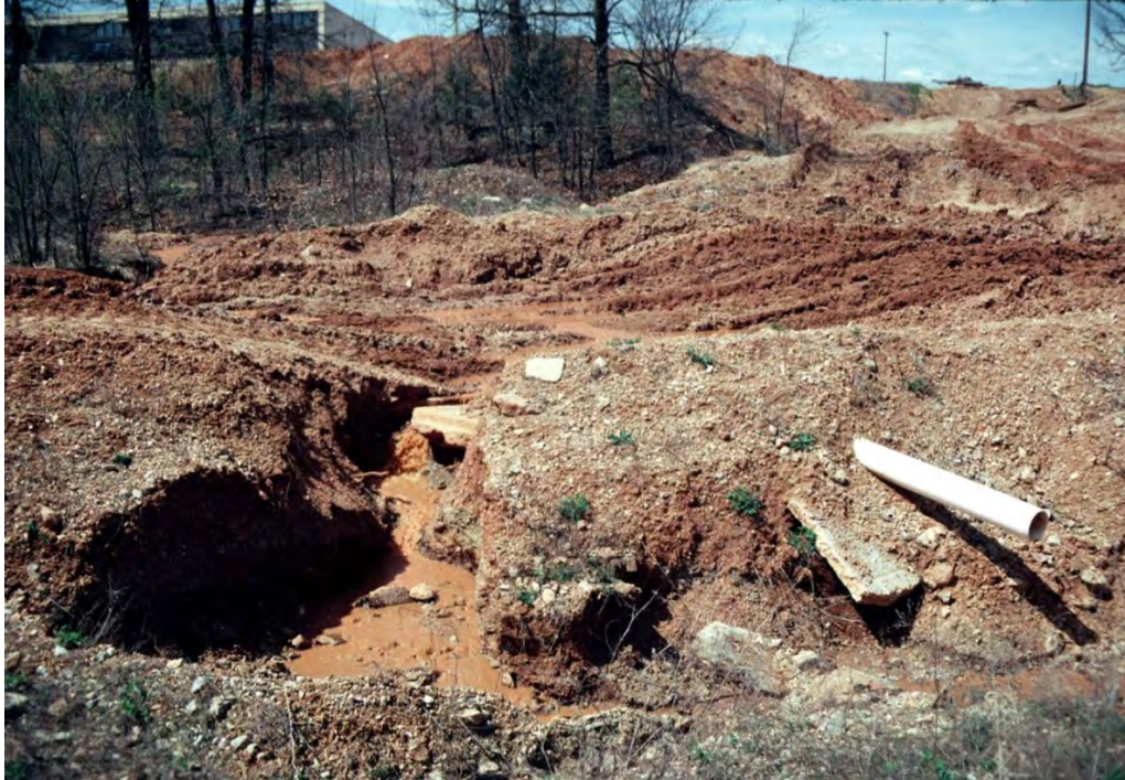
Figure C-1. Crossing before improvement showing blown culvert, erosion, and scouring of an improperly sited and designed crossing (photo by Joe Proffitt, Fort Leonard Wood, MO).
