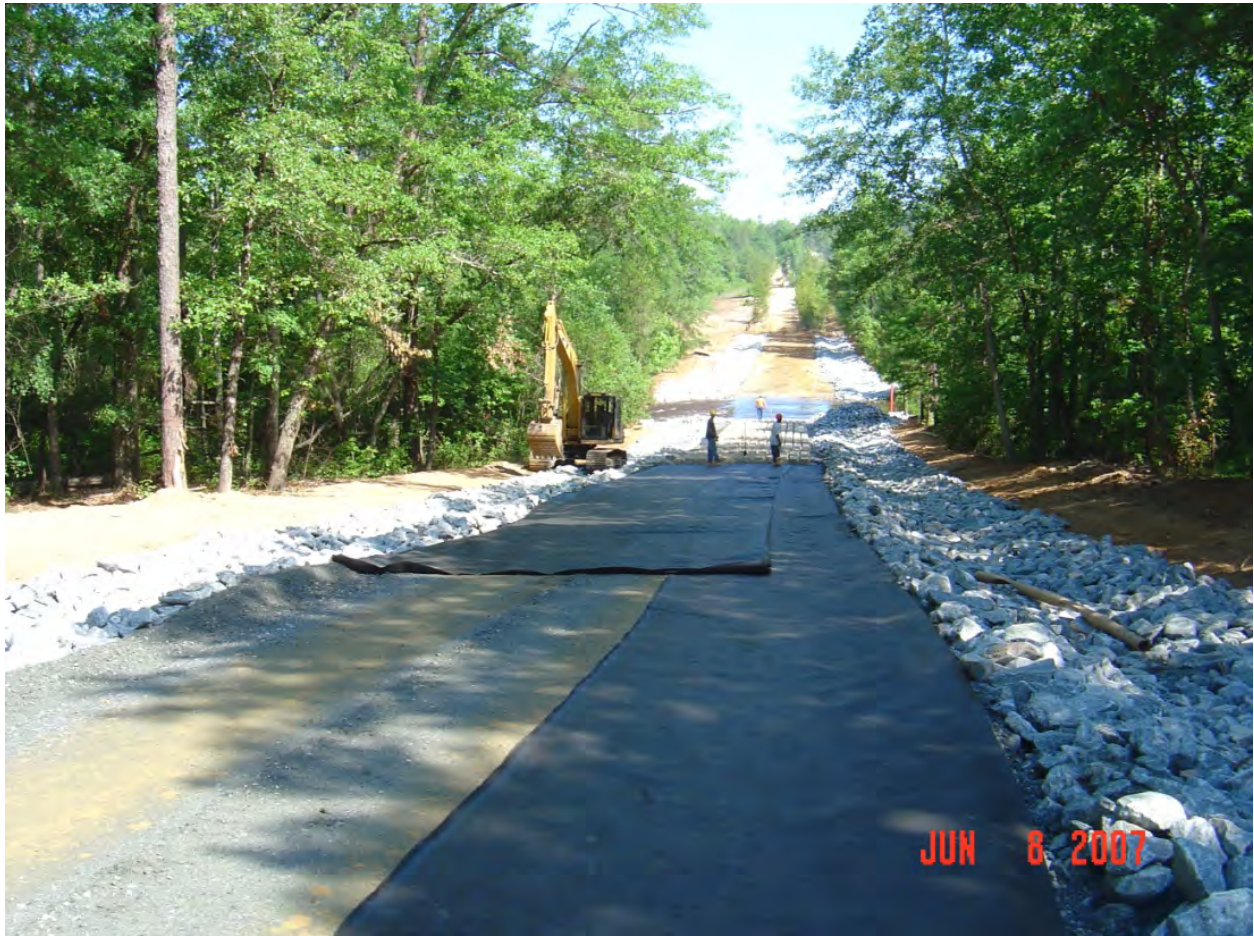
Figure C-4. LWC installation with rip rap used in ditches to prevent erosion (photo by Johnny Markham, Fort Benning, GA).
