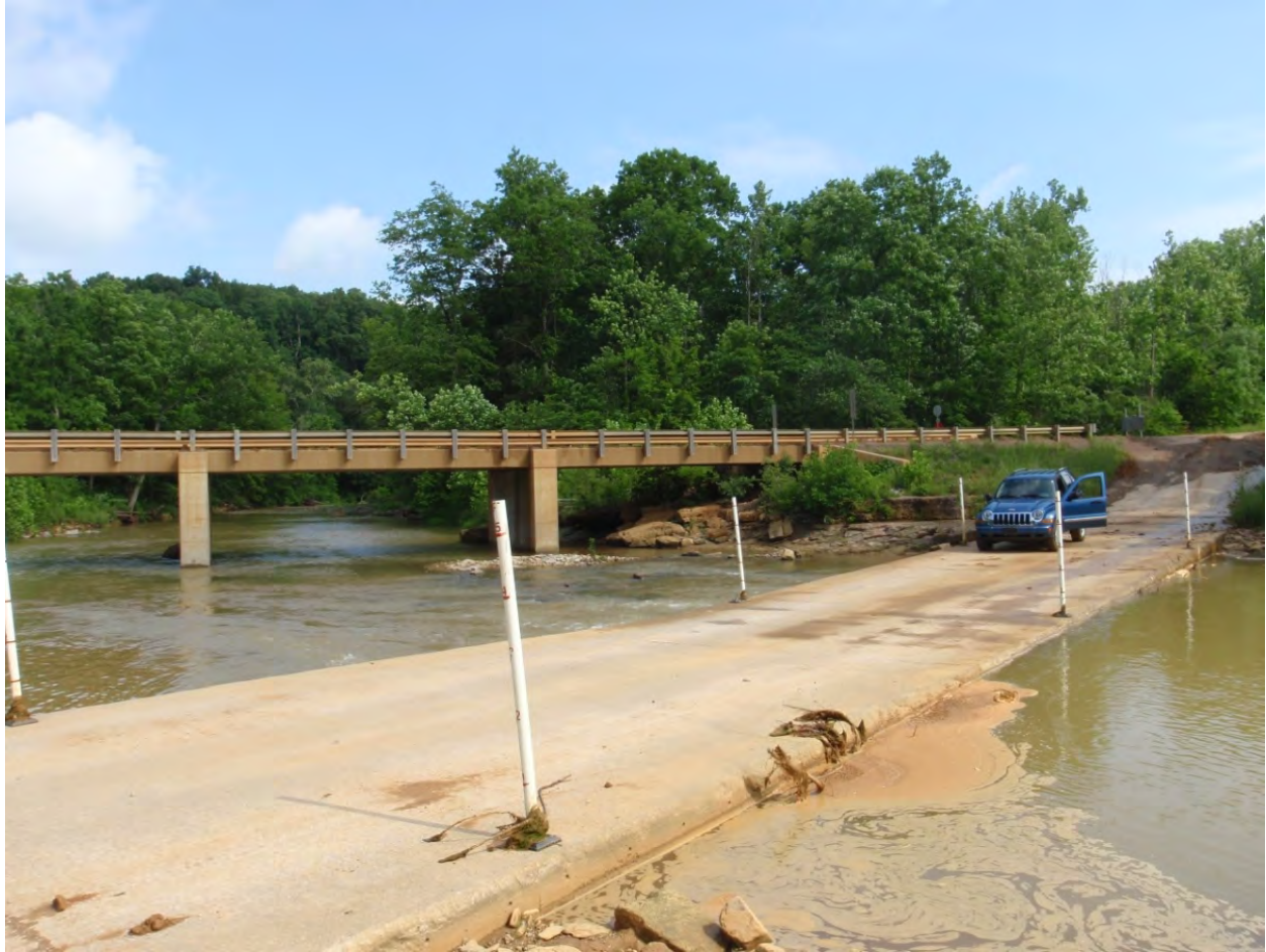
Figure B-1. Low-water crossing situated next to bridge. (Photo by Scot Serafin, Fort Knox)
