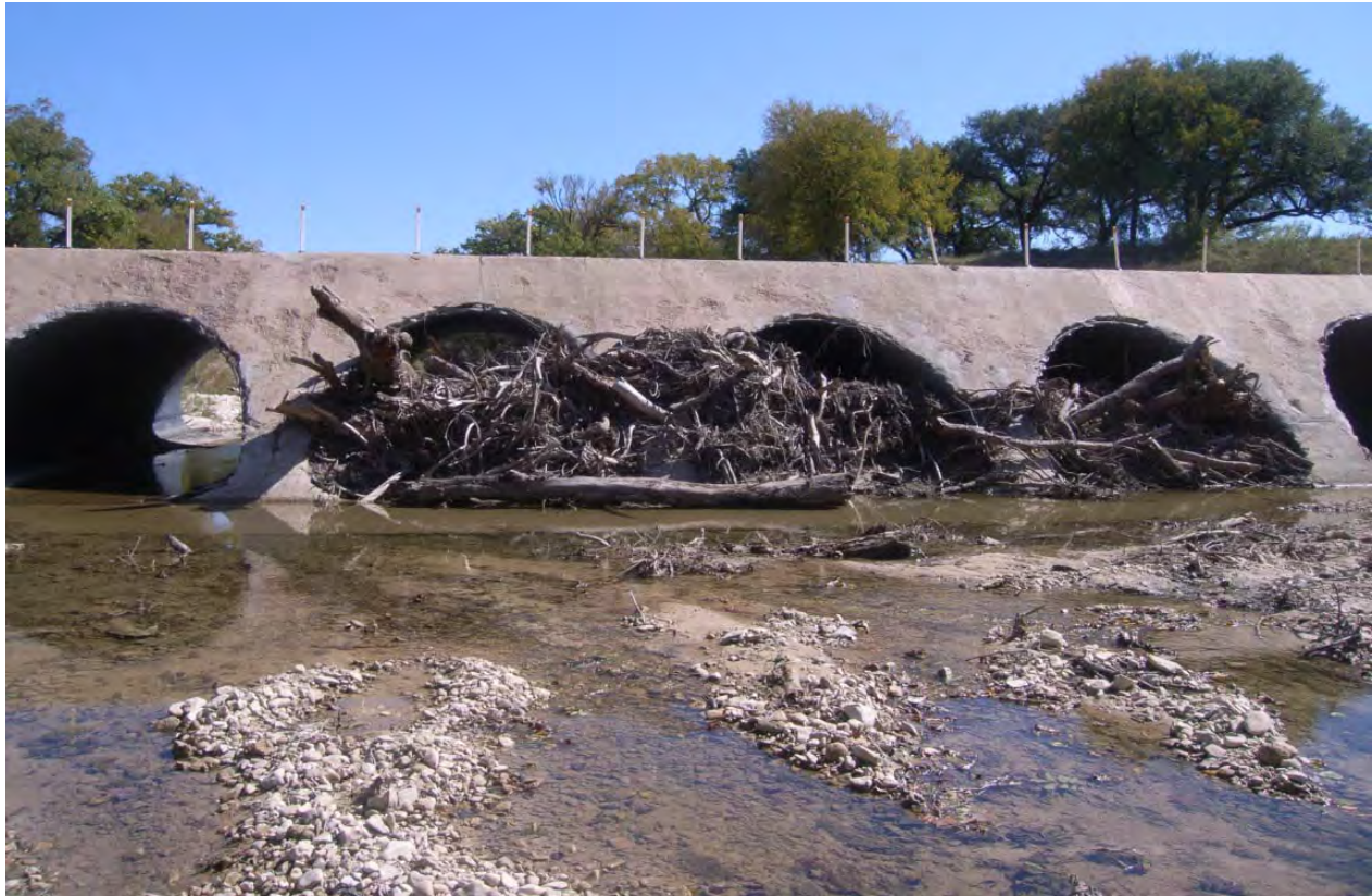
Figure C-8. Large, plugged culverts (photo by Jerry Paruzinski, Fort Hood, TX) .
