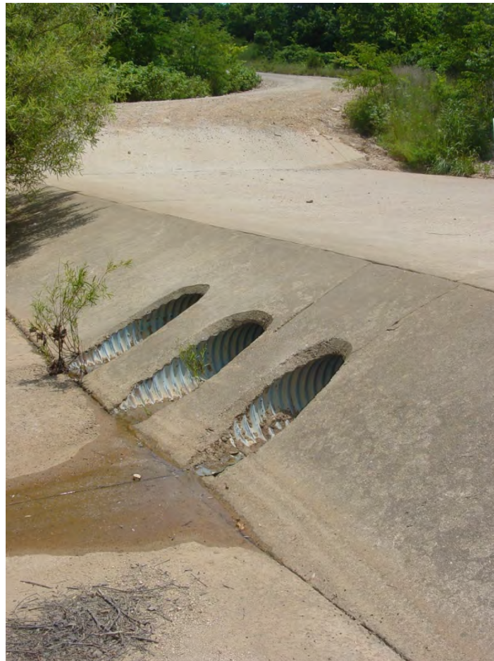
Figure A-2. Vented low-water crossing (photo by Joe Proffitt, Fort Leonard Wood, MO).
