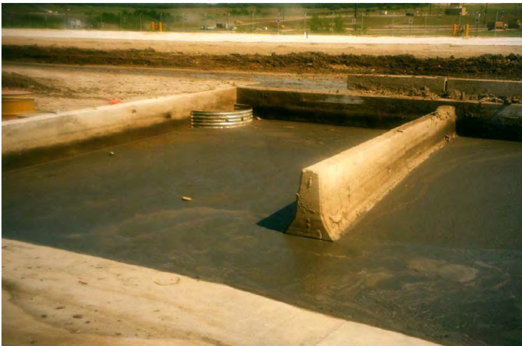
Figure B-1. Grit collection chamber.
