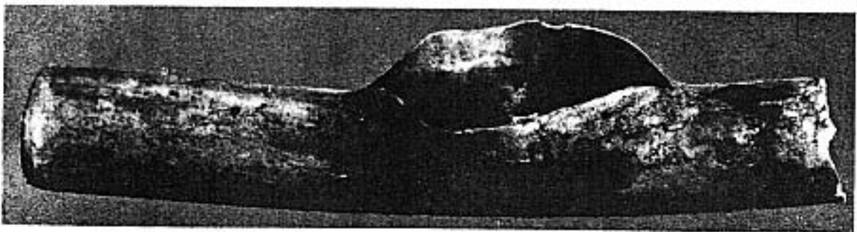
FIGURE 4-2. BOILER TUBE FAILURE CAUSED BY SCALE
