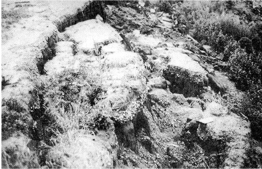
Figure 7-6. Slide failure or collapses of a steep slope.
