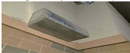
Image 11-2 EIFS Hood Termination Sealed (Winter)
