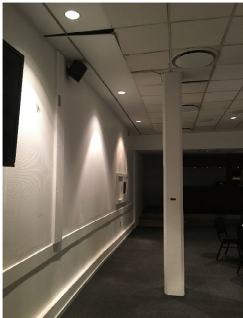
Figure 5-2. Left: A photo of a meeting room at a site in Thule, Greenland, where differential settling has led to wall and ceiling cracking. Photo by T. Douglas, CRREL.
