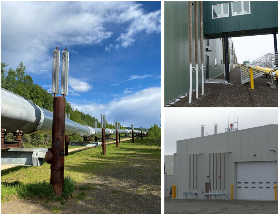
Figure 5-7. Images of thermosyphon installations. Left: on the Trans-Alaska Pipeline near Fairbanks, Alaska. Upper and lower right: along foundation edges of structures in Prudhoe Bay, Alaska. Images by T. Douglas, CRREL.
