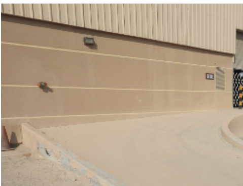
LRS Loading Ramp
