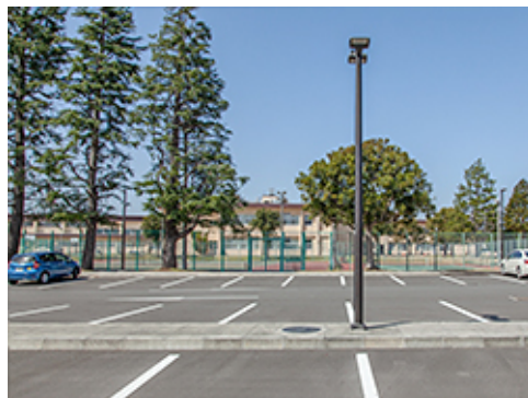
Parking Lot Lighting
