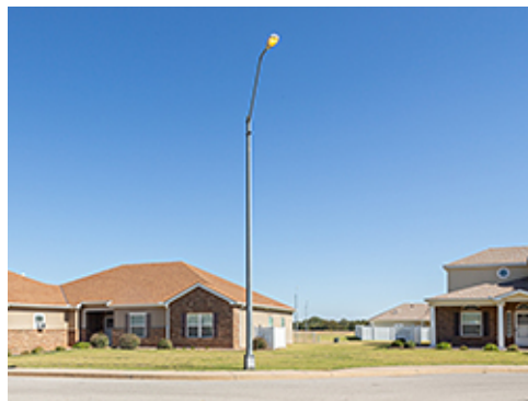
Street Light Fixture at Group 4
