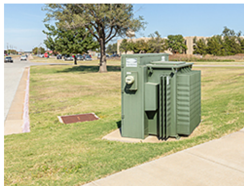
Electrical Cabinet and Equipment
