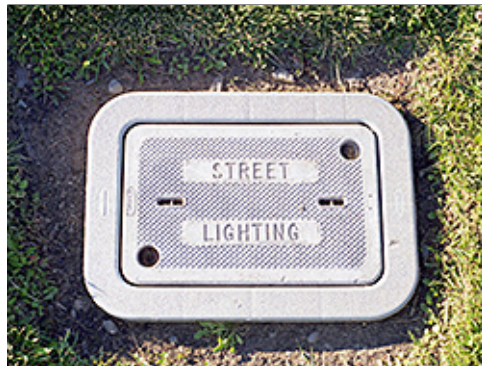
At-Grade Service Box
