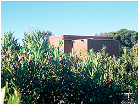
Electrical Gear Cabinets with Screening
