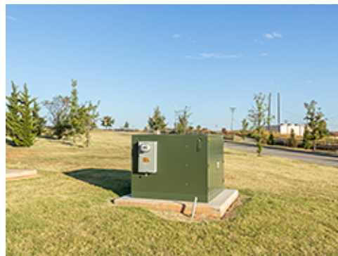
Green Cabinet in Grass Area
