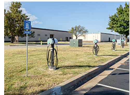
EV Charging Stations
