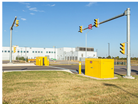
Emergency Control Equipment
