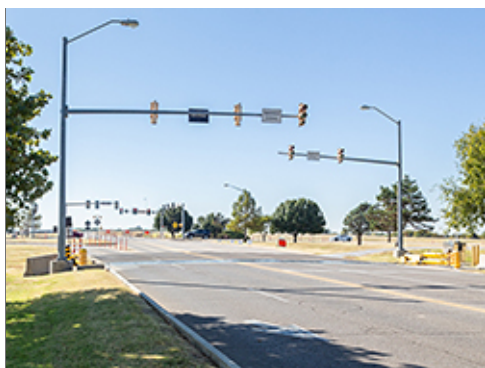
Pole with Traffic Signal Mounting
