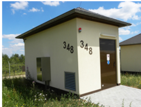
Generator (Emergency Power System)
