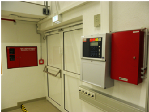
Fire Alarm System
