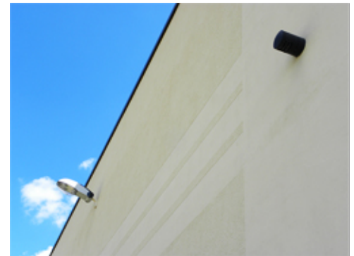
Wall Mounted Lighting
