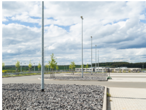
Parking Lot Lighting
