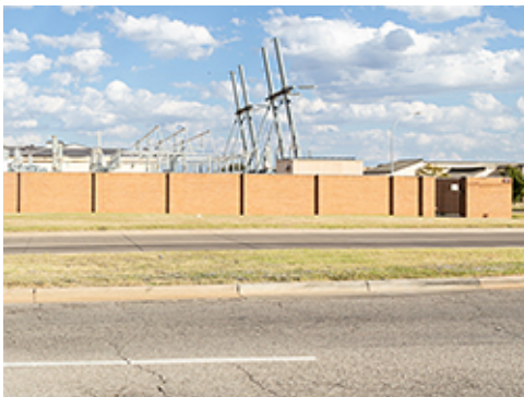
Power Substation with Masonry Screen Wall
