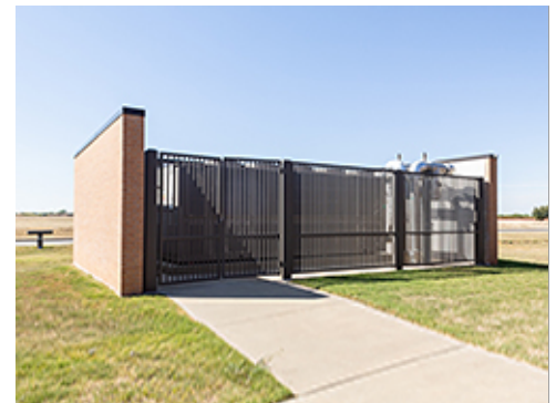
Utility Equipment Screen Wall and Gates
