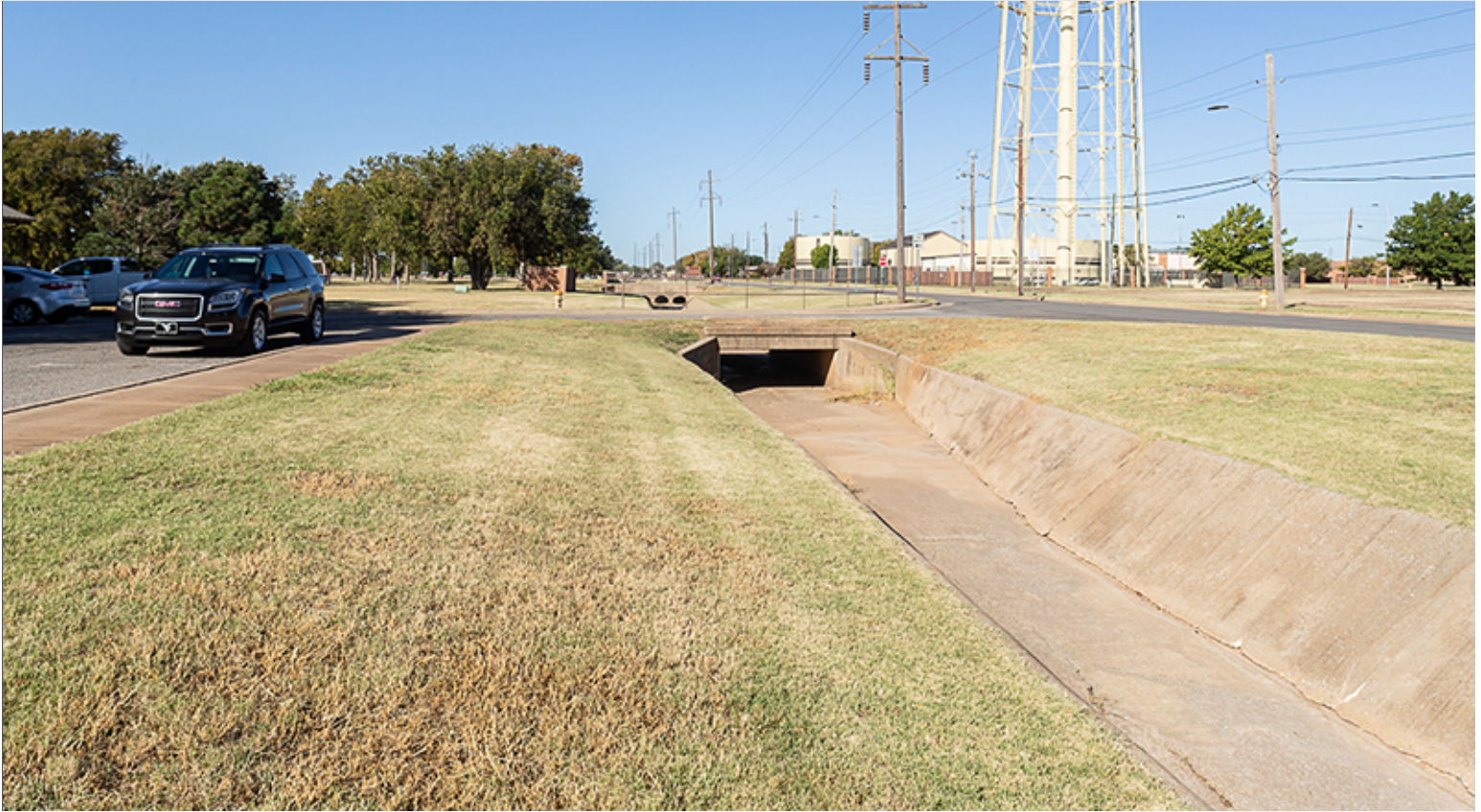
Channel Element of Base-wide Stormwater System
