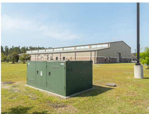
Equipment on Concrete Pad
