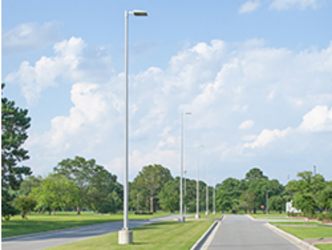
Street Lighting at Group 1
