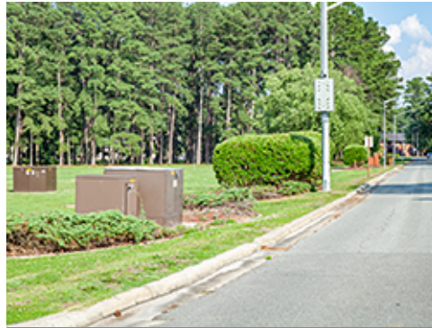
Consolidated Utility Cabinets
