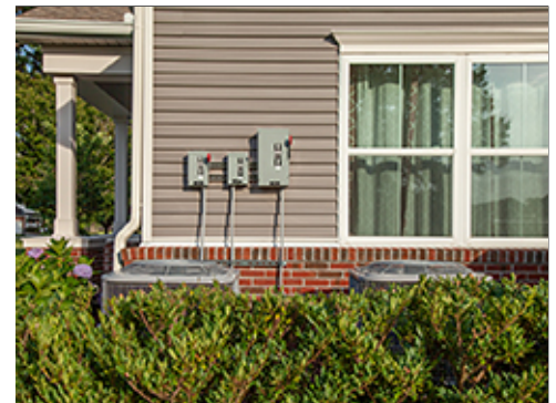
Landscape Screening of Mechanical Elements
