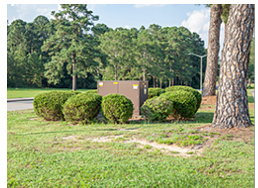
Buried Electric Service and Cabinet
