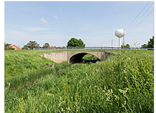
Base-wide Stormwater System
