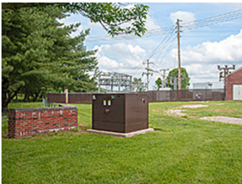
Utility Cabinet with Screen Wall
