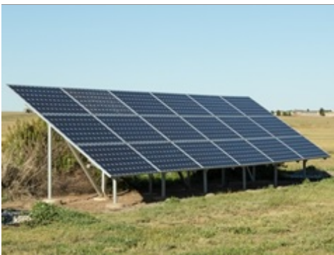
CDC Solar Photovoltaic Array
