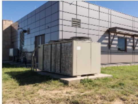
Exposed HVAC Unit
