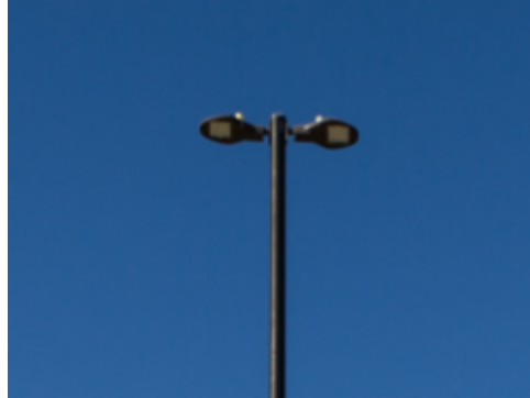
Parking Lot Lighting
